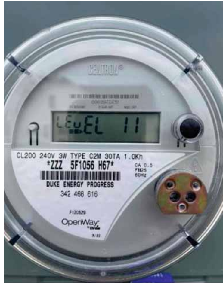
UTILITY COMPANY: Duke Energy NC
