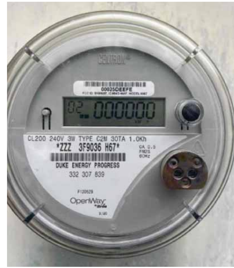
UTILITY COMPANY: Duke Energy NC
