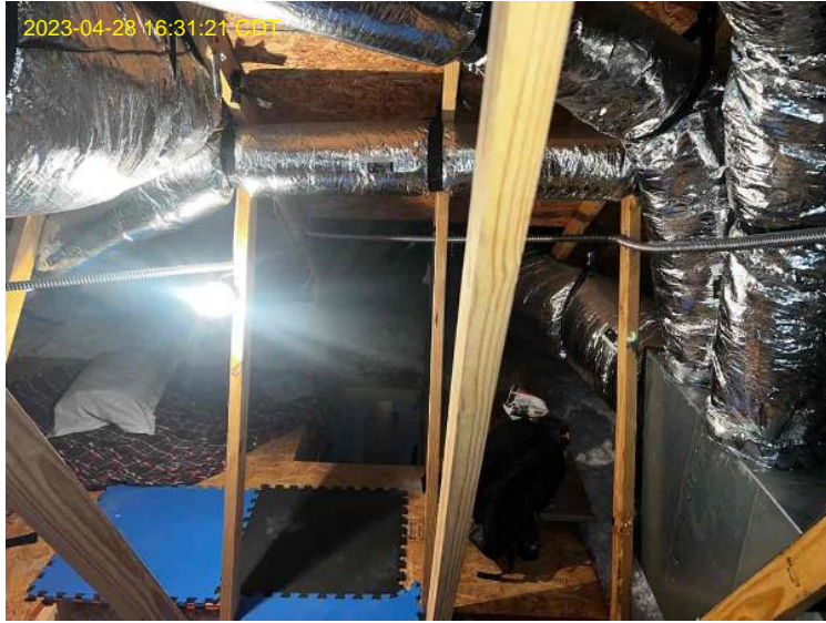
Roof/Array Work / Photo: Conduit Run(s)
