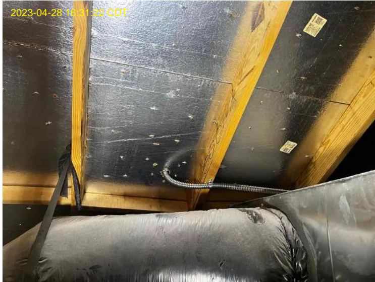
Roof/Array Work / Photo: Conduit Run(s)
