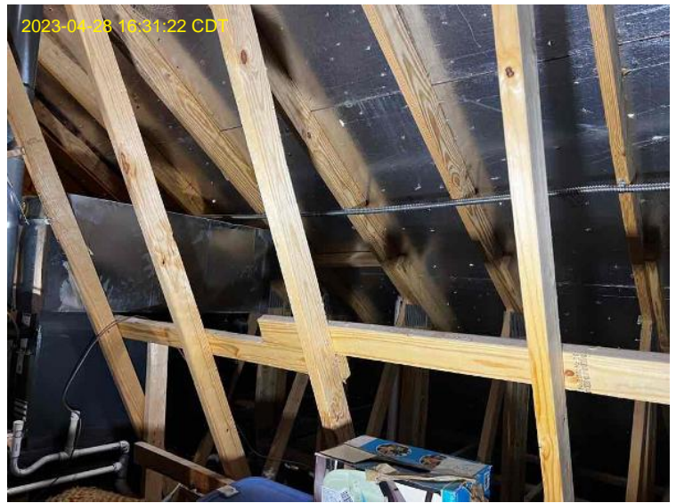
Roof/Array Work / Photo: Conduit Run(s)
