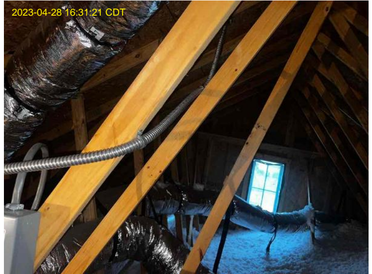
Roof/Array Work / Photo: Conduit Run(s)
