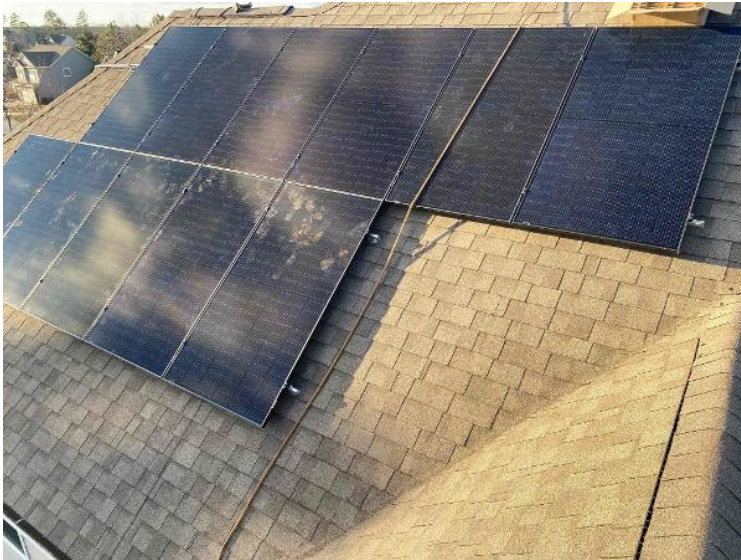
Roof / Completed Array(s) showing COMPLETE overview of arrays multiple pics and location of rooftop junction box (3 pics per array min.) (no close up pics)
