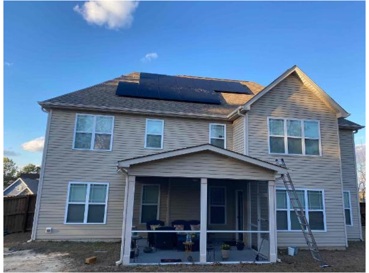
Roof / Completed Array(s) showing COMPLETE overview of arrays multiple pics and location of rooftop junction box (3 pics per array min.) (no close up pics)
