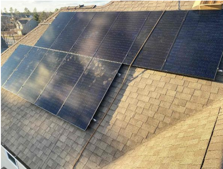
Roof / Completed Array(s) showing COMPLETE overview of arrays multiple pics and location of rooftop junction box (3 pics per array min.) (no close up pics)
