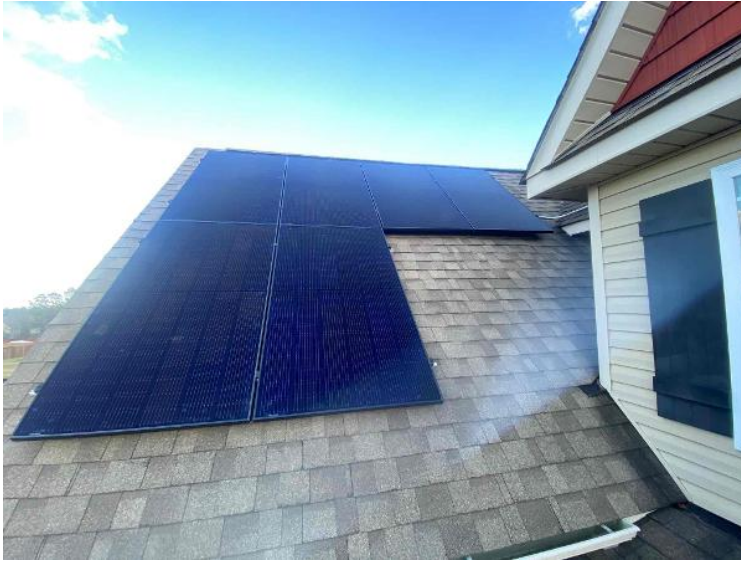
Roof / Completed Array(s) showing COMPLETE overview of arrays multiple pics and location of rooftop junction box (3 pics per array min.) (no close up pics)
