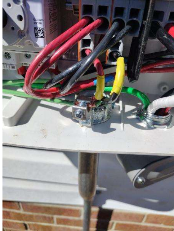
Electrical / PV Equipment - all PV equipment installed and completed, wiring, EGC (Solar Ground), entries/exits, open & closed boxes, completed overview.
