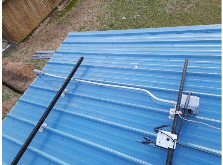
PV Arrays / Roof conduit photos- Entire conduit run to be shown along with proper supports and spacing off the roof.
