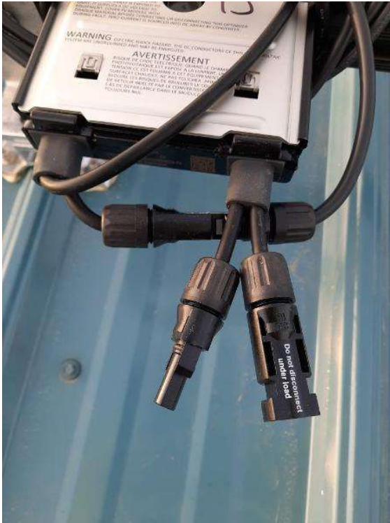
PV Arrays / Are there any wire splices in the array?
