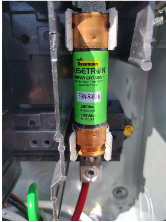
Electrical / AC Disconnect - Photos of fuse sizes and wire sizes
