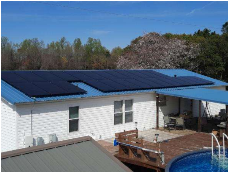
PV Arrays / Completed Array(s) showing COMPLETE overview of arrays with clean panels (No smears, handprints etc..) 3 pics per array from different angles showing each ENTIRE array.
