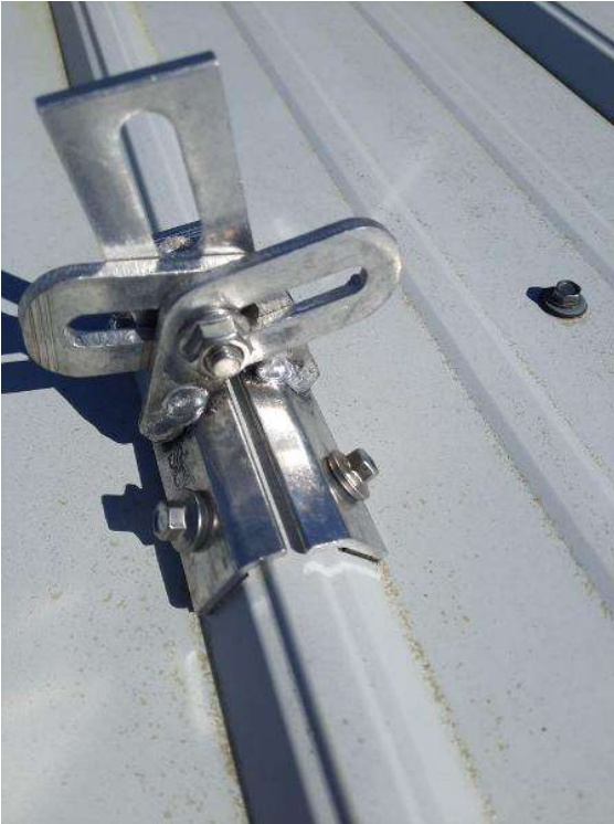
PV Arrays / Mount Installation - Need to show the correct sealing technique for at least one solar mount.
