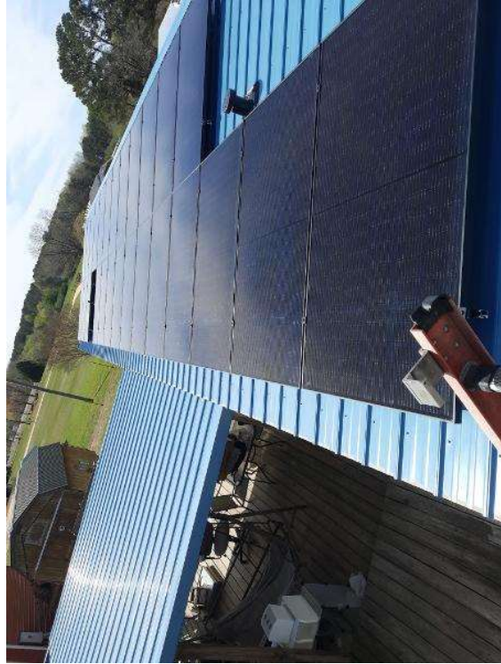
PV Arrays / Please provide pictures of the level and clean array(s) using various angles. Take at least 3.
