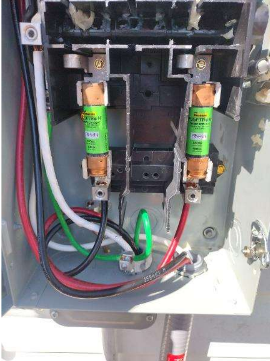
Electrical / PV Equipment - all PV equipment installed and completed, wiring, EGC (Solar Ground), entries/exits, open & closed boxes, completed overview.
