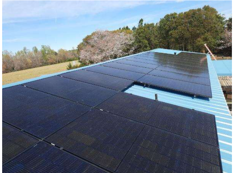
PV Arrays / Completed Array(s) showing COMPLETE overview of arrays with clean panels (No smears, handprints etc..) 3 pics per array from different angles showing each ENTIRE array.
