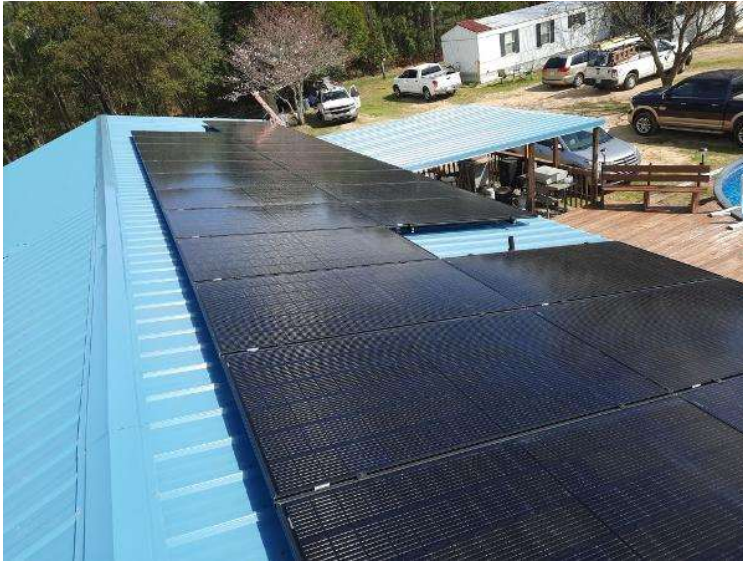
PV Arrays / Completed Array(s) showing COMPLETE overview of arrays with clean panels (No smears, handprints etc..) 3 pics per array from different angles showing each ENTIRE array.
