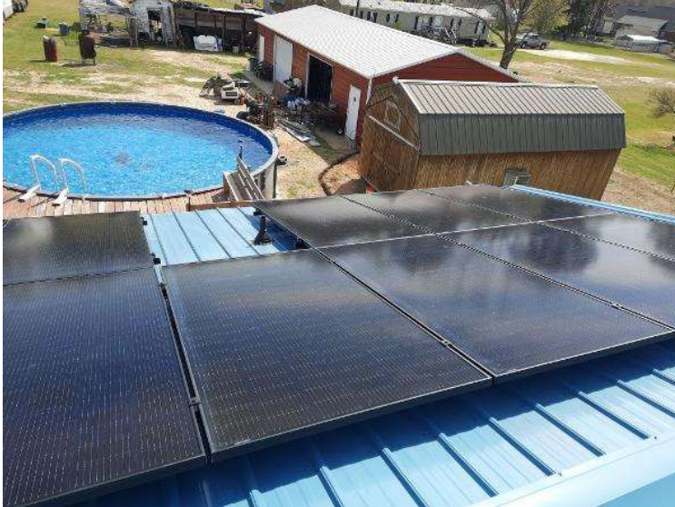
PV Arrays / Please provide pictures of the level and clean array(s) using various angles. Take at least 3.
