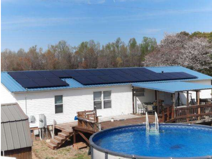
PV Arrays / Please provide pictures of the level and clean array(s) using various angles. Take at least 3.
