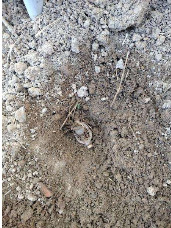
Electrical / GEC (Grounding Electrode Conductor) - Main GEC (photo of the home's grounding system)
