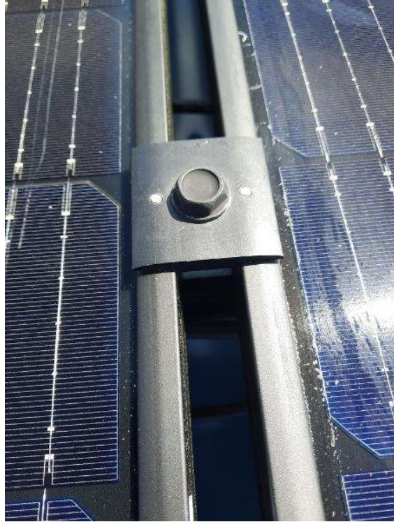
PV Arrays / Module Attachments - need to show modules are properly secured to racking.
