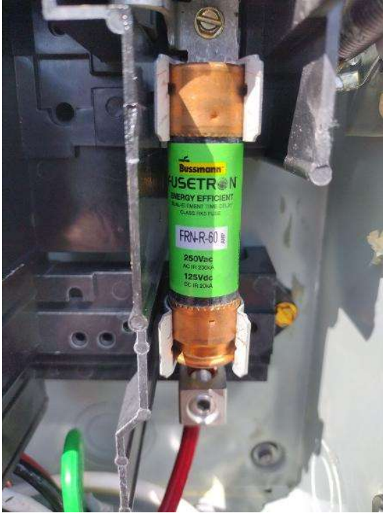
Electrical / PV Equipment - all PV equipment installed and completed, wiring, EGC (Solar Ground), entries/exits, open & closed boxes, completed overview.
