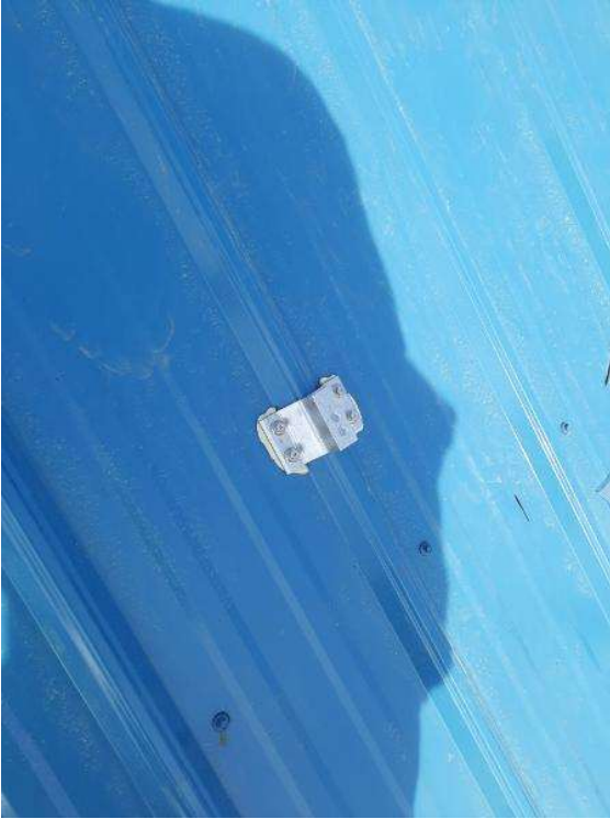
PV Arrays / Mount Installation - Need to show the correct sealing technique for at least one solar mount.
