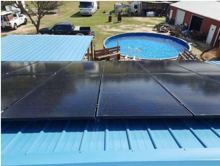
PV Arrays / Completed Array(s) showing COMPLETE overview of arrays with clean panels (No smears, handprints etc..) 3 pics per array from different angles showing each ENTIRE array.
