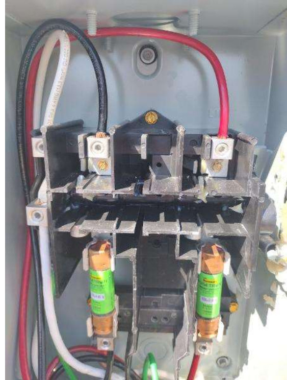
Electrical / PV Equipment - all PV equipment installed and completed, wiring, EGC (Solar Ground), entries/exits, open & closed boxes, completed overview.
