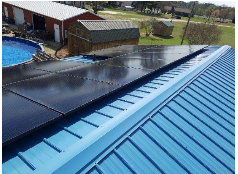
PV Arrays / Completed Array(s) showing COMPLETE overview of arrays with clean panels (No smears, handprints etc..) 3 pics per array from different angles showing each ENTIRE array.
