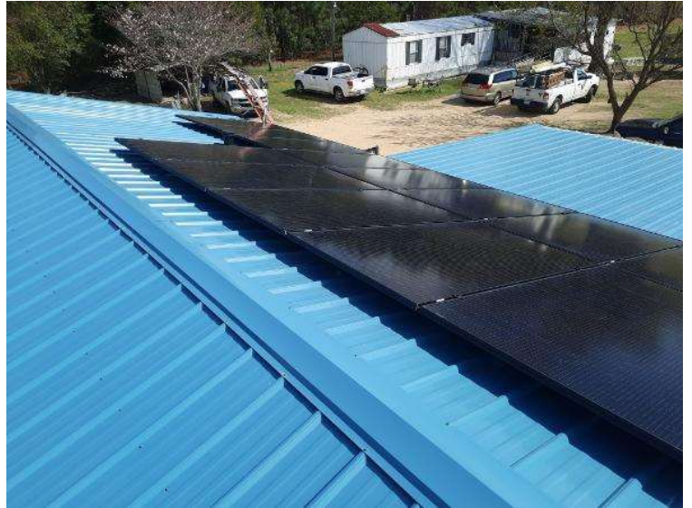
PV Arrays / Completed Array(s) showing COMPLETE overview of arrays with clean panels (No smears, handprints etc..) 3 pics per array from different angles showing each ENTIRE array.
