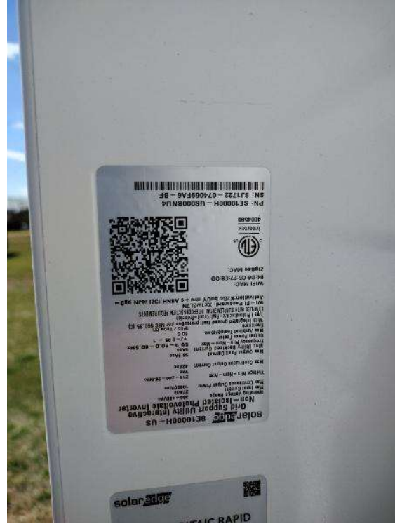
Electrical / Serial Numbers - clear photos of combiner/inverter and communication device serial numbers
