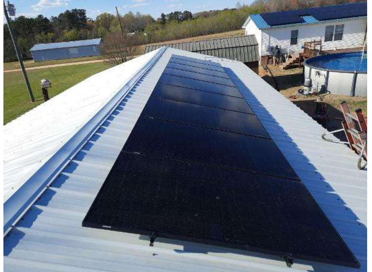
PV Arrays / Please provide pictures of the level and clean array(s) using various angles. Take at least 3.
