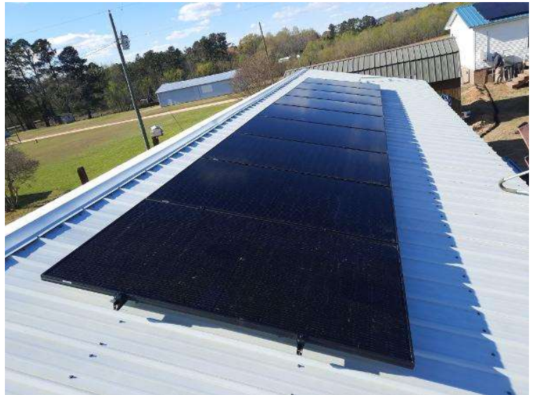
PV Arrays / Completed Array(s) showing COMPLETE overview of arrays with clean panels (No smears, handprints etc..) 3 pics per array from different angles showing each ENTIRE array.
