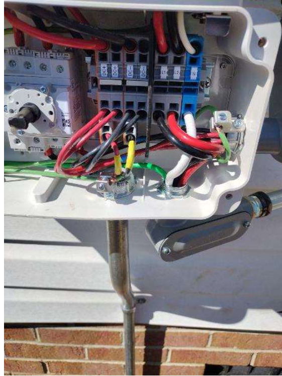
Electrical / PV Equipment - all PV equipment installed and completed, wiring, EGC (Solar Ground), entries/exits, open & closed boxes, completed overview.
