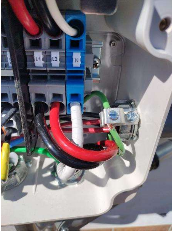
Electrical / PV Equipment - all PV equipment installed and completed, wiring, EGC (Solar Ground), entries/exits, open & closed boxes, completed overview.
