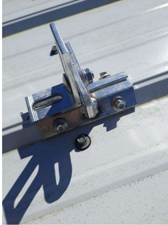
PV Arrays / Mount Installation - Need to show the correct sealing technique for at least one solar mount.
