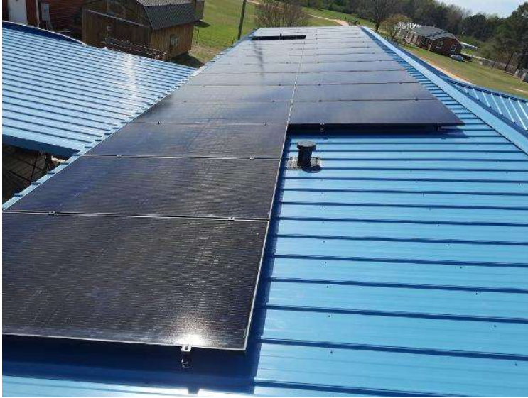
PV Arrays / Please provide pictures of the level and clean array(s) using various angles. Take at least 3.
