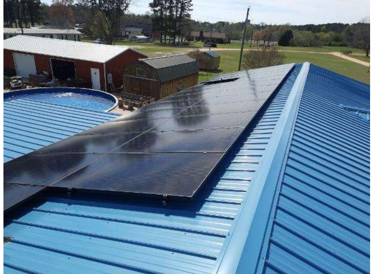
PV Arrays / Please provide pictures of the level and clean array(s) using various angles. Take at least 3.
