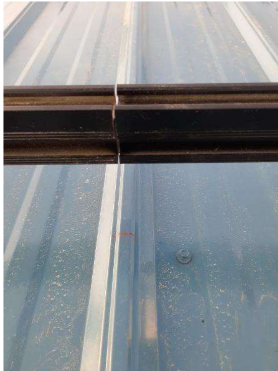
PV Arrays / Provide a photo of the front and back of ALL rail splices properly installed. Notate in the comments how many splices were used. If 0, no photos are necessary.
