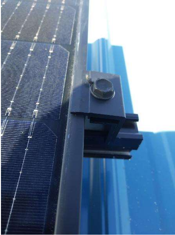
PV Arrays / Module Attachments - need to show modules are properly secured to racking.
