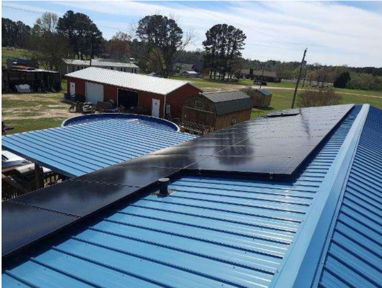
PV Arrays / Completed Array(s) showing COMPLETE overview of arrays with clean panels (No smears, handprints etc..) 3 pics per array from different angles showing each ENTIRE array.
