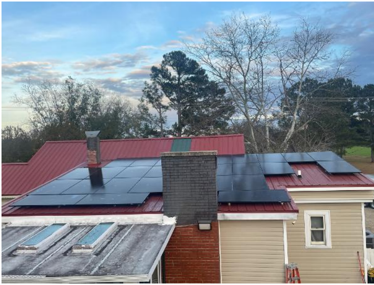
Roof / Techo / Complete Array (every module shown)
