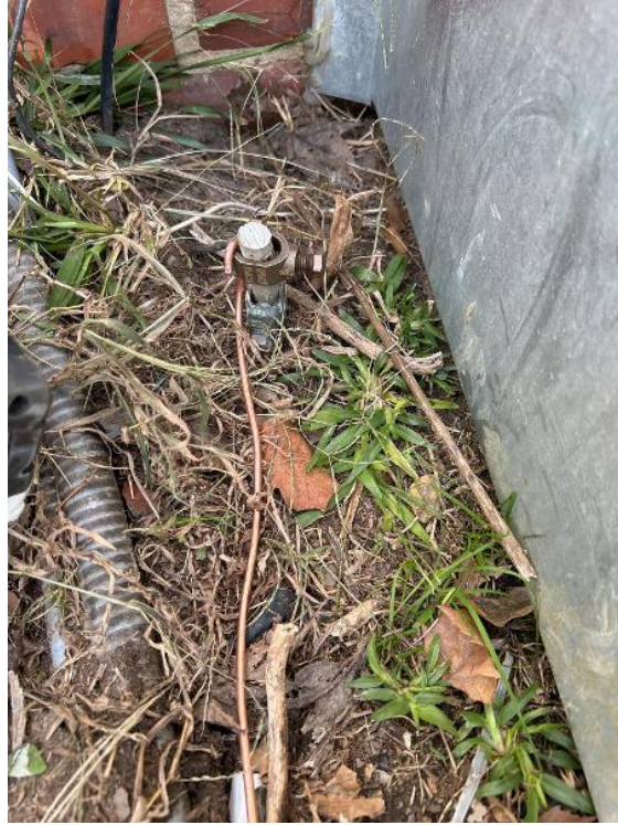
Electrical / Electrico / Visible Grounding to Electrode Show All (ground rods, water main, Ufer, other)
