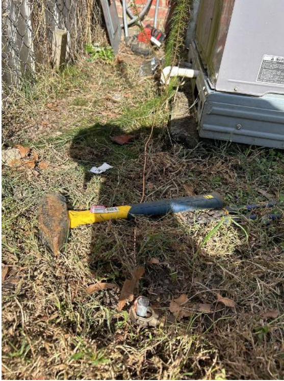
Electrical / Electrico / Visible Grounding to Electrode Show All (ground rods, water main, Ufer, other)
