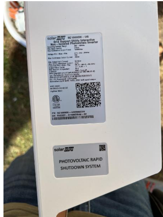
Electrical / Electrico / Inverter Serial Labels (full side label, serial QR code, & RGM)
