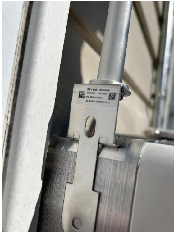
Electrical / Electrico / Inverter with Cell Kit (upper section of inverter without cover)
