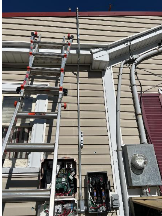
Electrical / Electrico / Attic Conduit Run
