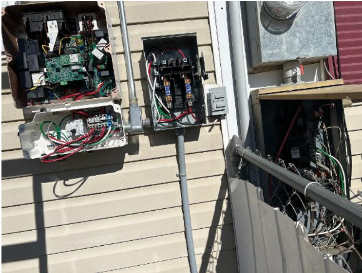
Electrical / Electrico / Interconnection Wiring Overview (pullback of meter /panel covers off)
