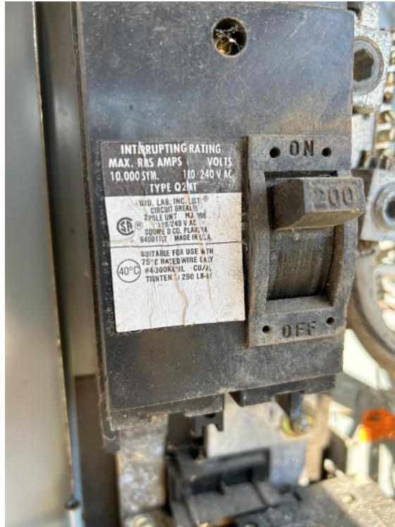
Electrical / Electrico / Interconnection (tie-in closeup, solar breaker rating, msp bus rating)
