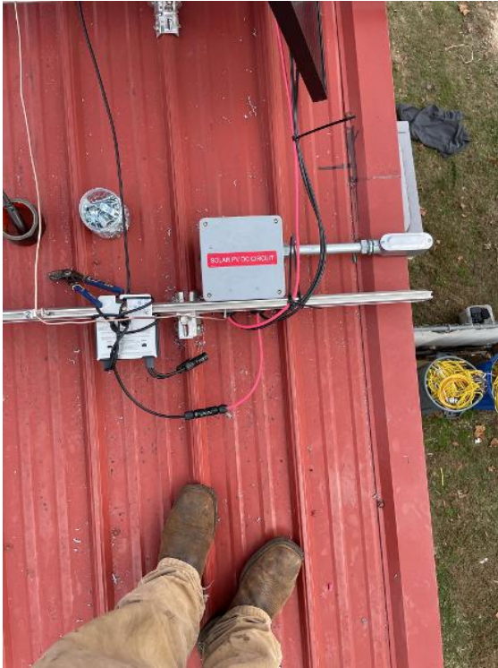
Roof / Techo / SolaDeck/Junction Box (each array cover on/off)
