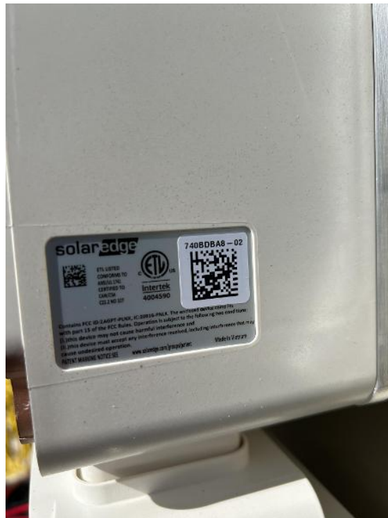
Electrical / Electrico / Inverter Serial Labels (full side label, serial QR code, & RGM)
