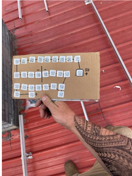
Roof / Techo / Optimizer/Microinverter Map (arranged in array layout)
