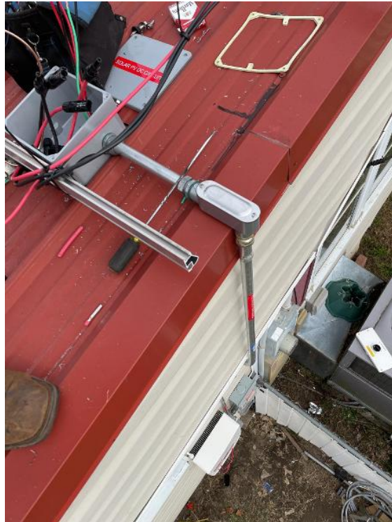
Roof / Techo / Rooftop Conduit Penetration (showing sealant under flashing and around conduit)
