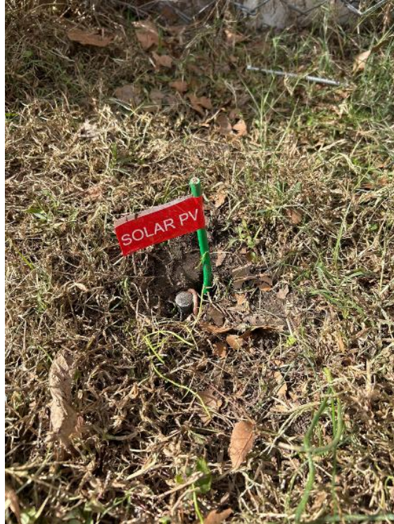
Electrical / Electrico / Visible Grounding to Electrode Show All (ground rods, water main, Ufer, other)
