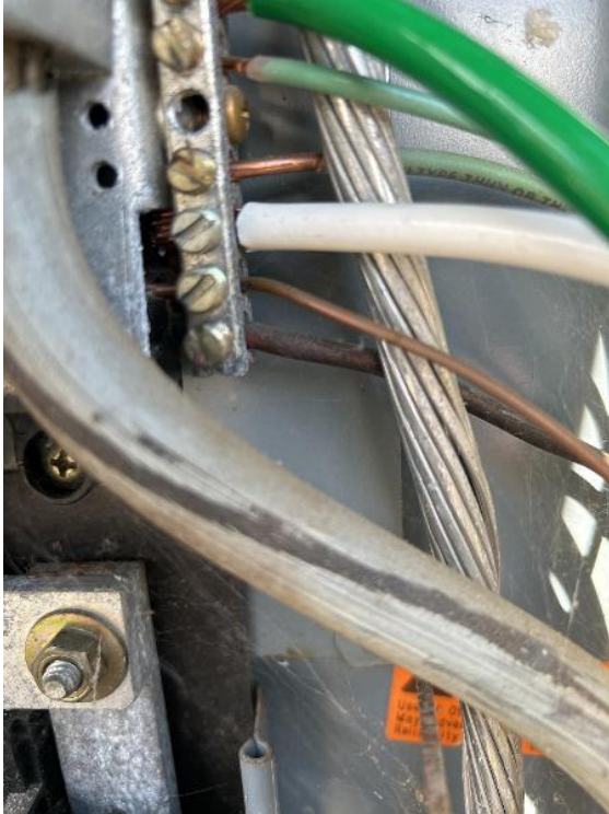
Electrical / Electrico / Visible Grounding to Electrode Show All (ground rods, water main, Ufer, other)
