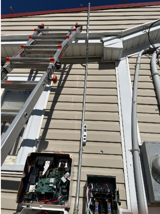
Electrical / Electrico / BOS Conduit Run (show point of entry with sealant closeup inside and out of conduit body, and drainage weep holes)
