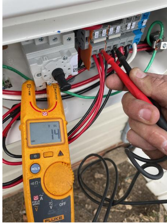
Electrical / Electrico / Voltage at Open Circuit (DCv of each string, not connected to inverter)
