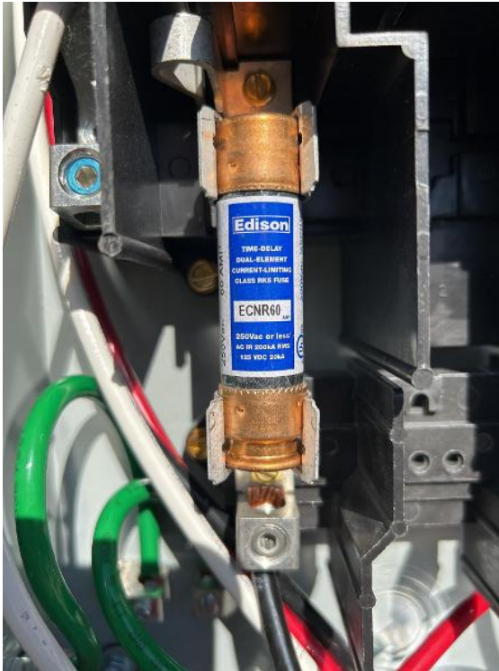
Electrical / Electrico / AC Disconnect Wiring (close up of fuse rating when needed)
