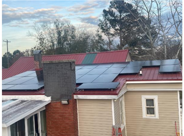
Roof / Techo / Complete Array (every module shown)
