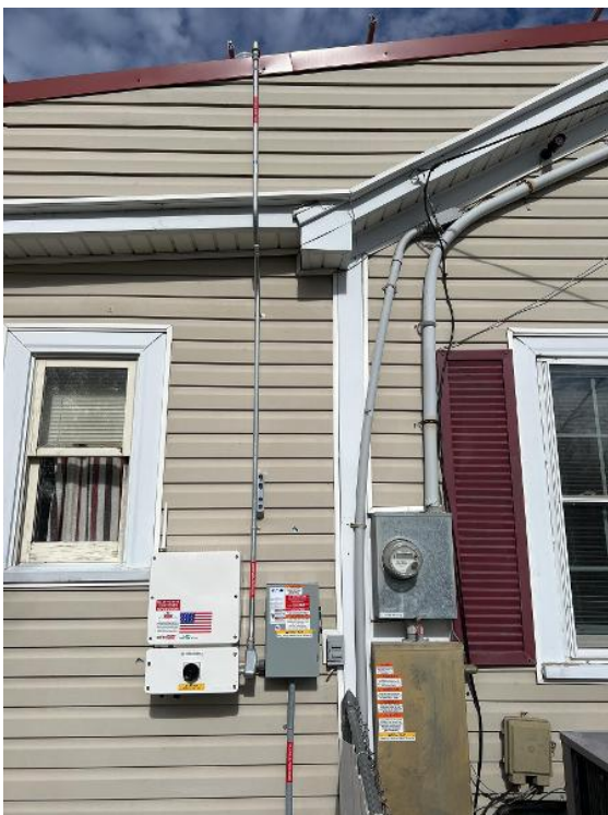
Electrical / Electrico / Electrical Equipment Overview (pullback of all boxes, discos, meters, inverter)
