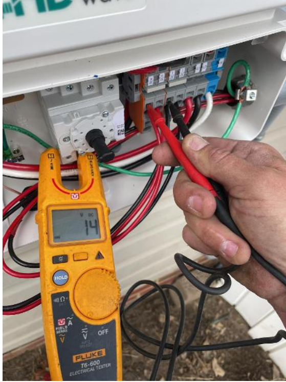
Electrical / Electrico / Voltage at Open Circuit (DCv of each string, not connected to inverter)
