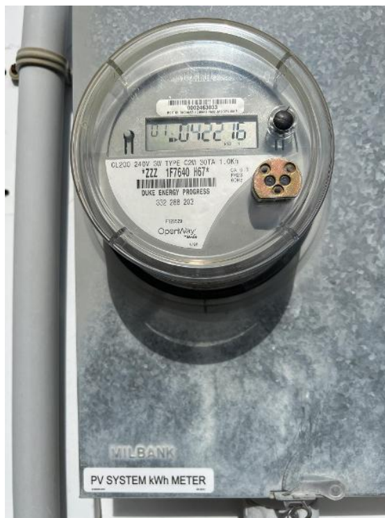
Electrical / Electrico / Utility Service Meter with Warning Label (including utility meter number closeup)
