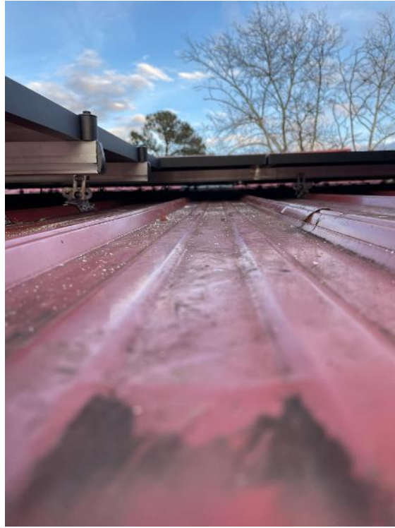
Roof / Techo / Under Array Wire Management (each array)
