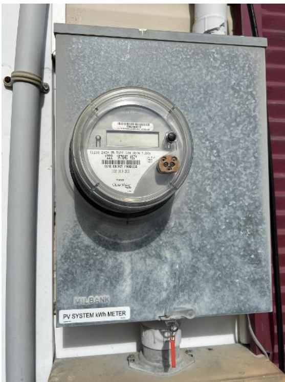
Electrical / Electrico / BOS Stickers for Each Box (covers on)
