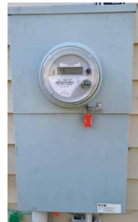
UTILITY COMPANY: Duke Energy NC
