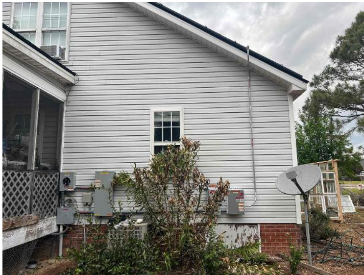
Electrical / MSP (Main Service Panel) - Photo of Entire Box After Interconnection
