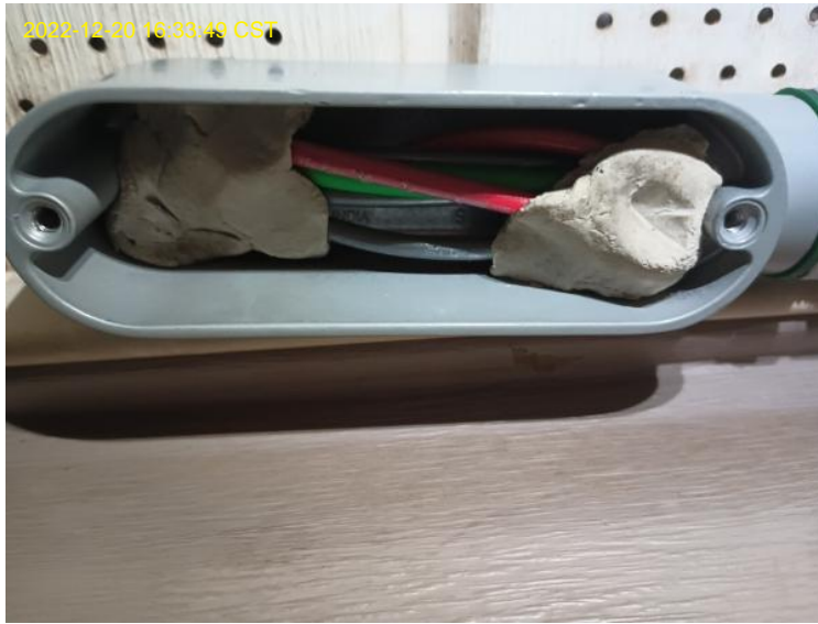
Roof/Array Work / Photo: Conduit Run(s)
