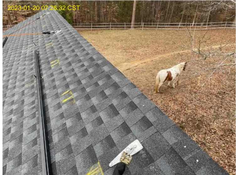
Safety / Photo: Fall Protection Anchor
