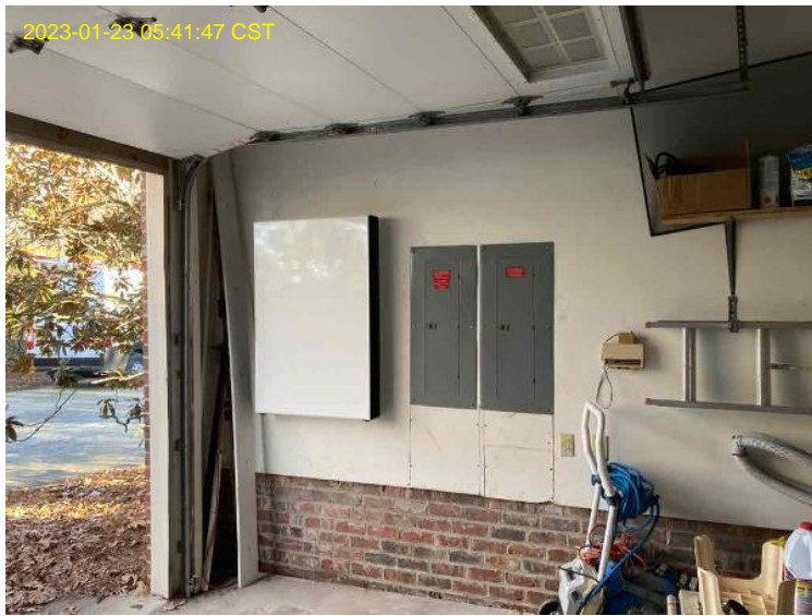
Electrical Information / Photo: EQ Wall Wide Shot
