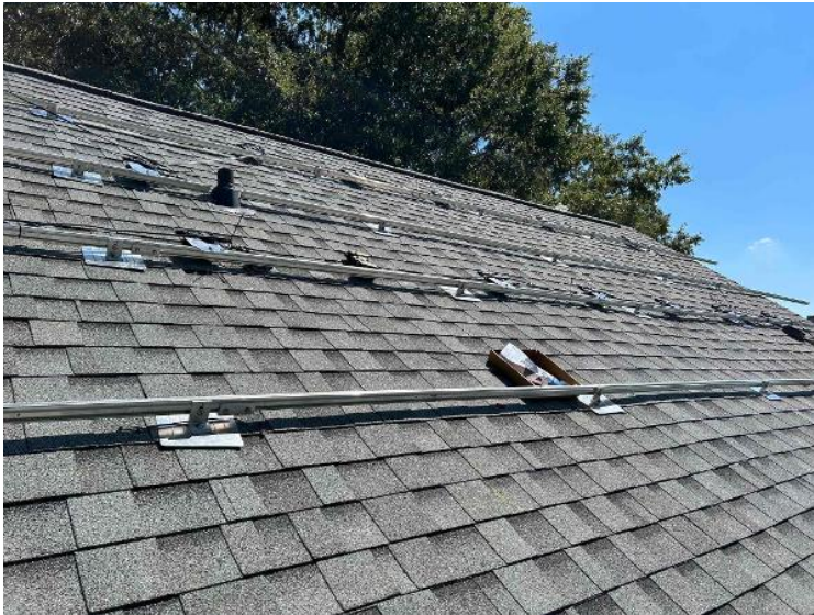
Roof / Attachment Layout - showing COMPLETE layouts, staggered attachments, span measurement. (2 pics per array min)
