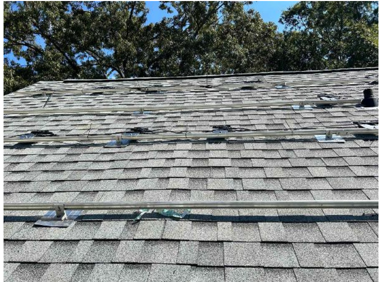
Roof / Attachment Layout - showing COMPLETE layouts, staggered attachments, span measurement. (2 pics per array min)
