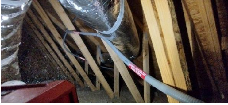
Electrical / Path To Array Roof/Attic - conduit run, j-box inside and out, sealed penetration, etc.,
