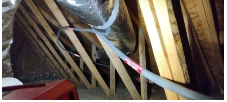
Electrical / Path To Array Roof/Attic - conduit run, j-box inside and out, sealed penetration, etc.,
