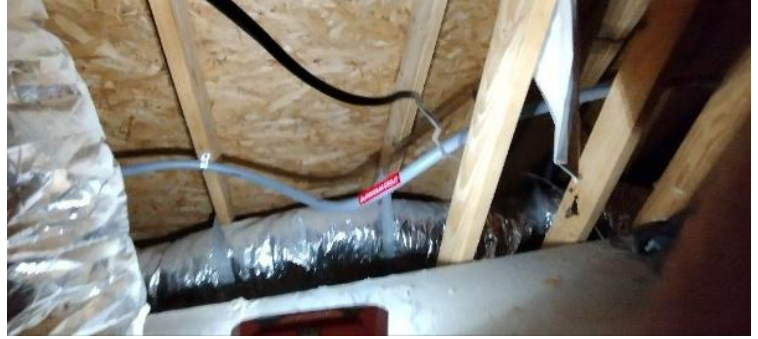
Electrical / Path To Array Roof/Attic - conduit run, j-box inside and out, sealed penetration, etc.,
