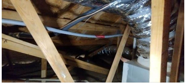
Electrical / Path To Array Roof/Attic - conduit run, j-box inside and out, sealed penetration, etc.,
