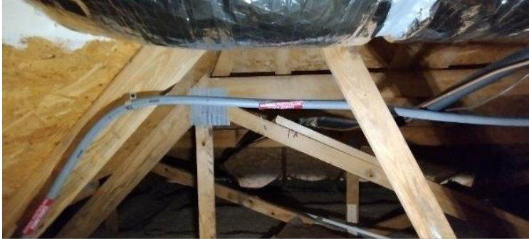
Electrical / Path To Array Roof/Attic - conduit run, j-box inside and out, sealed penetration, etc.,
