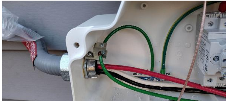
Electrical / GEC (Grounding Electrode Conductor) - main GEC (photo of the home's grounding system, MSP overview if none found)
