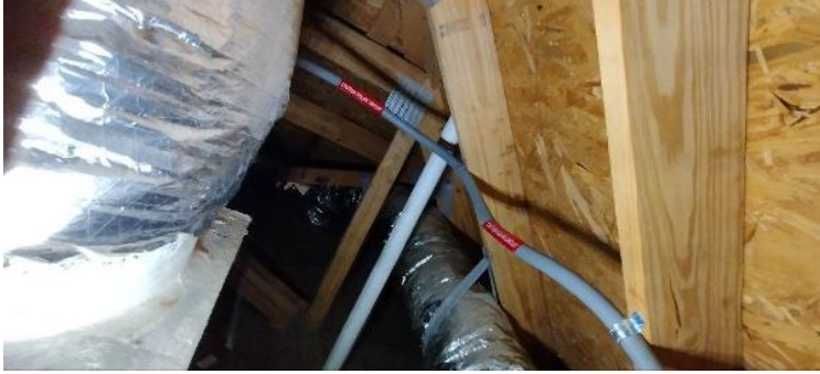
Electrical / Path To Array Roof/Attic - conduit run, j-box inside and out, sealed penetration, etc.,
