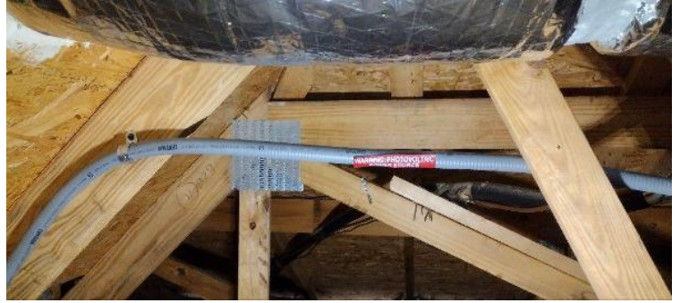
Electrical / Path To Array Roof/Attic - conduit run, j-box inside and out, sealed penetration, etc.,
