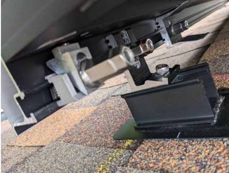
Roof / Trim Rail Grounding: 1) Take an up close photo of the trim rail bonding lug.
