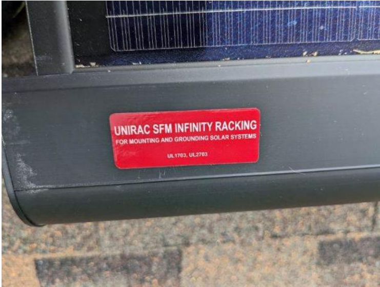
Roof / Photo of Trim Rail sticker installed
