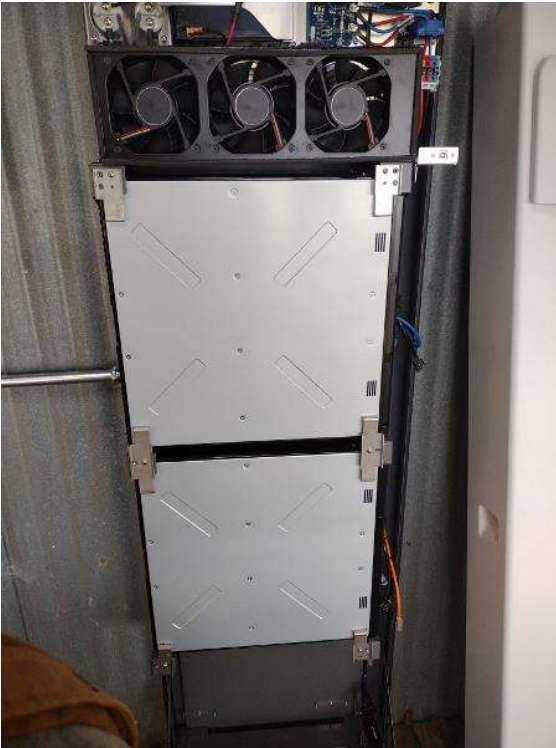
Electrical / Battery Cabinet: open and closed
