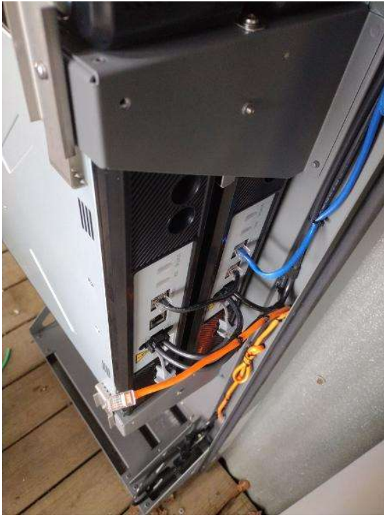
Electrical / All battery connections inside the cabinet
