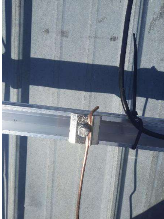
PV Arrays / Take an up close photo of EACH rail bonding lug with proper grounding wire installed.
