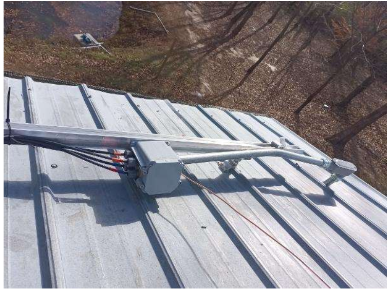
Electrical / PV Equipment - all PV equipment installed and completed, wiring, EGC (Solar Ground), entries/exits, open & closed boxes, completed overview.
