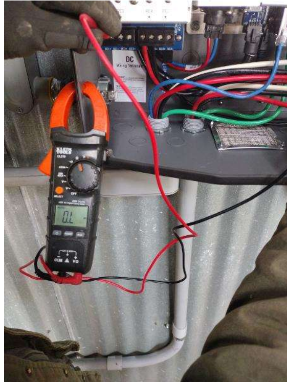
Electrical / Photo of resistance reading between Rebus and ground. You will need to use the Ohm setting on your multimeter. If you don't have meter then what are we even doing here.
