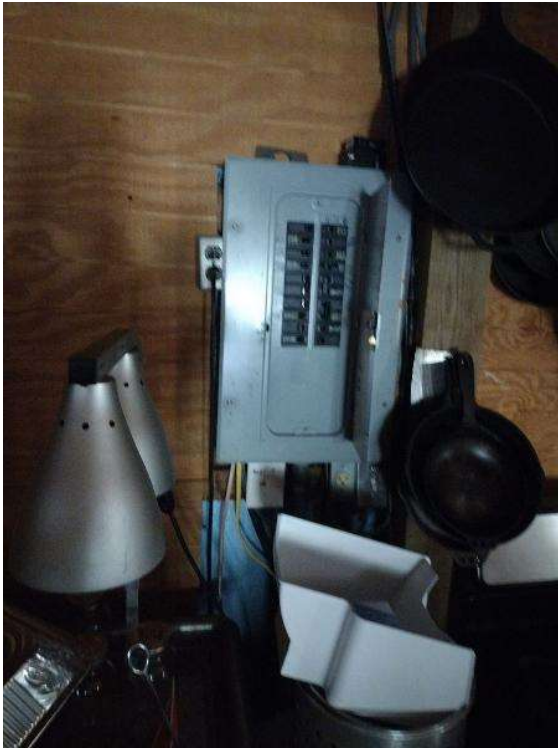
Electrical / Photo of the Protected Loads Panel
