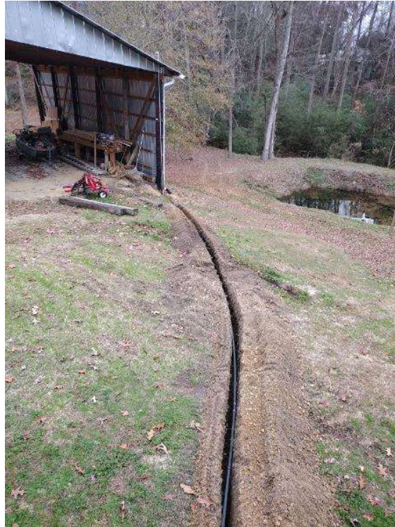
Electrical / Path To Array Roof/Attic - Conduit run, snap some shots showing the conduit is labled and secured properly.
