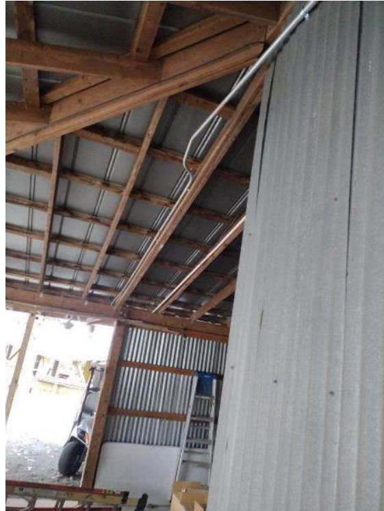
Electrical / Path To Array Roof/Attic - Conduit run, snap some shots showing the conduit is labeled and secured properly.
