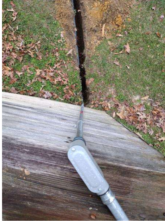
Electrical / Path To Array Roof/Attic - Conduit run, snap some shots showing the conduit is labled and secured properly.
