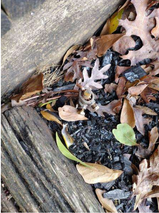
Electrical / Photo of the the GEC you installed and some clear shots of the acorns and clear shots of the pathway from our EGC to the existing EGC.
