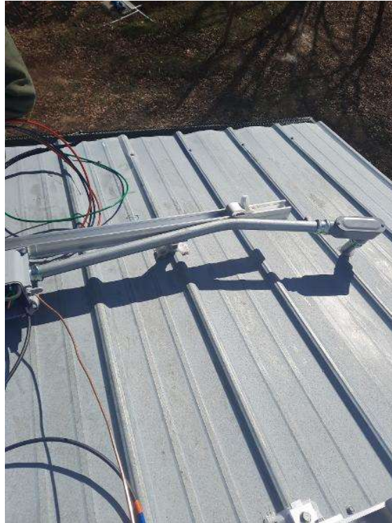
PV Arrays / Roof conduit photos- Entire conduit run to be shown along with proper supports.
