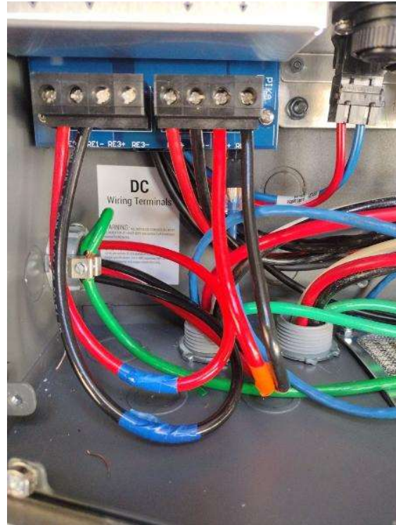
Electrical / Rebus DC terminals
