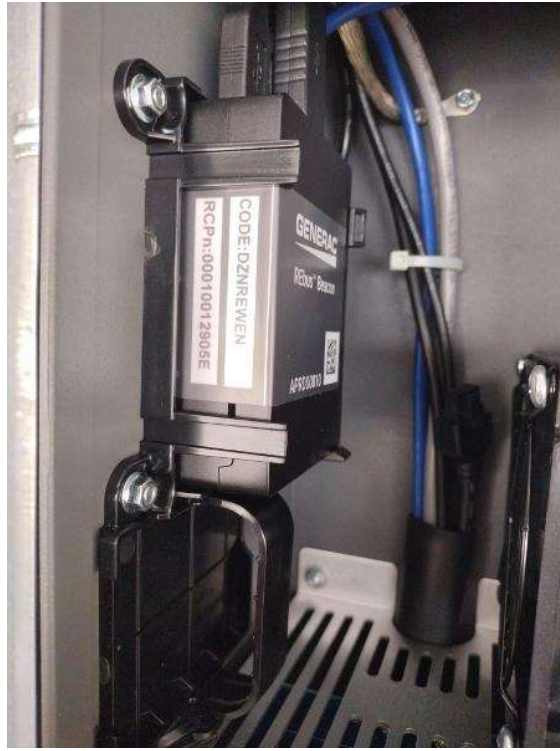
Electrical / Beacon and Cell Modem properly installed
