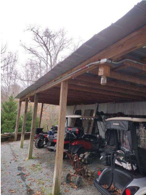
Electrical / Path To Array Roof/Attic - Conduit run, snap some shots showing the conduit is labled and secured properly.
