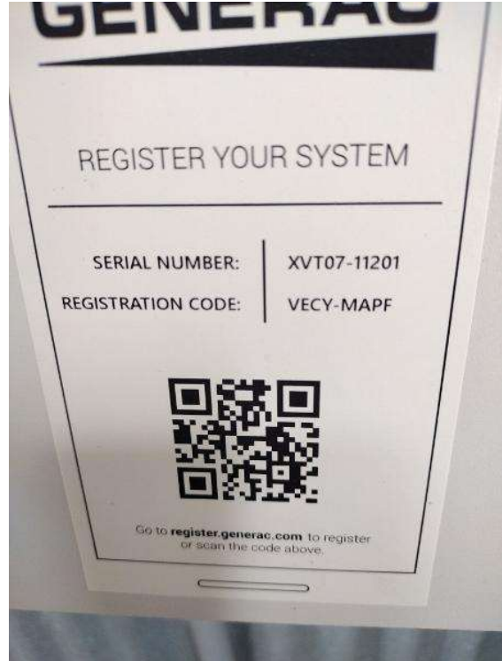
Electrical / PWRCell serial number for each PWRCell installed
