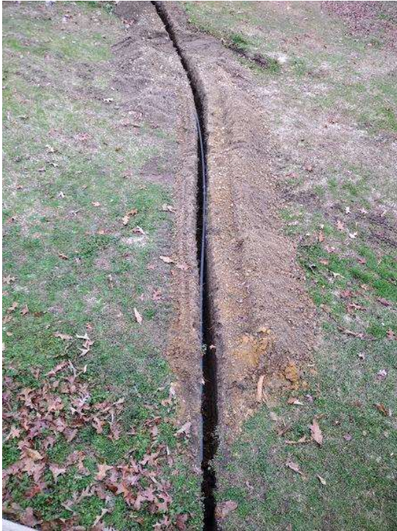
Electrical / Path To Array Roof/Attic - Conduit run, snap some shots showing the conduit is labled and secured properly.
