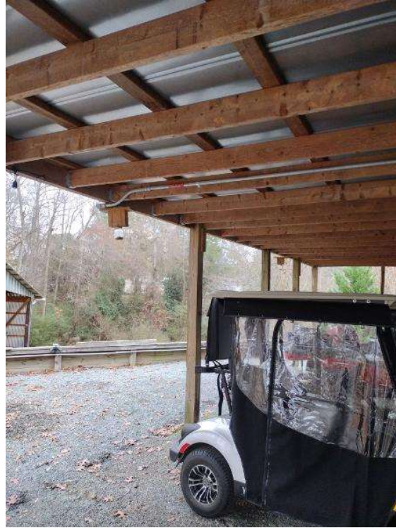
Electrical / Path To Array Roof/Attic - Conduit run, snap some shots showing the conduit is labled and secured properly.
