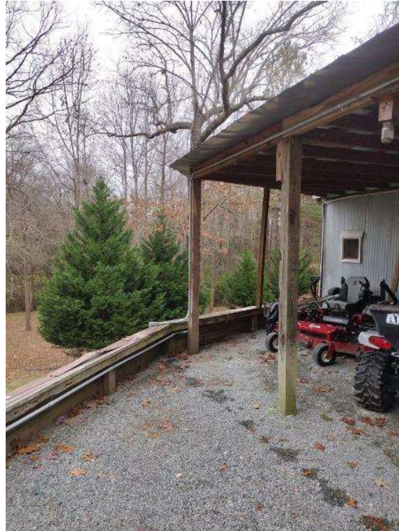
Electrical / Path To Array Roof/Attic - Conduit run, snap some shots showing the conduit is labled and secured properly.
