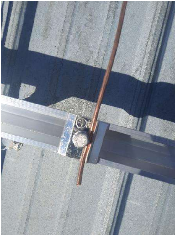
PV Arrays / Take an up close photo of EACH rail bonding lug with proper grounding wire installed.
