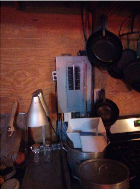
Electrical / Protected loads panel with all wires landed
