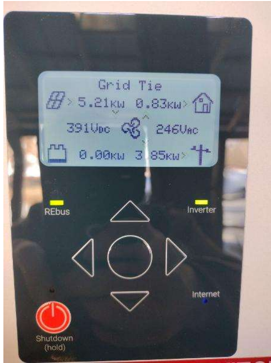
Electrical / Screen photos showing the proper mode selected
