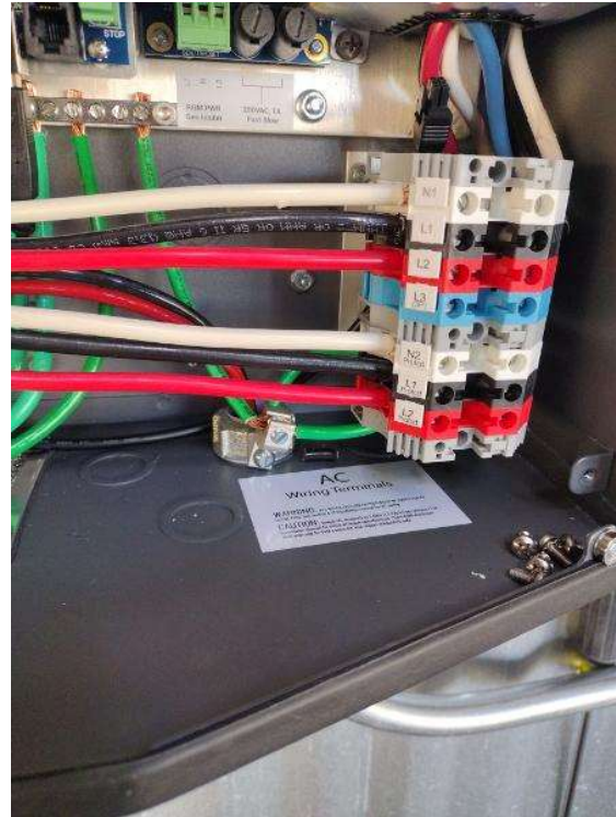
Electrical / Installed PWRCell Inverter (open showing full inverter plus all terminations)
