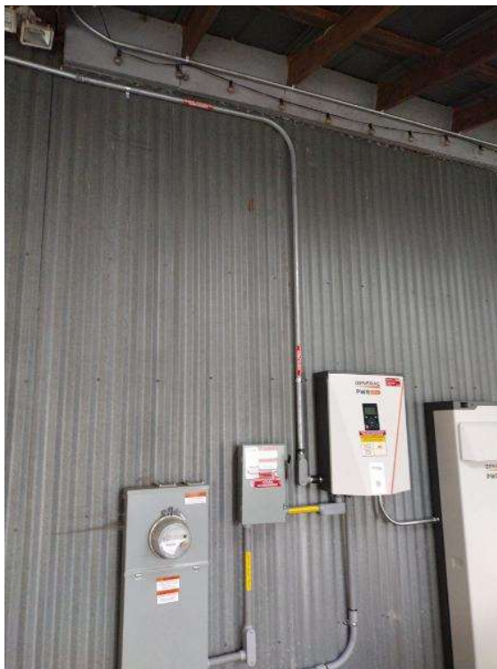
Electrical / Provide enough photos to show all wire/conduit runs through the structure. The photos must show the entirety of all wire/conduit that was installed. It must show that the proper labeling and straps/staples have been applied.
