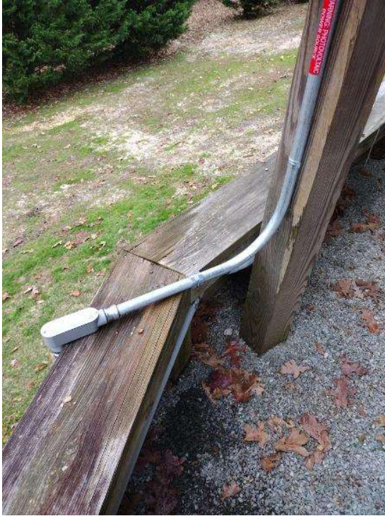
Electrical / Path To Array Roof/Attic - Conduit run, snap some shots showing the conduit is labled and secured properly.
