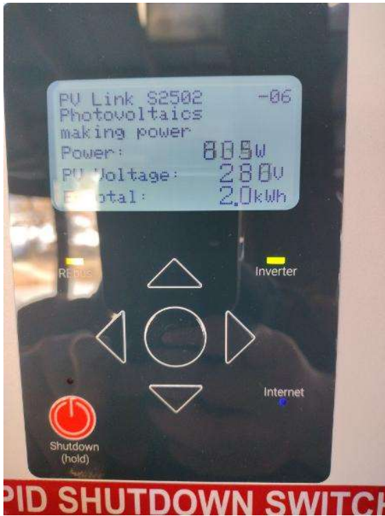
Electrical / Each PV LINK installed and the serial that correspond to the equipment on the inverter screen.
