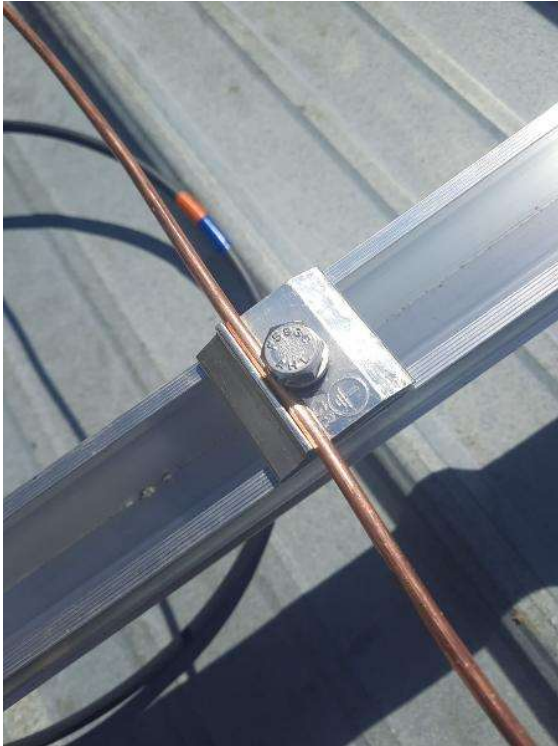
PV Arrays / Take an up close photo of EACH rail bonding lug with proper grounding wire installed.
