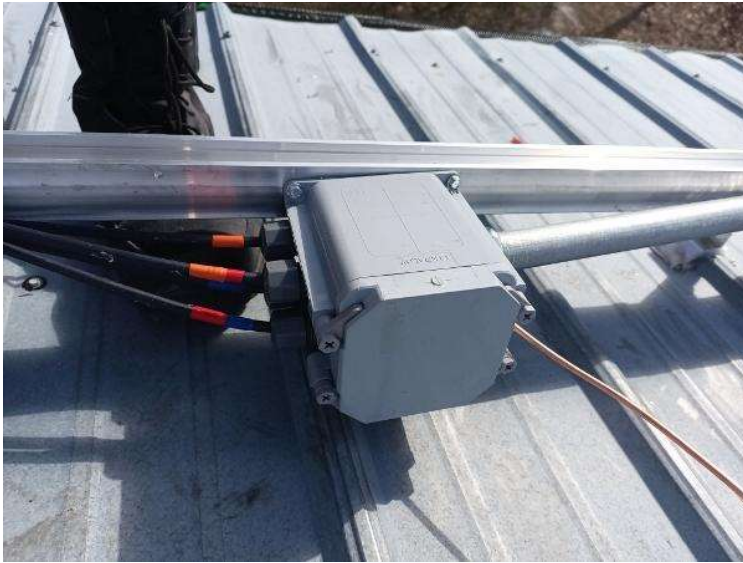
Electrical / PV Equipment - all PV equipment installed and completed, wiring, EGC (Solar Ground), entries/exits, open & closed boxes, completed overview.
