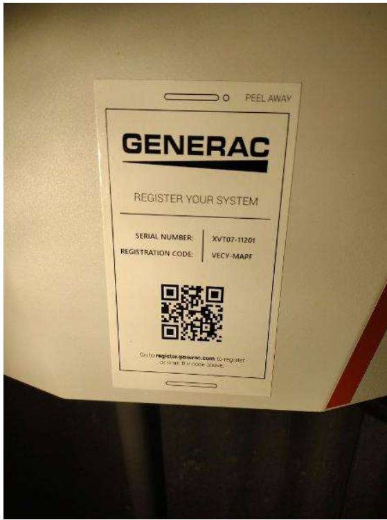
Electrical / Inverter Serial number
