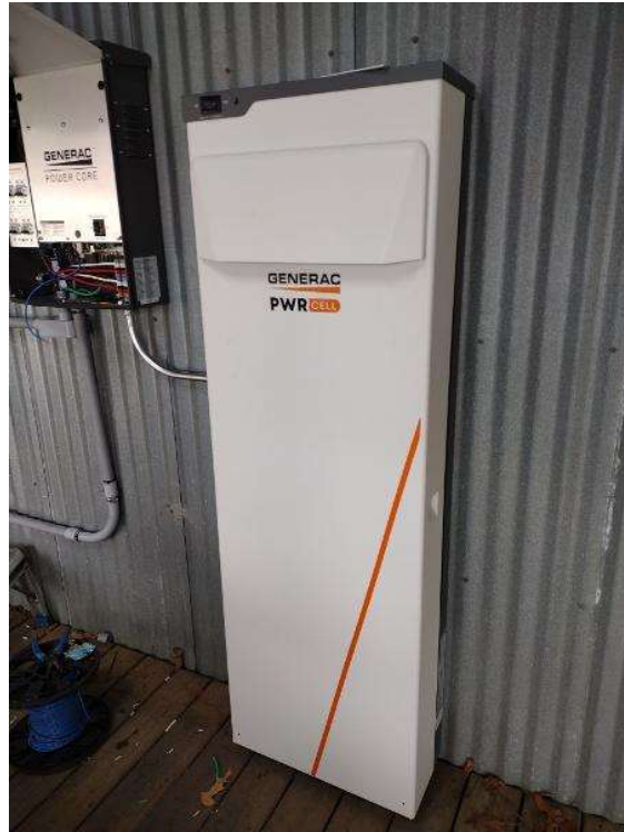
Electrical / Battery Cabinet: open and closed
