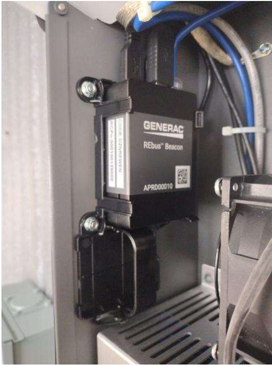
Electrical / Beacon and Cell Modem properly installed
