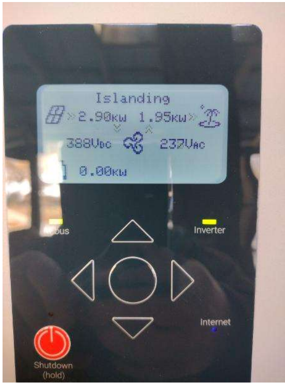
Electrical / Screen photo showing islanding is activated
