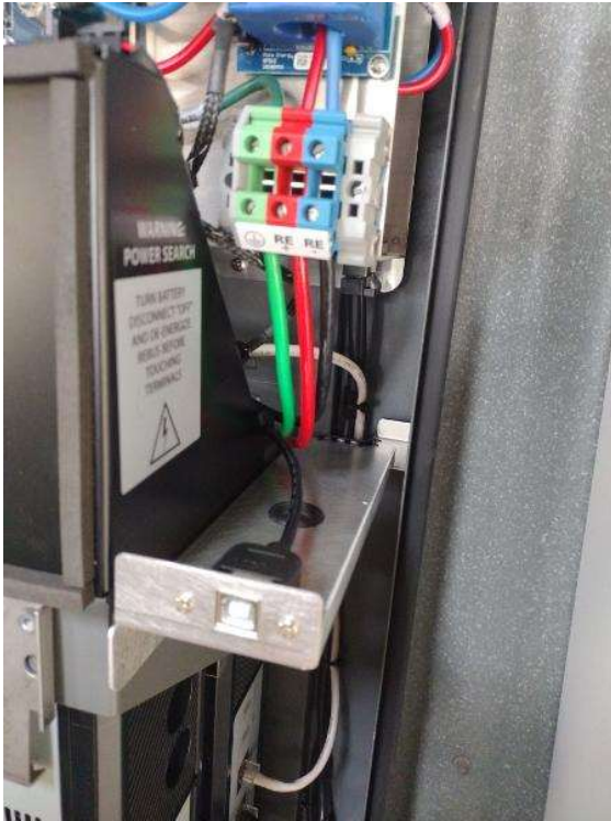
Electrical / All battery connections inside the cabinet
