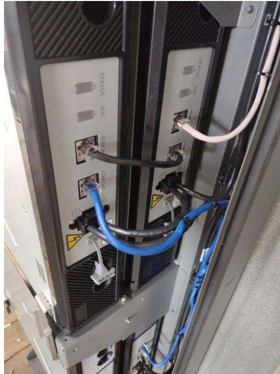
Electrical / All battery connections inside the cabinet
