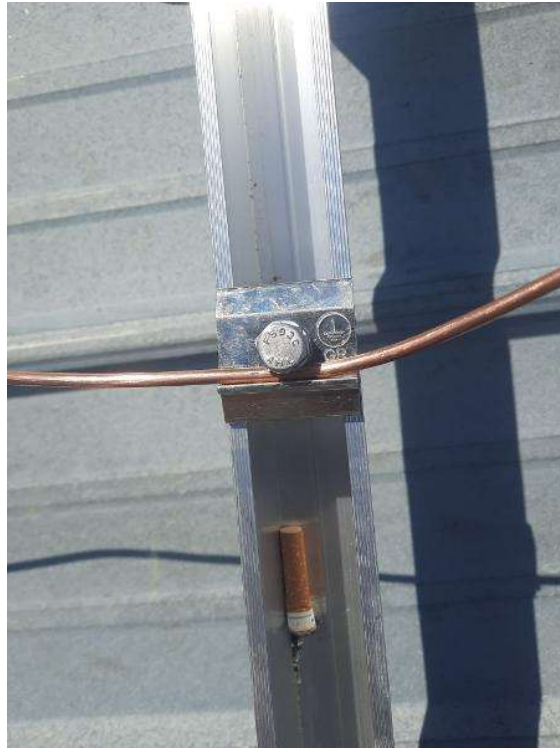
PV Arrays / Take an up close photo of EACH rail bonding lug with proper grounding wire installed.
