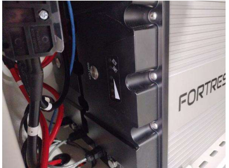
Electrical / Snap a photo of the all the dip switches in the battery bank toggled properly
