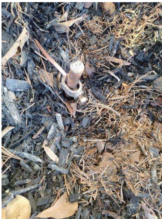
Electrical / Photo of the the GEC you installed and some clear shots of the acorns and clear shots of the pathway from our EGC to the existing EGC.
