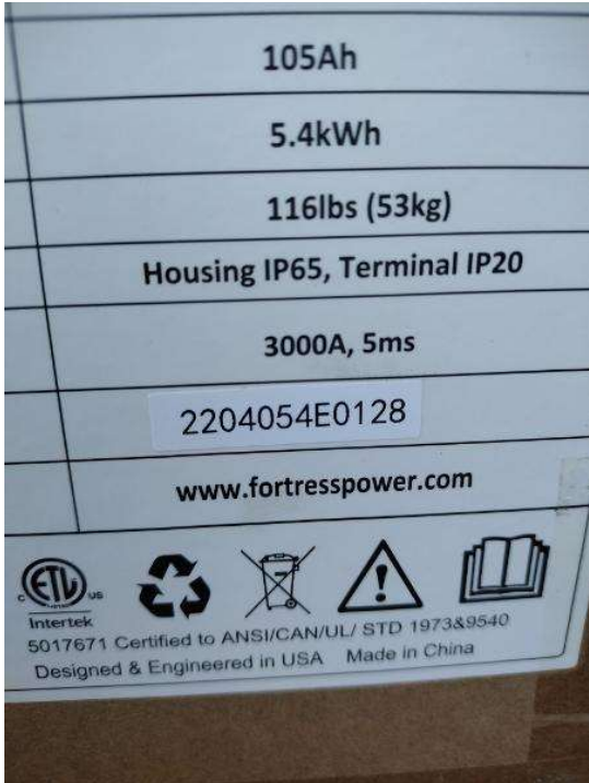
Electrical / Serial Numbers - clear photos of combiner/inverter and communication device serial numbers
