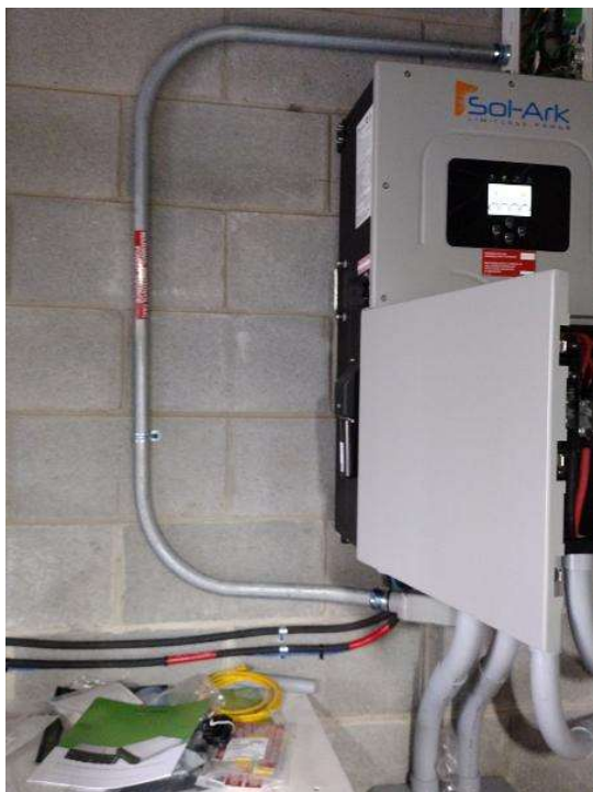
Electrical / Path To Array Roof/Attic - Conduit run, snap some shots showing the conduit is labeled and secured properly.
