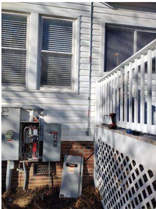
Electrical / Path To Array Roof/Attic - Conduit run, snap some shots showing the conduit is labeled and secured properly.
