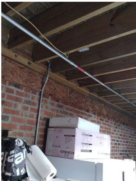
Electrical / Path To Array Roof/Attic - Conduit run, snap some shots showing the conduit is labeled and secured properly.
