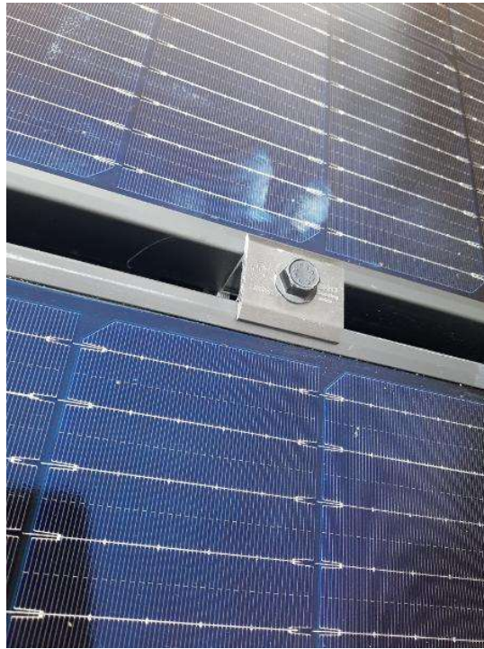
PV Arrays / Module Attachments - need to show modules are properly secured to racking.
