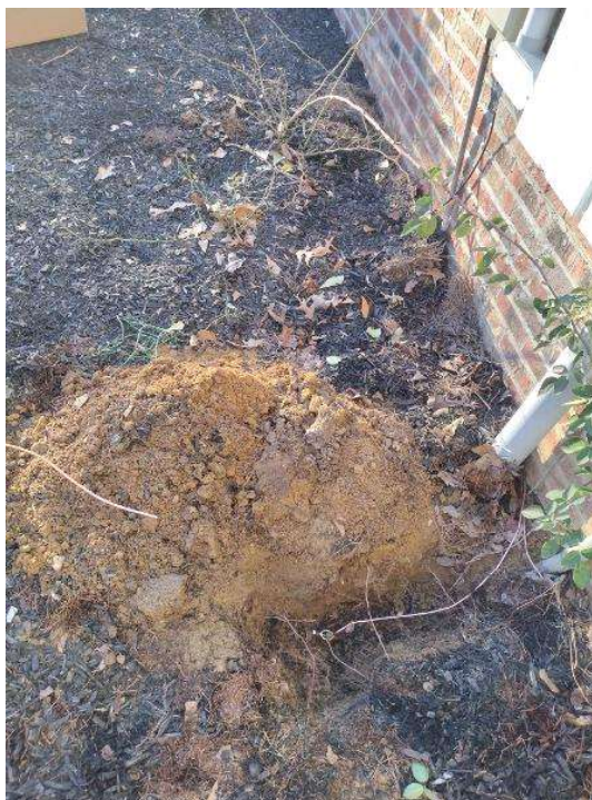
Electrical / Photo of the the GEC you installed and some clear shots of the acorns and clear shots of the pathway from our EGC to the existing EGC.
