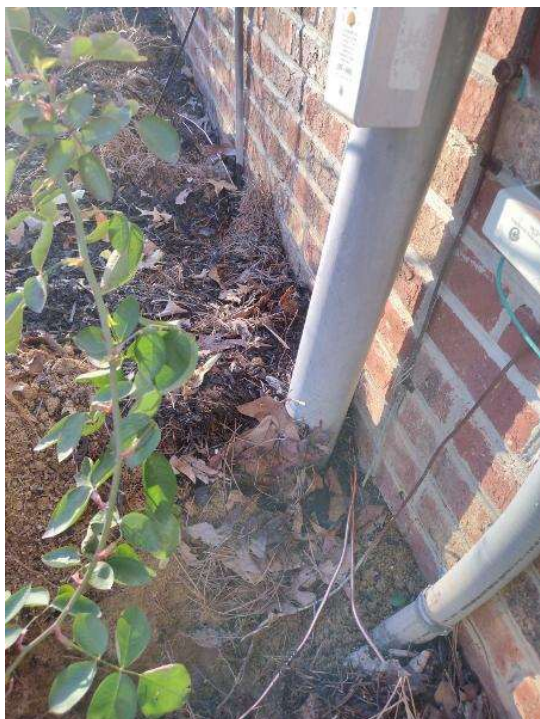
Electrical / GEC (Grounding Electrode Conductor) - Main GEC (photo of the home's grounding system)
