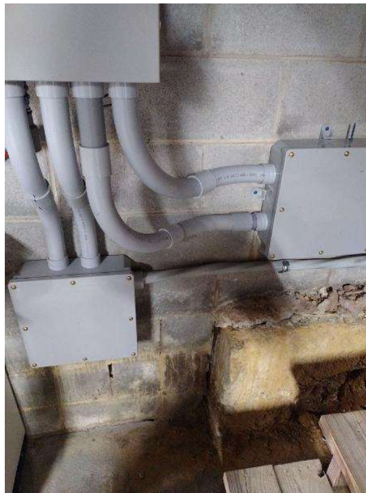
Electrical / PV Equipment - all PV equipment installed and completed, wiring, EGC (Solar Ground), entries/exits, open & closed boxes, completed overview.
