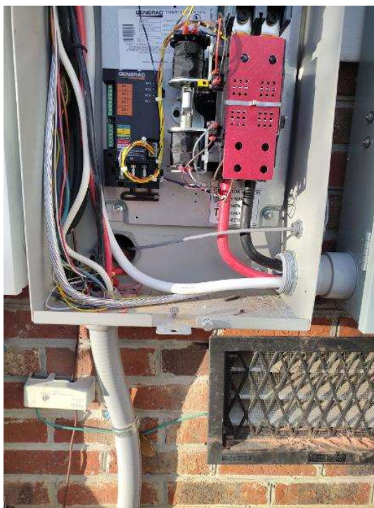
Electrical / MSP (Main Service Panel): Detailed photos of breaker installed
