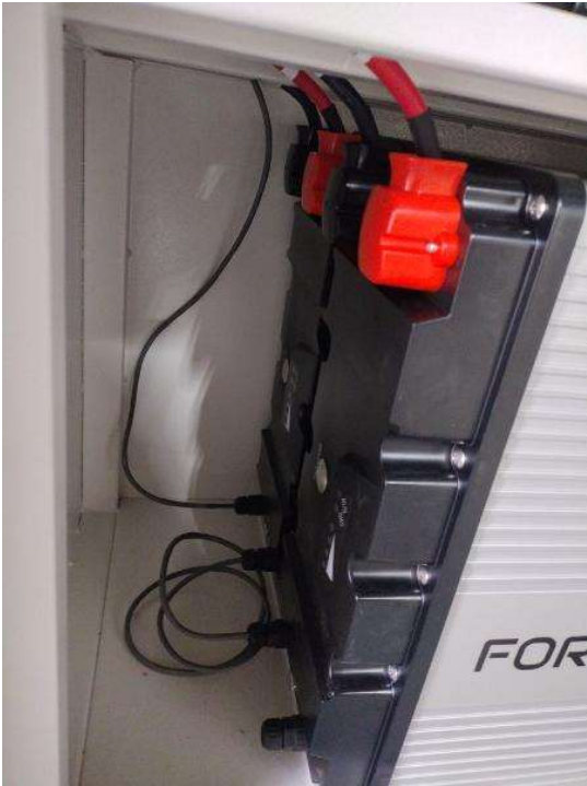
Electrical / Snap a photo of the connections at the battery.
