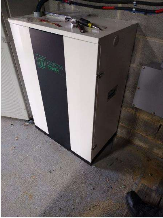
Electrical / Take a photo of the battery bank from the front and sides.
