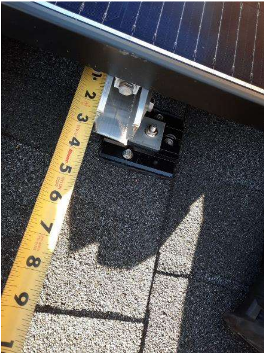
PV Arrays / Provide a photo of ALL rail cantilevers with measurements. "Cantilever" is how far the rail extends from the last mount at the edge of an array.
