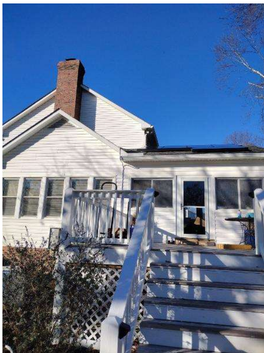
Electrical / Path To Array Roof/Attic - Conduit run, snap some shots showing the conduit is labeled and secured properly.
