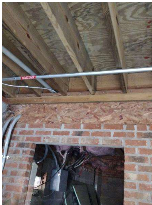
Electrical / Path To Array Roof/Attic - Conduit run, snap some shots showing the conduit is labeled and secured properly.
