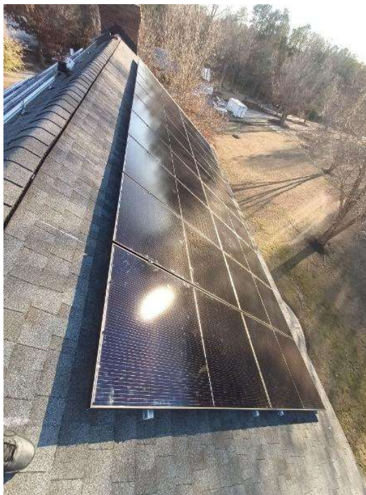
PV Arrays / Completed Array(s) showing COMPLETE overview of arrays with clean panels (No smears, handprints etc..) 3 pics per array from different angles showing each ENTIRE array.
