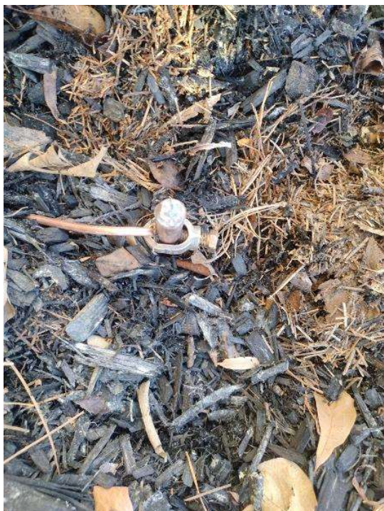
Electrical / GEC (Grounding Electrode Conductor) - Main GEC (photo of the home's grounding system)
