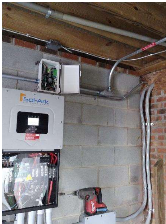
Electrical / Path To Array Roof/Attic - Conduit run, snap some shots showing the conduit is labeled and secured properly.
