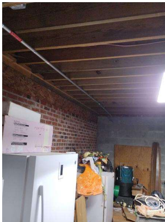
Electrical / Path To Array Roof/Attic - Conduit run, snap some shots showing the conduit is labeled and secured properly.
