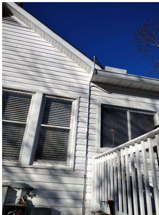
Electrical / Path To Array Roof/Attic - Conduit run, snap some shots showing the conduit is labeled and secured properly.
