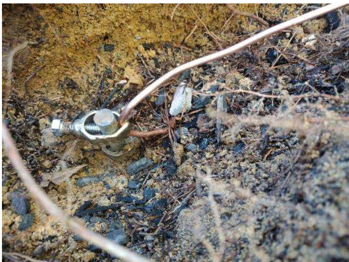
Electrical / Photo of the the GEC you installed and some clear shots of the acorns and clear shots of the pathway from our EGC to the existing EGC.
