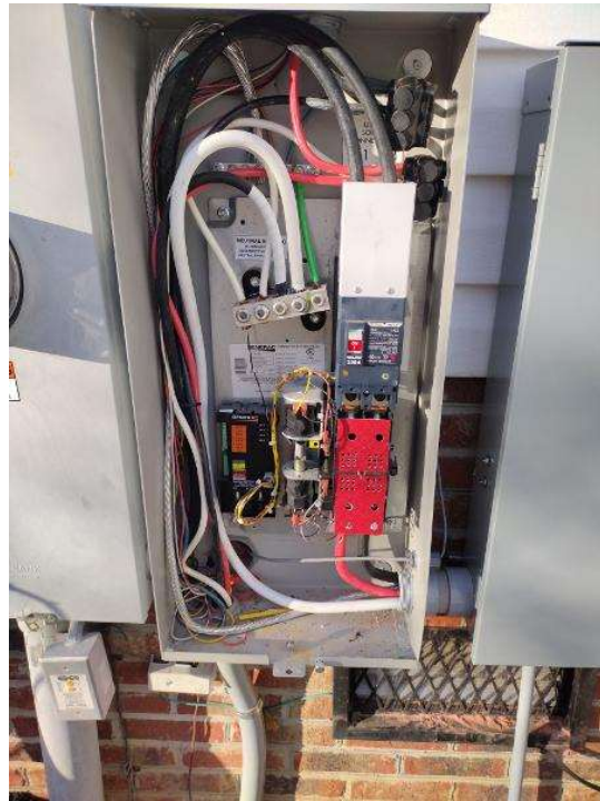
Electrical / MSP (Main Service Panel) - Photo of Entire Box After Interconnection
