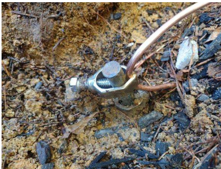
Electrical / GEC (Grounding Electrode Conductor) - Main GEC (photo of the home's grounding system)
