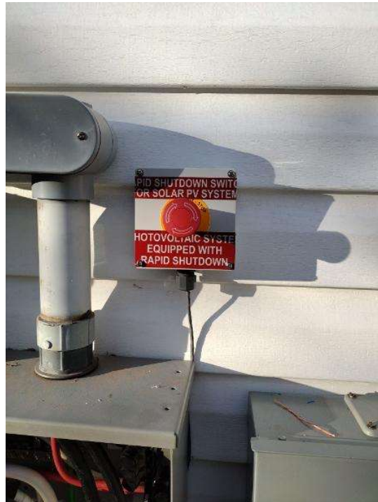
Electrical / Snap a photo of the inside of rapid shutdown switch. The outside too. With stickers. Take a few. Be liberal with it. If the RSD is just an AC disco then upload some redundant photos. It won't hurt yah.
