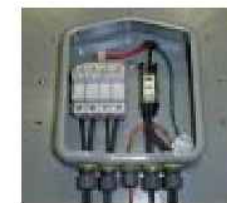
Model SD 0783-41, wired with Din Rail mounted fuse holders, bus bar and power distribution block.
