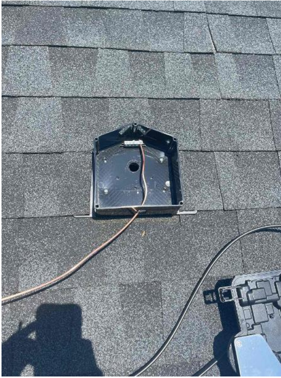
Smart Sun Energy (Super Nova Solar, LLC) Loc: 35.2355, -78.9649
