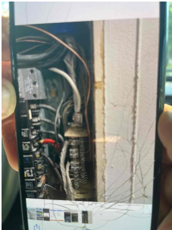
Smart Sun Energy (Super Nova Solar, LLC) Loc: 35.2355, -78.9654
