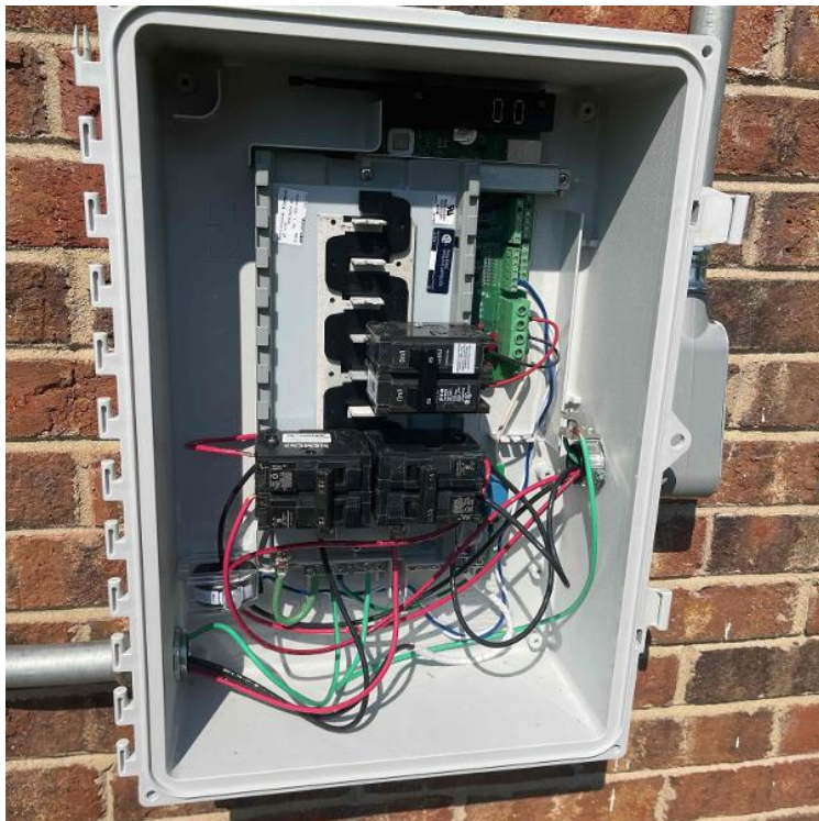
Smart Sun Energy (Super Nova Solar, LLC) Loc: 35.2354, -78.9651
