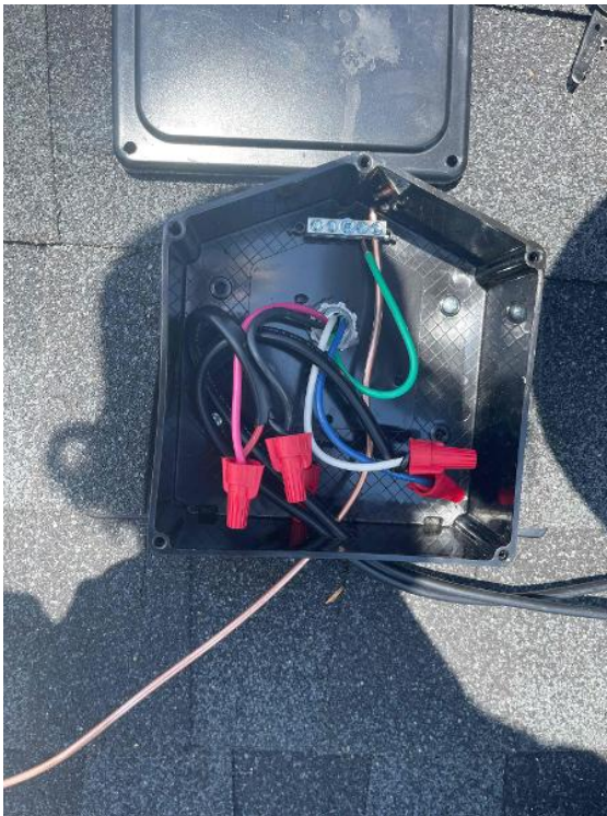
Smart Sun Energy (Super Nova Solar, LLC) Loc: 35.2355, -78.965
