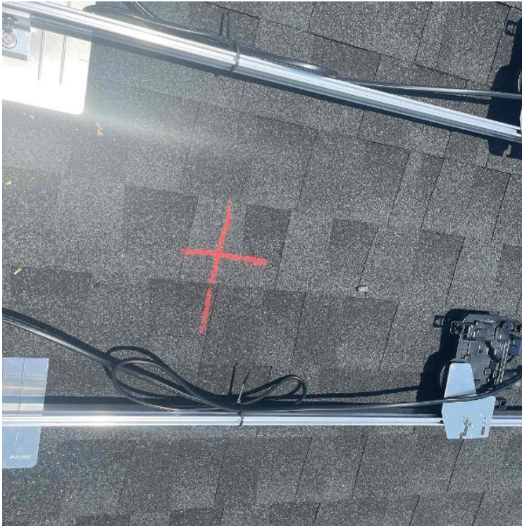
Smart Sun Energy (Super Nova Solar, LLC) Loc: 35.2355, -78.9649
