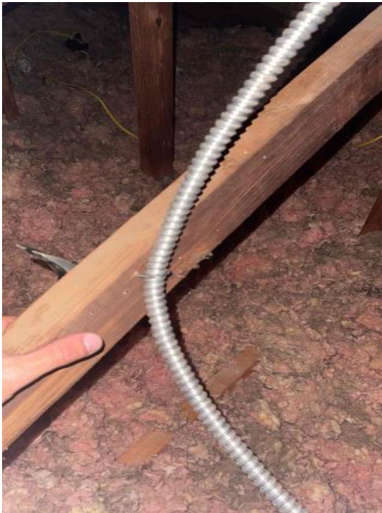
Smart Sun Energy (Super Nova Solar, LLC)
