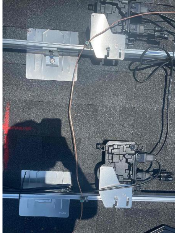
Smart Sun Energy (Super Nova Solar, LLC) Loc: 35.2355, -78.9648
