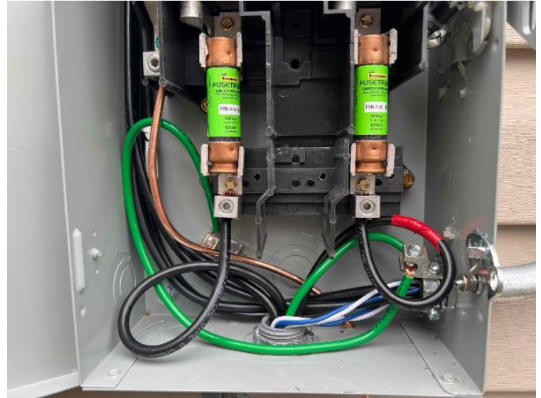
Electrical / AC Disconnect - Photos of fuse sizes and wire sizes
