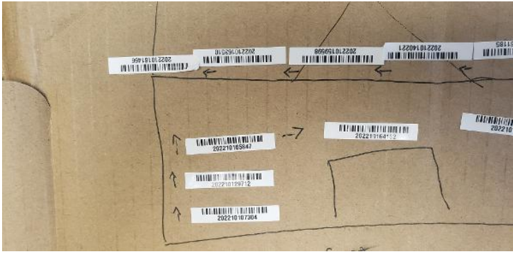
Completion / STICKER MAP: Optimizer/micro-inverter stickers and sticker map showing layout and string map to j-box
