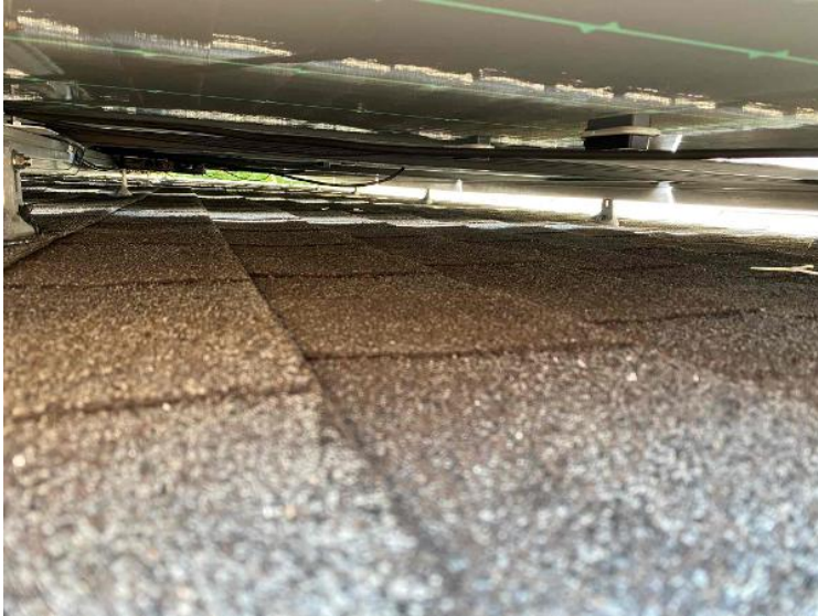
Roof / Wire Management - Quality pictures (need to show the entire array under the panel through pictures.absolutely no dangling wires)
