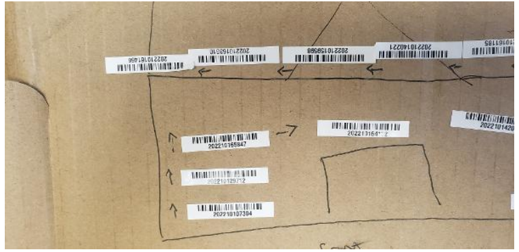
Completion / STICKER MAP: Optimizer/micro-inverter stickers and sticker map showing layout and string map to j-box
