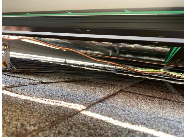
Roof / Wire Management - Quality pictures (need to show the entire array under the panel through pictures.absolutely no dangling wires)
