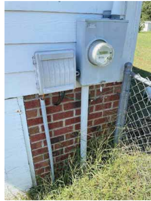
UTILITY COMPANY: Duke Energy NC
