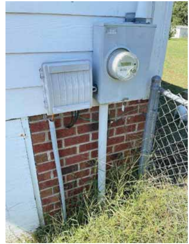
UTILITY COMPANY: Duke Energy NC
