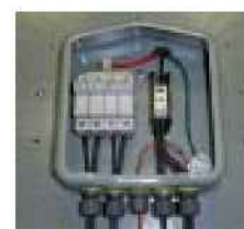
Model SD 0783-41, wired with Din Rail mounted fuse holders, bus bar and power distribution block.
