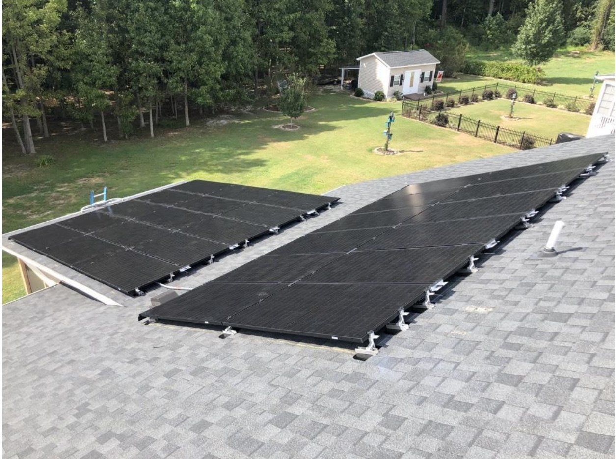
Hale, Rick, 20 Dot CourtFuquay-Varina, NC 27526- PV Inspection Pictures
