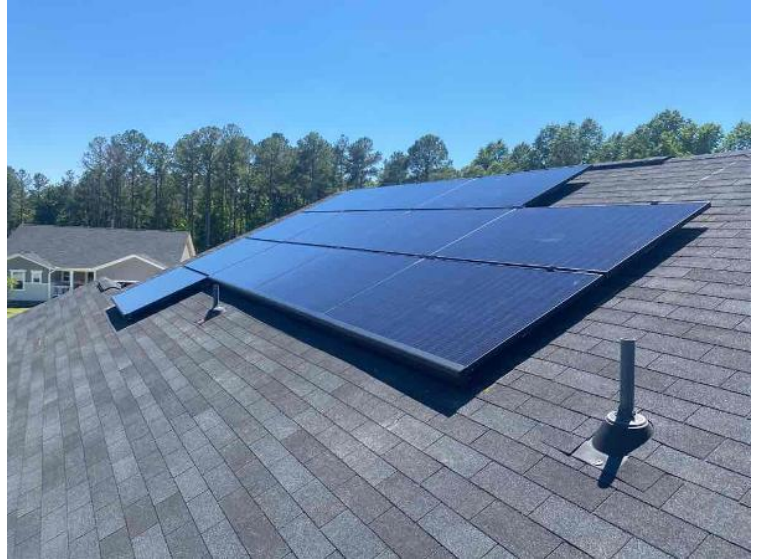
Roof - ARRAY(s) COMPLETED: showing COMPLETE overview of arrays multiple pics and location of soladek (3 pics per array min.) (no close up pics)
