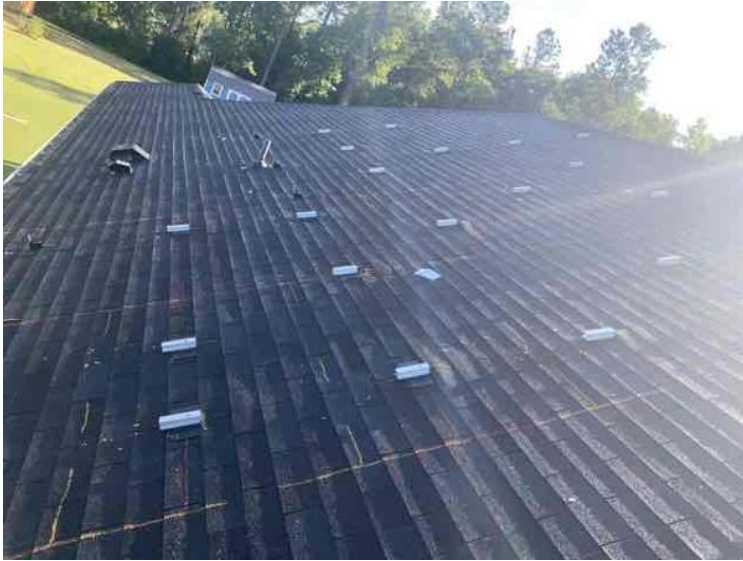
Roof - ATTACHMENT LAYOUT - showing COMPLETE layouts, staggered attachments, span measurement and picture of the mount flashings installed correctly. (2 pics per array min)
