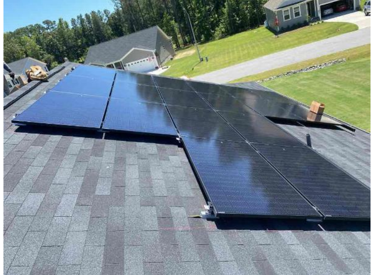
Roof - ARRAY(s) COMPLETED: showing COMPLETE overview of arrays multiple pics and location of soladek (3 pics per array min.) (no close up pics)
