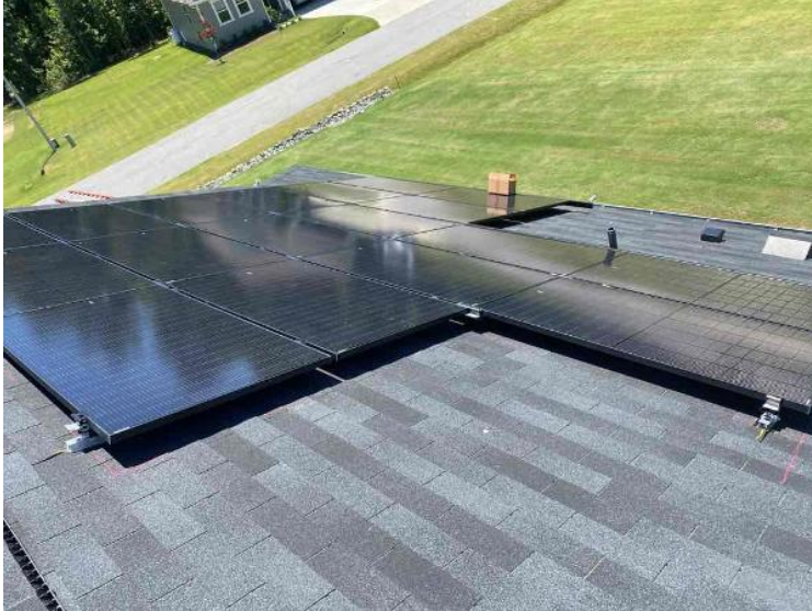
Roof - ARRAY(s) COMPLETED: showing COMPLETE overview of arrays multiple pics and location of soladek (3 pics per array min.) (no close up pics)
