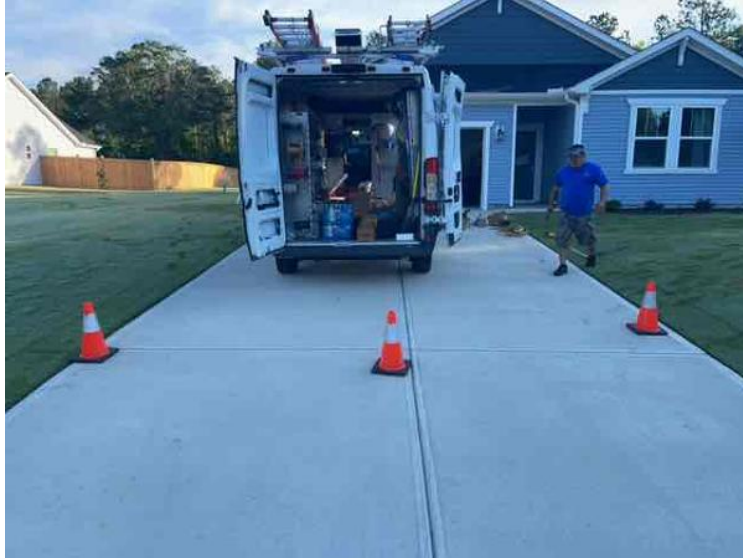
Job Setup - RAZ - Restricted area zones, safety cones and hazard tape. This needs to be completed prior to starting work.
