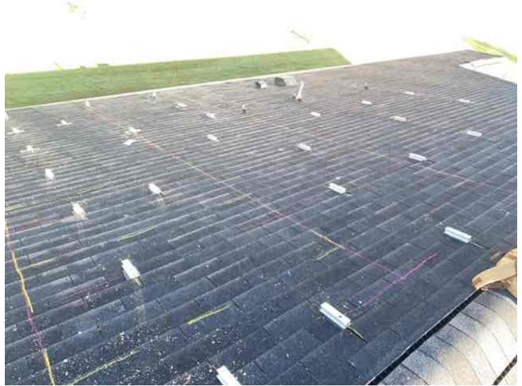
Roof - ATTACHMENT LAYOUT - showing COMPLETE layouts, staggered attachments, span measurement and picture of the mount flashings installed correctly. (2 pics per array min)
