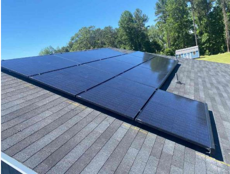
Roof - ARRAY(s) COMPLETED: showing COMPLETE overview of arrays multiple pics and location of soladek (3 pics per array min.) (no close up pics)
