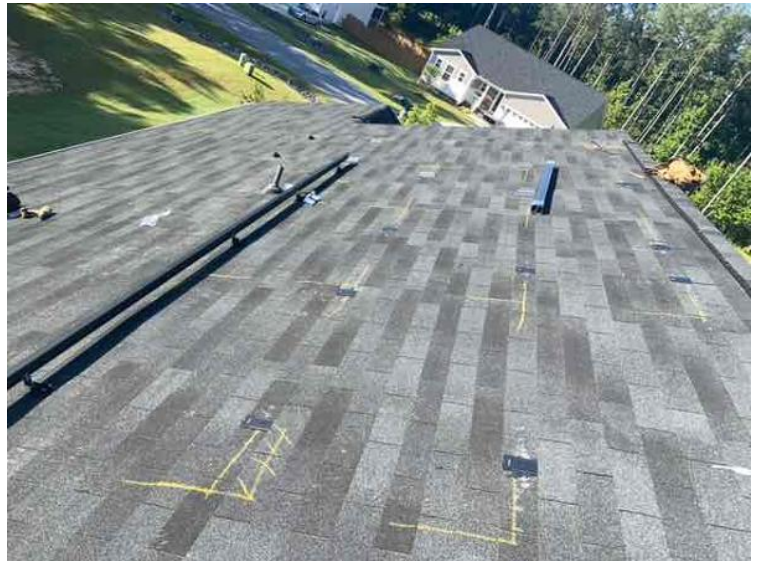
Roof - ATTACHMENT LAYOUT - showing COMPLETE layouts, staggered attachments, span measurement and picture of the mount flashings installed correctly. (2 pics per array min)
