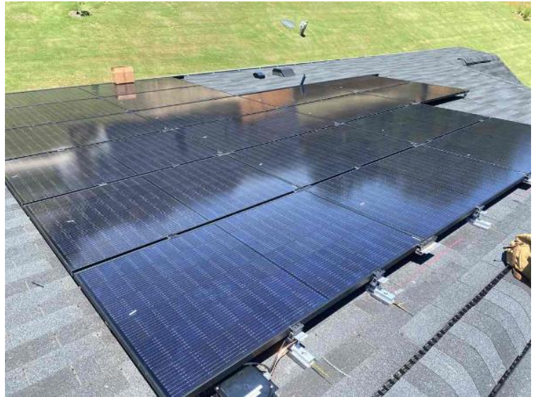
Roof - ARRAY(s) COMPLETED: showing COMPLETE overview of arrays multiple pics and location of soladek (3 pics per array min.) (no close up pics)
