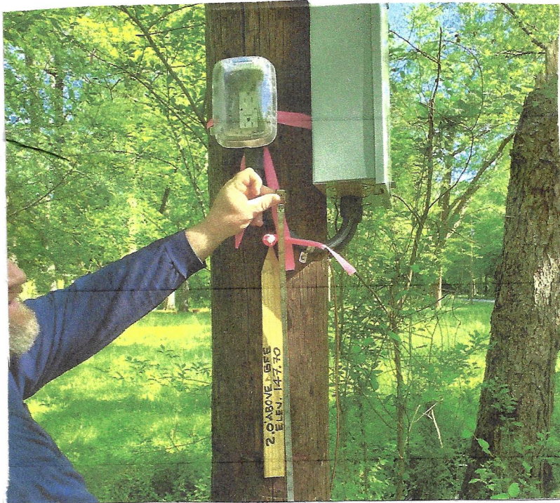
Photo One Caption ELECTRIC PANEL
