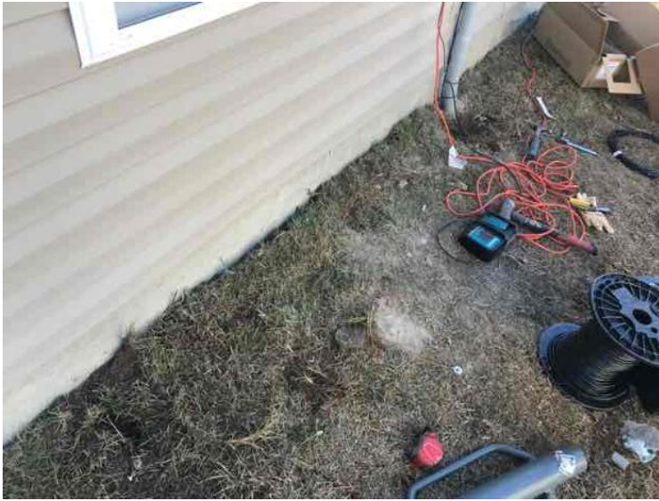
Roof/Array Information - Photo: Conduit Run
