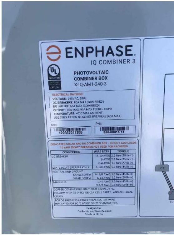
Electrical Information - Photo: Inverter Data Plate
