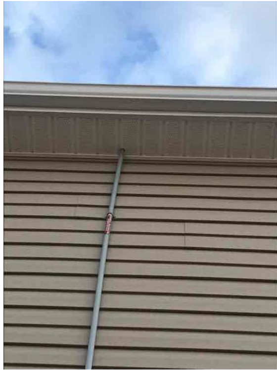
Roof/Array Information - Photo: Conduit Run
