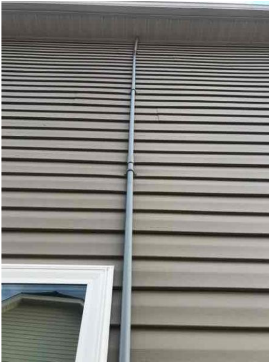
Roof/Array Information - Photo: Conduit Run
