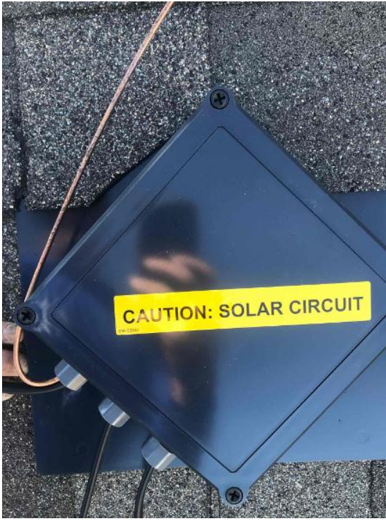
Roof/Array Information - Photo: Junction Box Location
