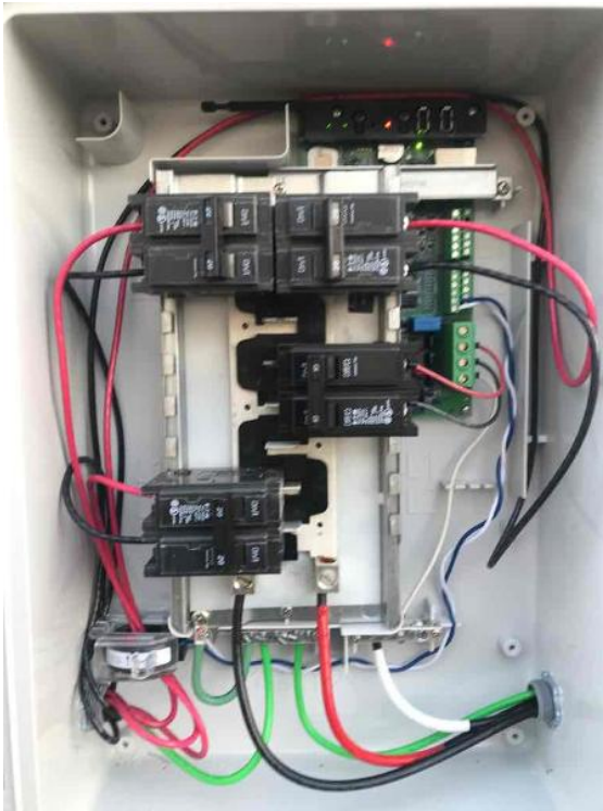
Electrical Information - Photo: Electrical Component Overview
