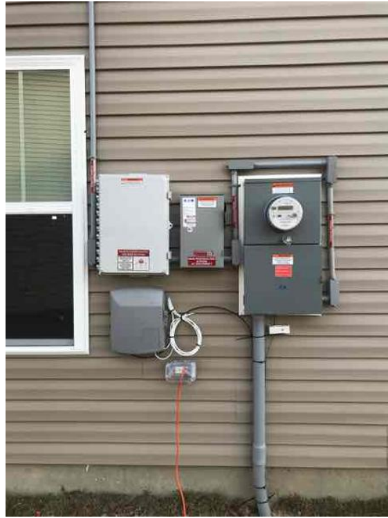
Roof/Array Information - Photo: Conduit Run
