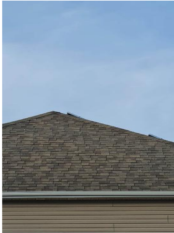
Roof/Array Information - Photo: Overall Array
