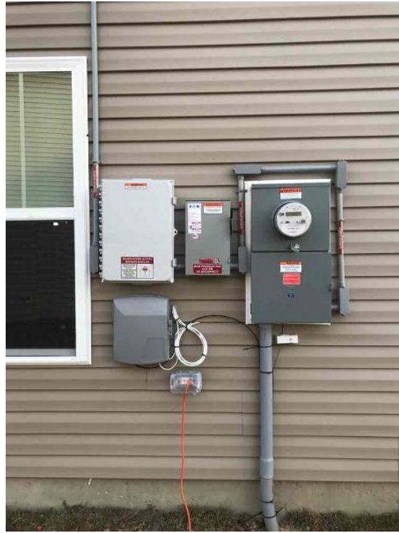
Electrical Information - Photo: Electrical Component Overview
