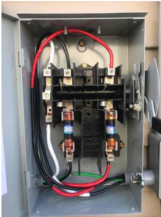
Electrical Information - Photo: AC Disconnect
