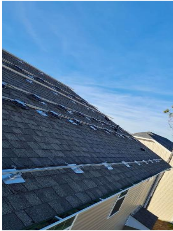
Roof/Array Information - Photo: Under Array (wire management)
