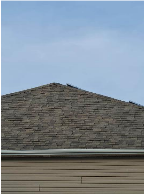
Roof/Array Information - Photo: Overall Array
