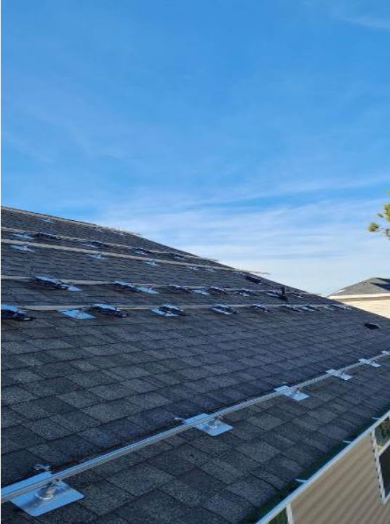
Roof/Array Information - Photo: Under Array (wire management)
