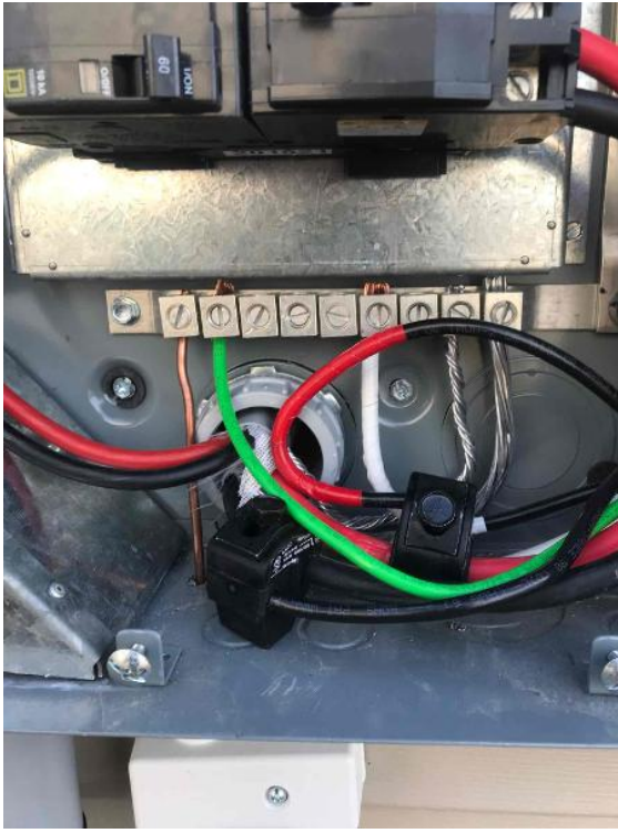
Electrical Information - Photo: Main Service Panel
