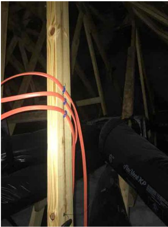
Roof/Array Information - Photo: Conduit Run
