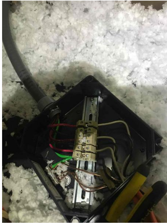
Roof/Array Information - Photo: Junction Box Location
