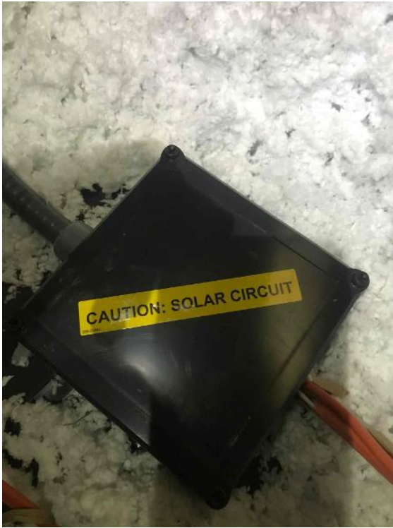
Roof/Array Information - Photo: Junction Box Location
