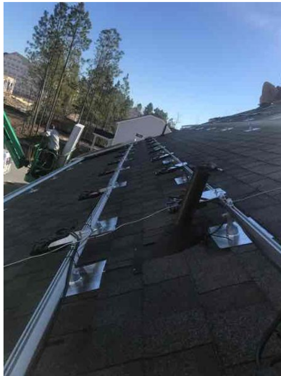
Electrical Information - Photo: Inverter(s)
