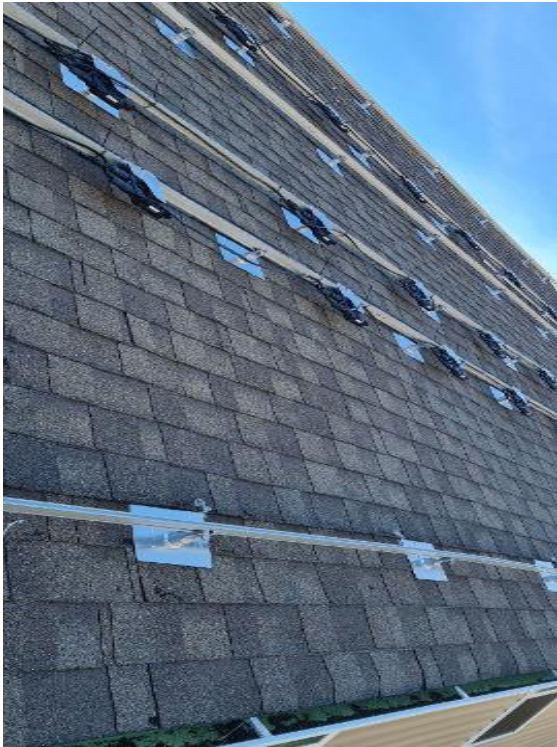
Roof/Array Information - Photo: Under Array (wire management)
