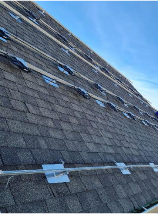
Roof/Array Information - Photo: Under Array (wire management)
