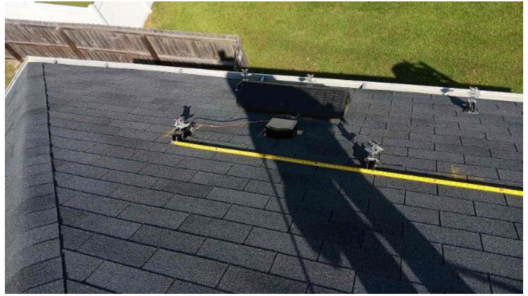
Module Installation / Ready for Modules (All rail-less parts required to land modules complete)
