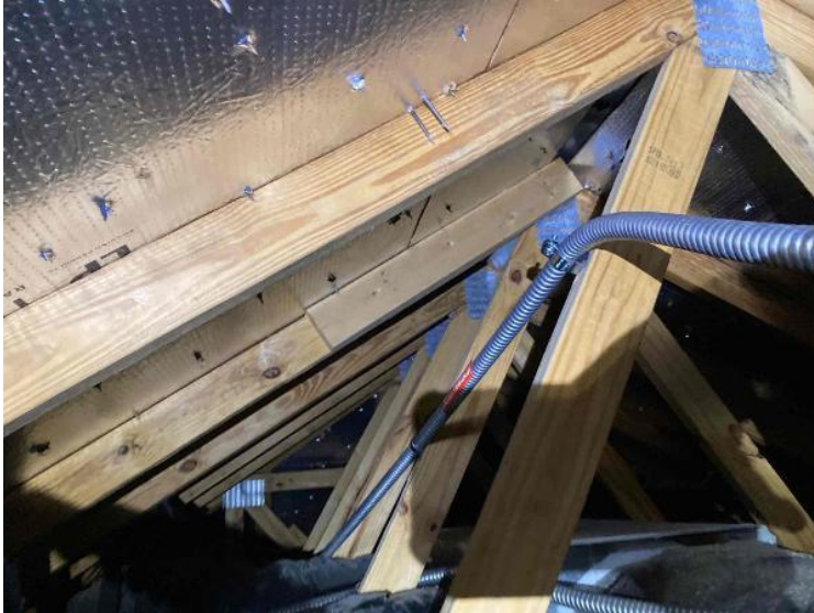
Rooftop Conduit Run / Conduit Run: Overall Run Between Arrays, Down To Conduit Leaving Roof (Support every 5' for Sunrun jobs)
