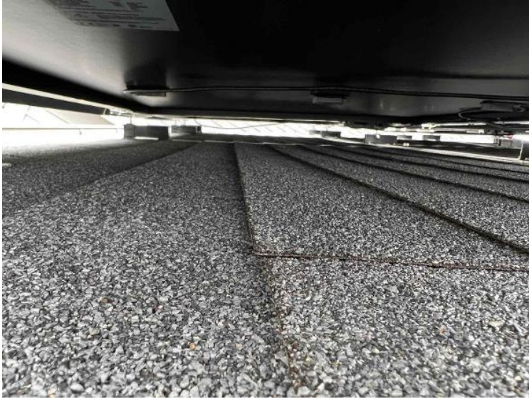
Module Installation / Wire management Under the Array (1 photo per row of modules per array)
