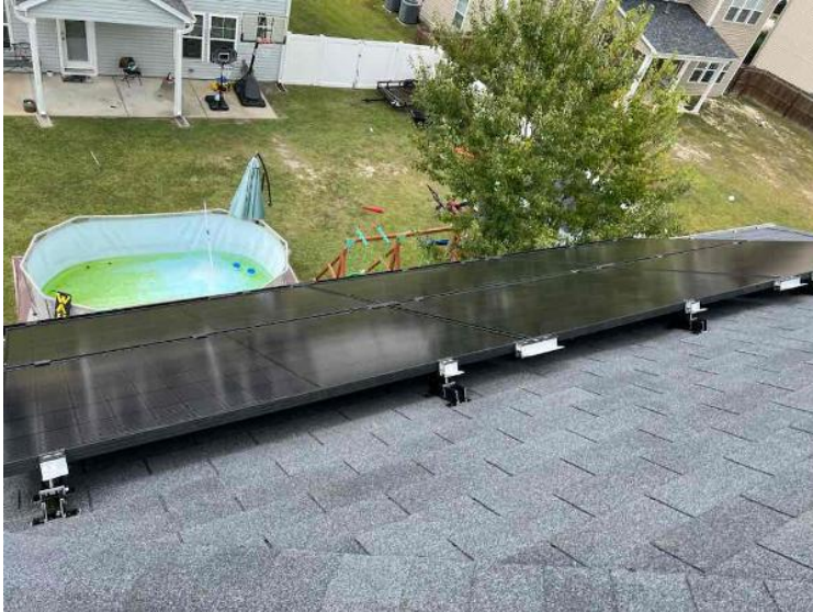
Project Completion Photos / Complete Array Photos (all modules can be counted in each array)
