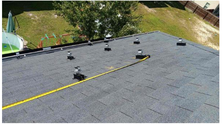
Module Installation / Ready for Modules (All rail-less parts required to land modules complete)
