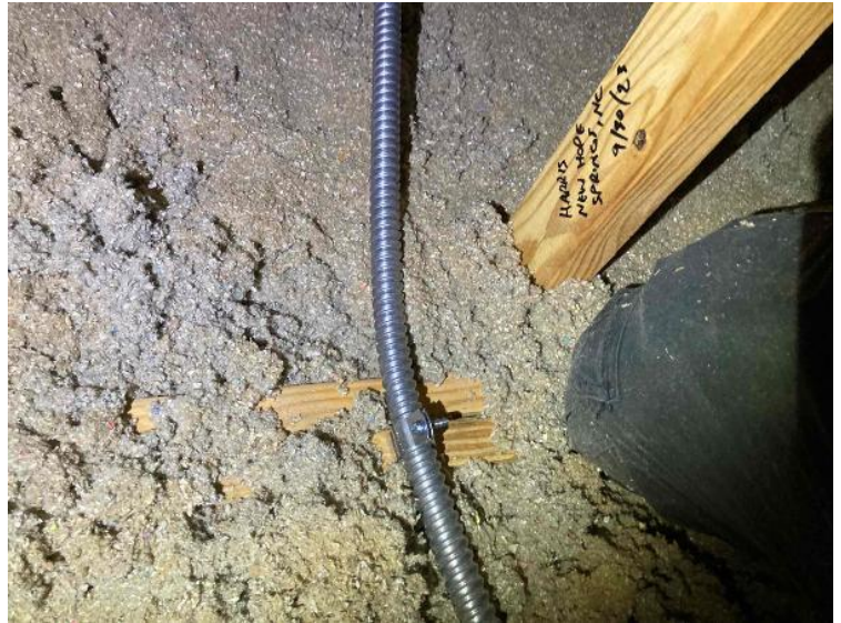
Rooftop Conduit Run / Conduit Run: Overall Run Between Arrays, Down To Conduit Leaving Roof (Support every 5' for Sunrun jobs)
