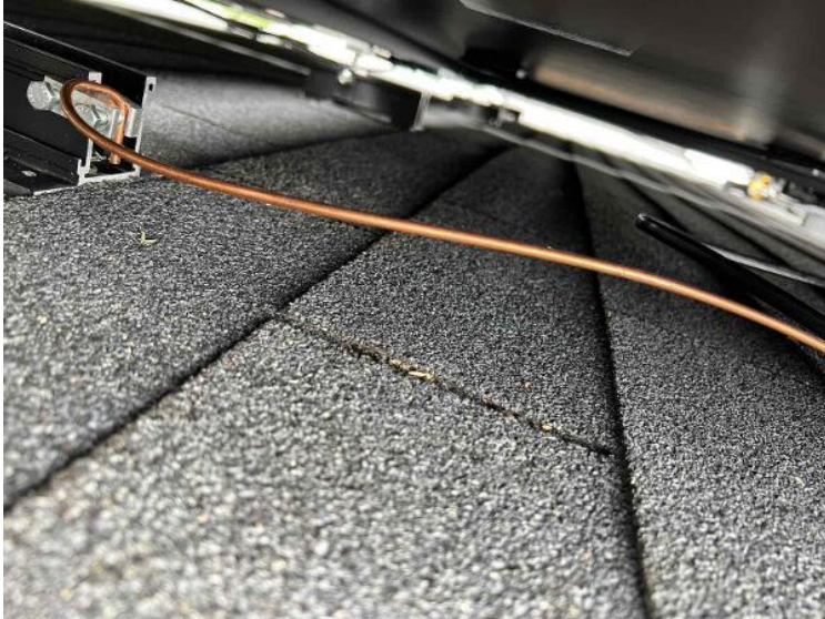
Module Installation / Wire management Under the Array (1 photo per row of modules per array)
