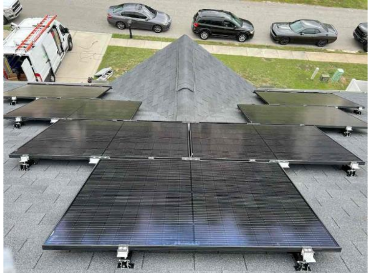
Project Completion Photos / Complete Array Photos (all modules can be counted in each array)
