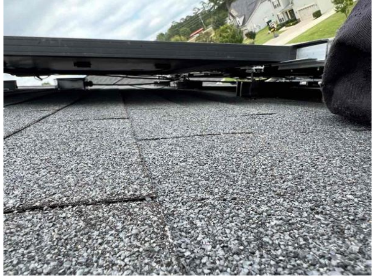
Module Installation / Wire management Under the Array (1 photo per row of modules per array)
