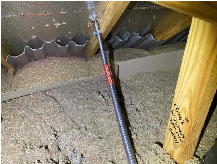
Rooftop Conduit Run / Conduit Run: Overall Run Between Arrays, Down To Conduit Leaving Roof (Support every 5' for Sunrun jobs)
