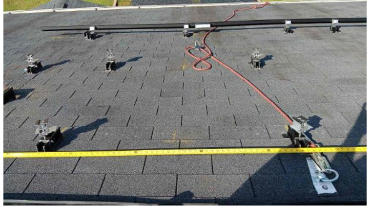
Module Installation / Ready for Modules (All rail-less parts required to land modules complete)
