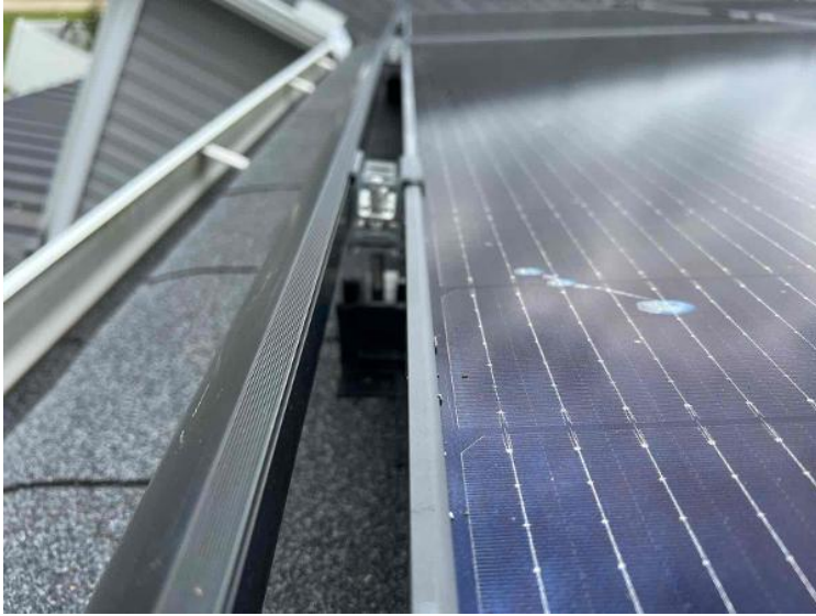
Module Installation / Close Up of Trimrail Splice + Trimrail Clip + Trimrail Roof Attachment Complete
