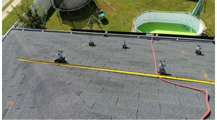
Module Installation / Ready for Modules (All rail-less parts required to land modules complete)
