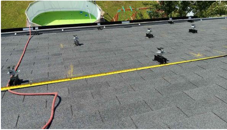
Module Installation / Ready for Modules (All rail-less parts required to land modules complete)
