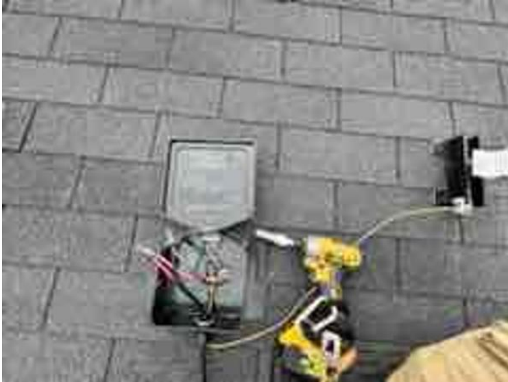
Rooftop Conduit Run / Close up photo of Weep Holes + Wet Rated Wire Nuts /Terminal Blocks + Duct Seal complete
