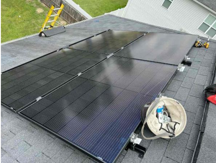
Project Completion Photos / Complete Array Photos (all modules can be counted in each array)
