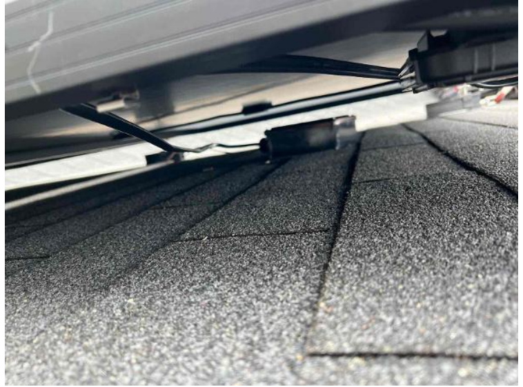
Module Installation / Wire management Under the Array (1 photo per row of modules per array)
