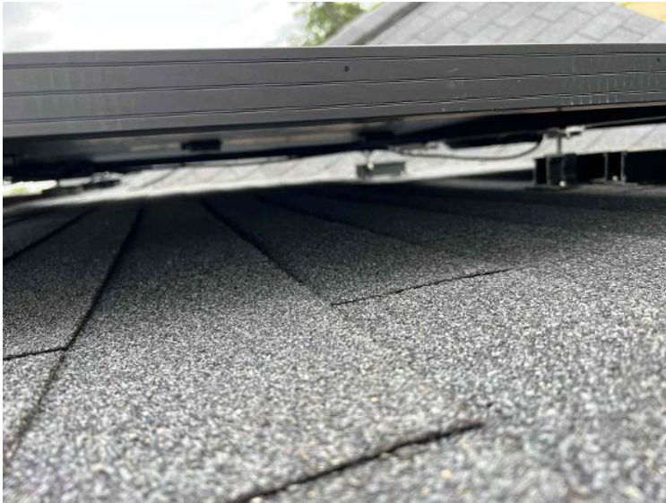
Module Installation / Wire management Under the Array (1 photo per row of modules per array)
