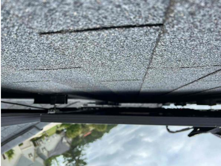
Module Installation / Wire management Under the Array (1 photo per row of modules per array)
