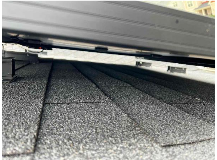
Module Installation / Wire management Under the Array (1 photo per row of modules per array)
