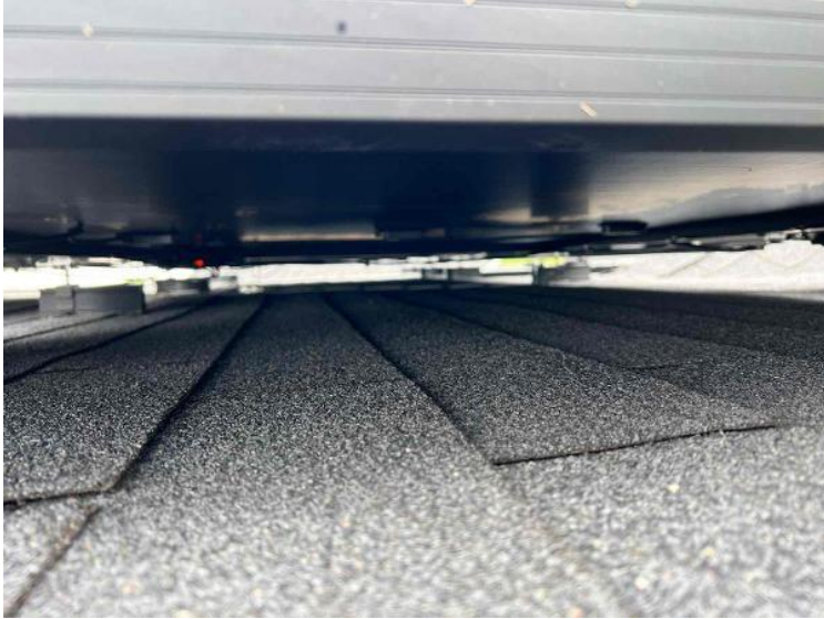
Module Installation / Wire management Under the Array (1 photo per row of modules per array)
