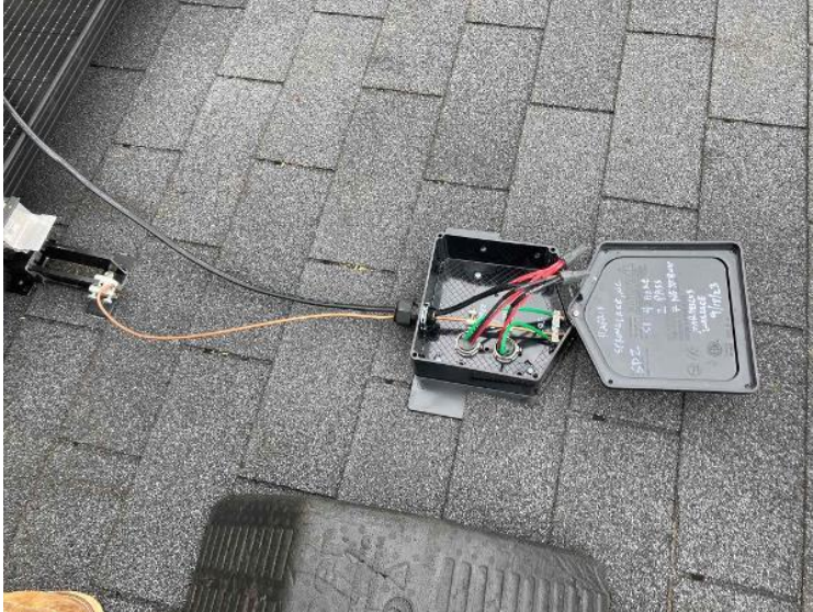
Rooftop Conduit Run / Close up photo of Weep Holes + Wet Rated Wire Nuts /Terminal Blocks + Duct Seal complete
