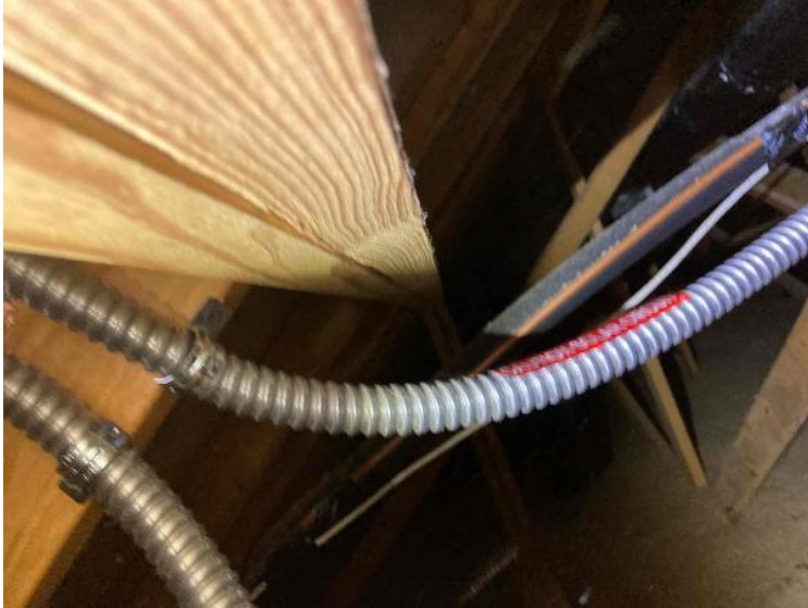
Rooftop Conduit Run / Conduit Run: Overall Run Between Arrays, Down To Conduit Leaving Roof (Support every 5' for Sunrun jobs)
