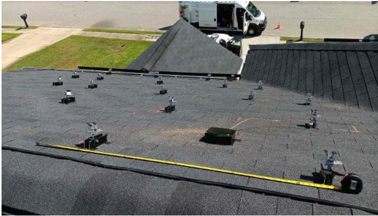
Module Installation / Ready for Modules (All rail-less parts required to land modules complete)
