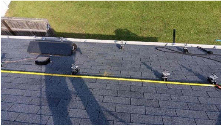
Module Installation / Ready for Modules (All rail-less parts required to land modules complete)
