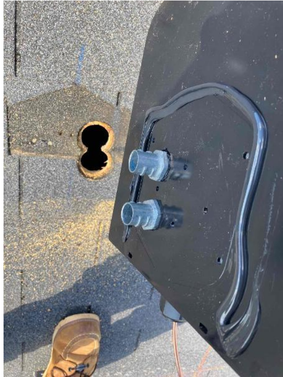
Rooftop Conduit Run / Conduit Support Flashing (U-Shape Seal + Installed)
