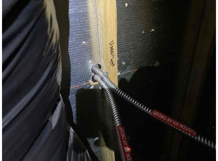
Rooftop Conduit Run / Conduit Run: Overall Run Between Arrays, Down To Conduit Leaving Roof (Support every 5' for Sunrun jobs)
