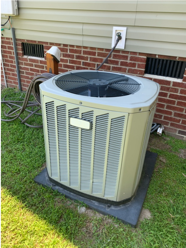
Photos of Existing Outdoor Systems to be Removed (4 of 4)
