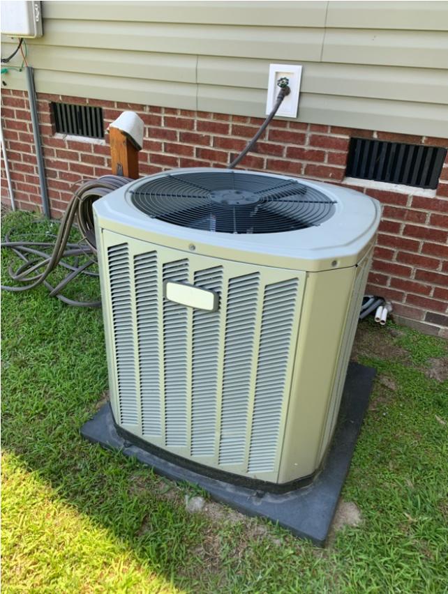
Photo of New OUTDOOR UNIT location (2 of 3)
