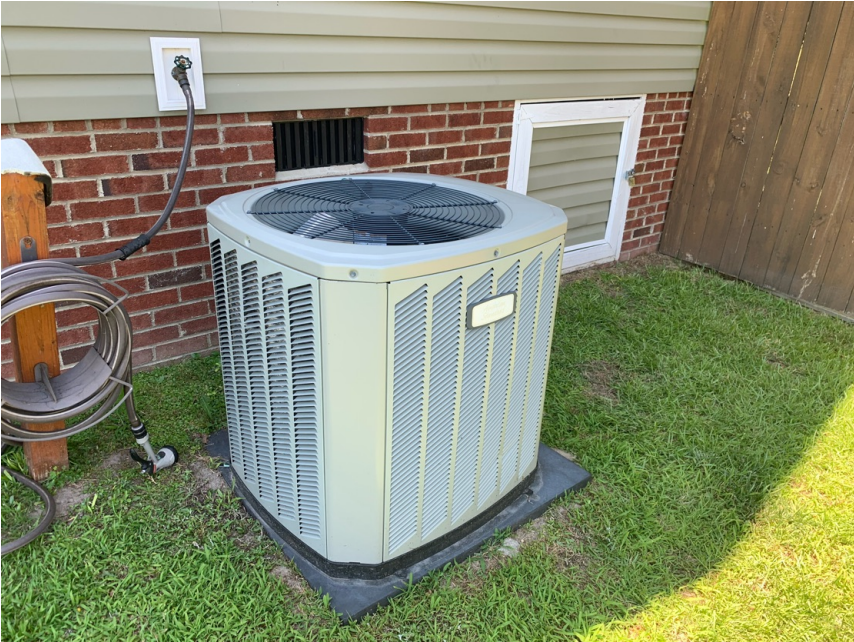
Photo of New OUTDOOR UNIT location (1 of 3)
