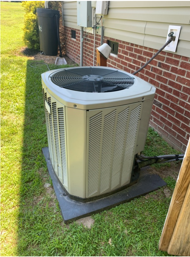
Photo of New OUTDOOR UNIT location (3 of 3)
