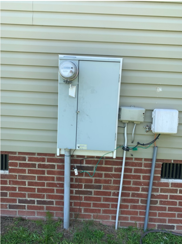
Photo of existing electrical panel & Breaker (2 of 2)
