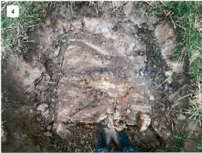
View of Deteriorated Outlet Lid Before Removal
