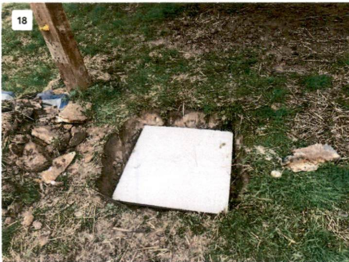
View of Temporary Lid Placed Over Deteriorated Outlet Lid by Inspector
