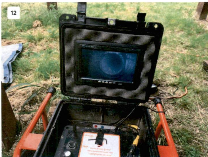
View of Inside of Distribution Box
