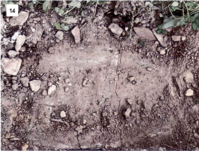
View of Cracked Distribution Box Lid
