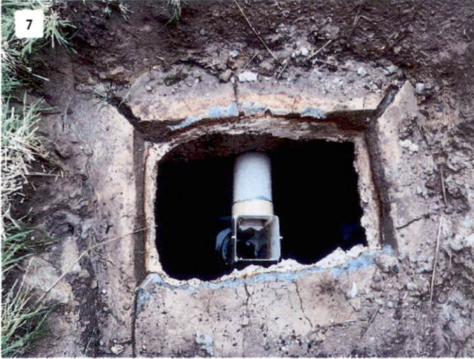
View of Large Cracks and Significant Deterioration
