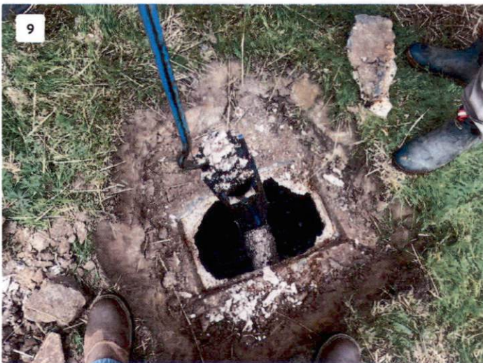
View of Dirty Outlet Tee Filter
