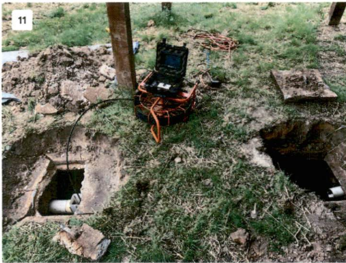
View of Drain Camera Used to Locate and View Distribution Box
