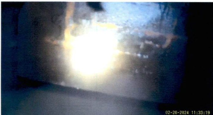
Septic Tank wall signs of deterioration
