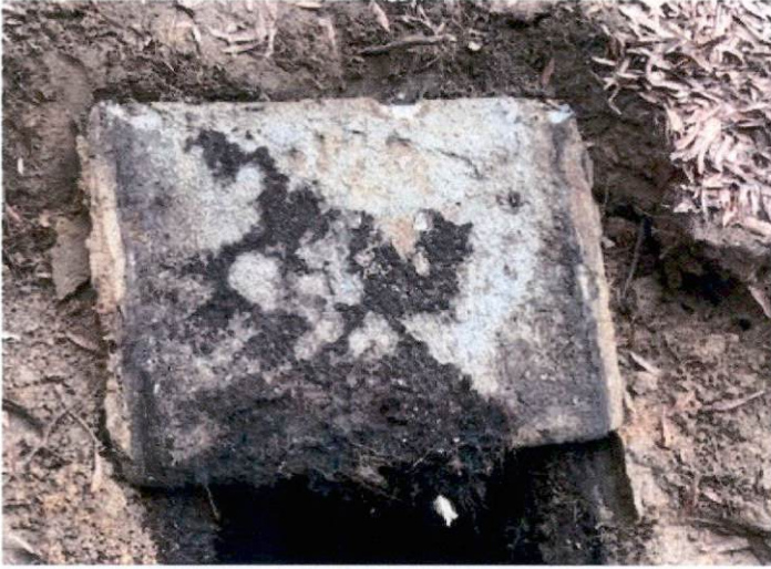
Lid cover is cracked
