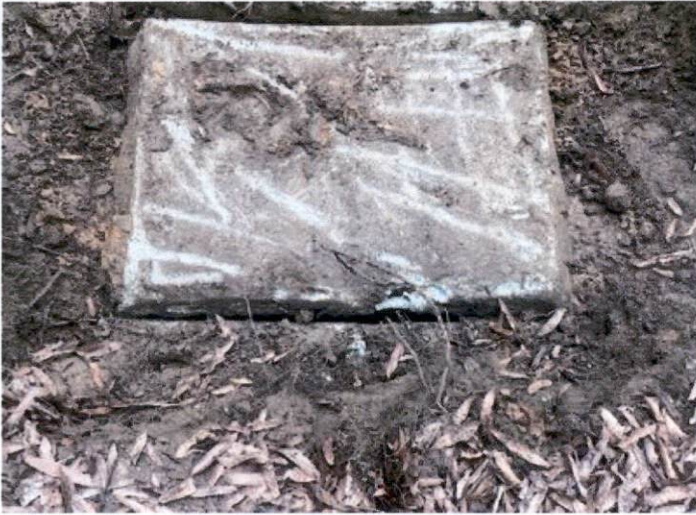
Signs of infiltration
