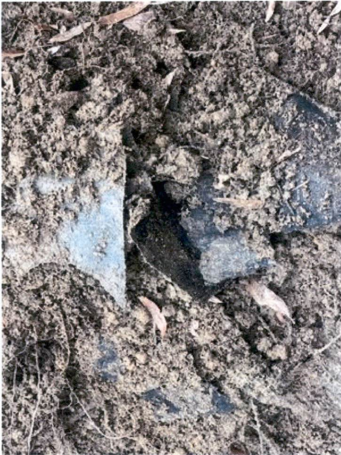
The inlet lid caover had what appears to be Geotextile fabric over the cover
