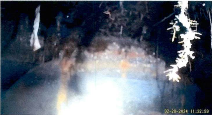
Small roots in septic tank
