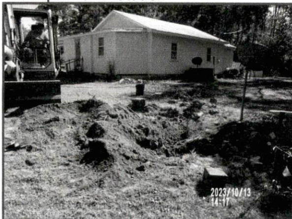
P1. Septic Tank Location
