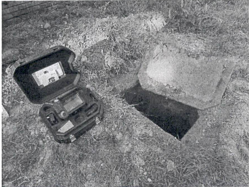
Figure 3 Removed the lid to expose the drain line & setup our Wohler 700 sewer scope
