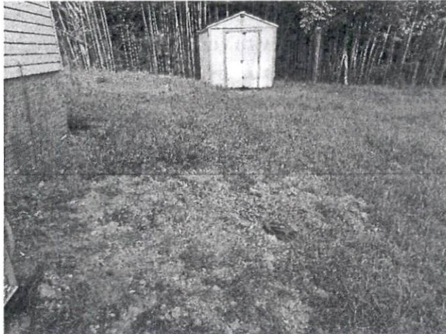
Figure 1 Condition of septic area upon arrival
