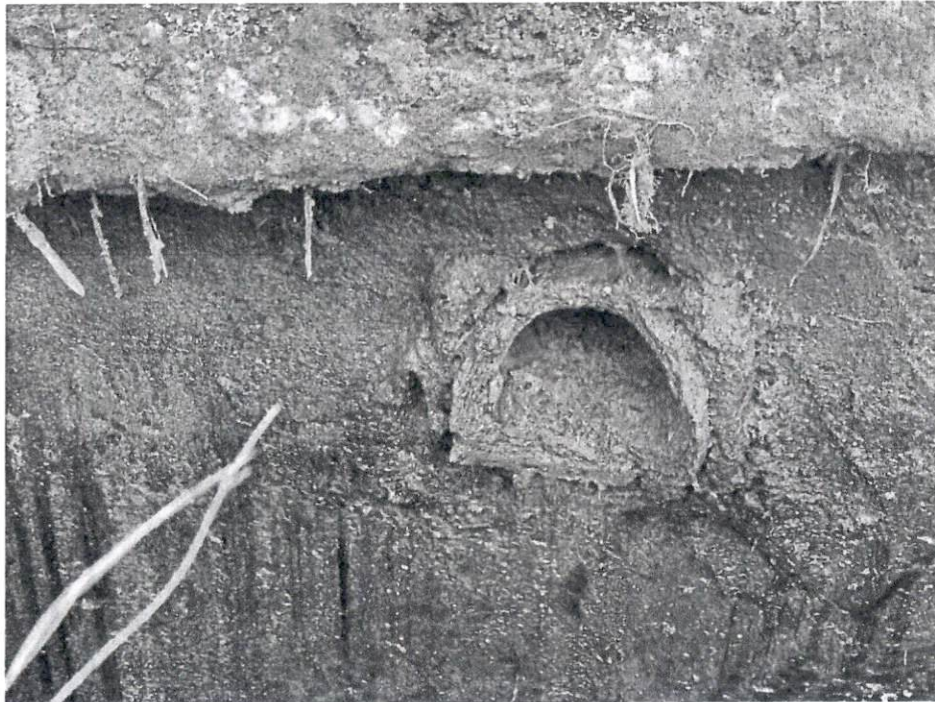
Figure 4 This is the condition of the tank outlet pipe
