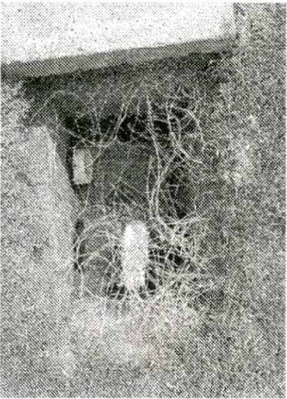
5. Inside view of Distribution box (grass roots)
