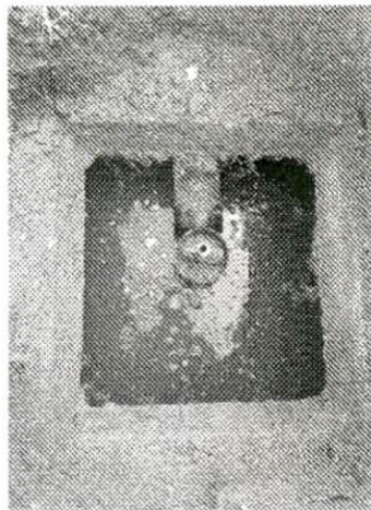
2. Outlet side of septic tank
