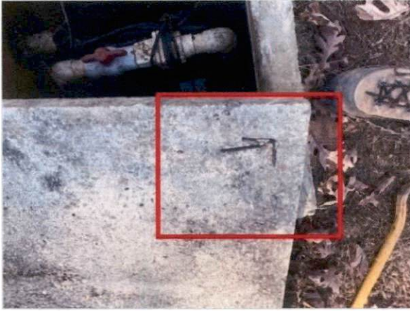
Pump tank riser cover signs of deterioration exposed rebar.
