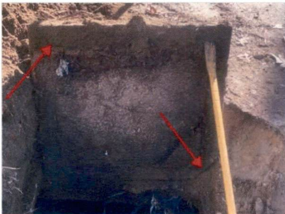
Inlet lid cover chipped and cracked
