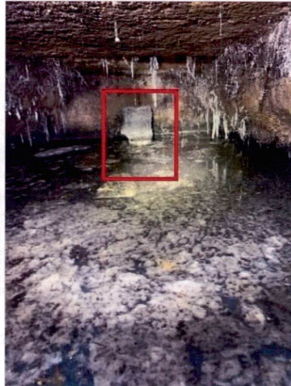
Outlet T missing filter
