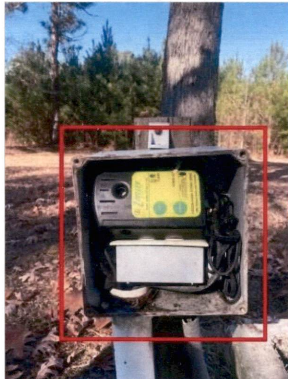
Control box alarm not functioning when tested missing breaker and safety switch
