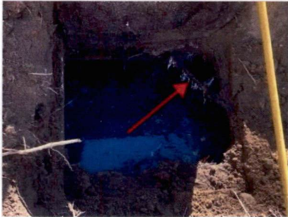
Root penetrating septic tank
