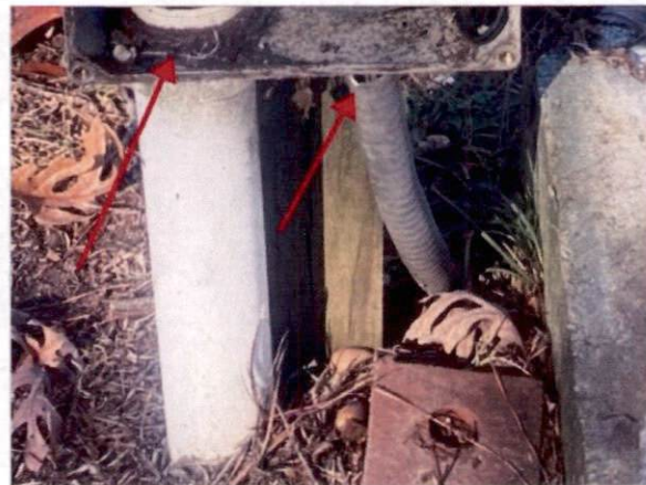
Control box conduit rusted and not secure
