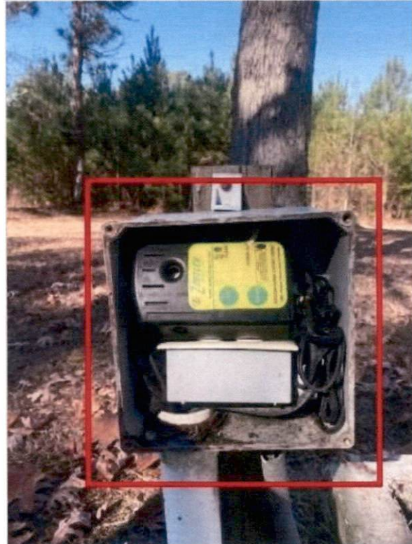
Control box alarm not functioning when tested missing breaker and safety switch
