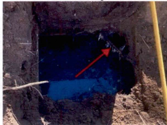
Root penetrating septic tank
