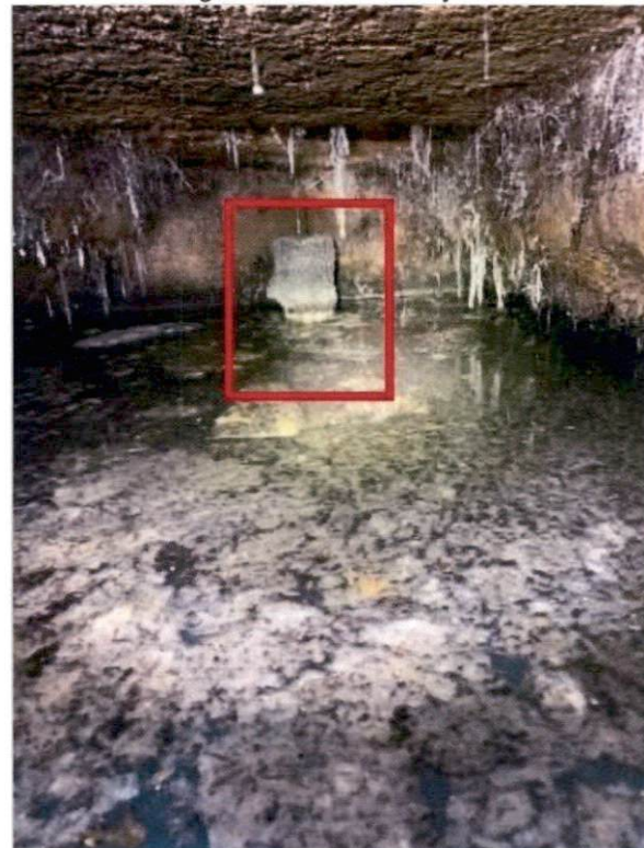
Outlet T missing filter
