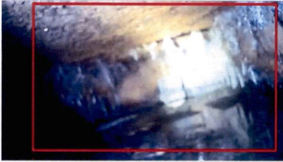
Roots inside septic tank
