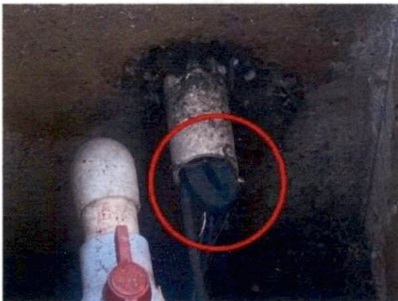
conduit from pump tank to control box not sealed
