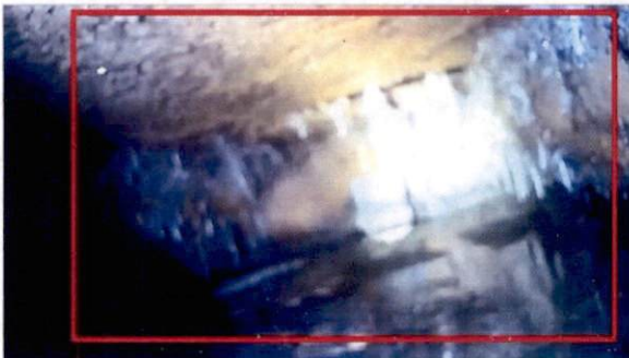
Roots inside septic tank
