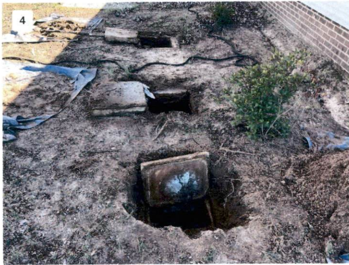
View of Location of Distribution Box
