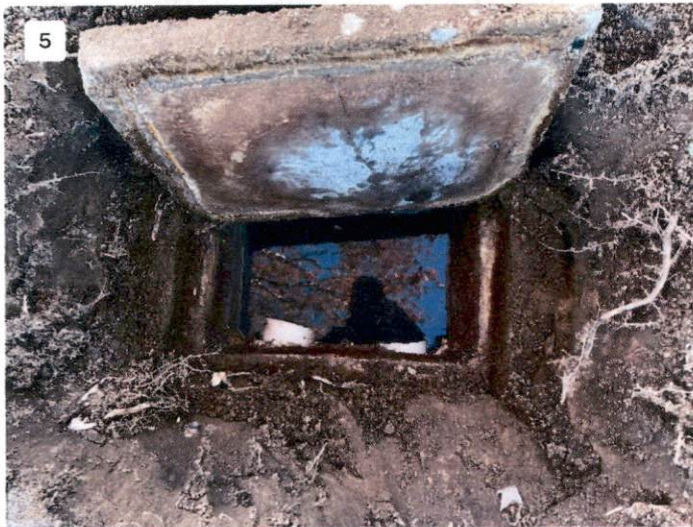
View of Inside of Distribution Box
