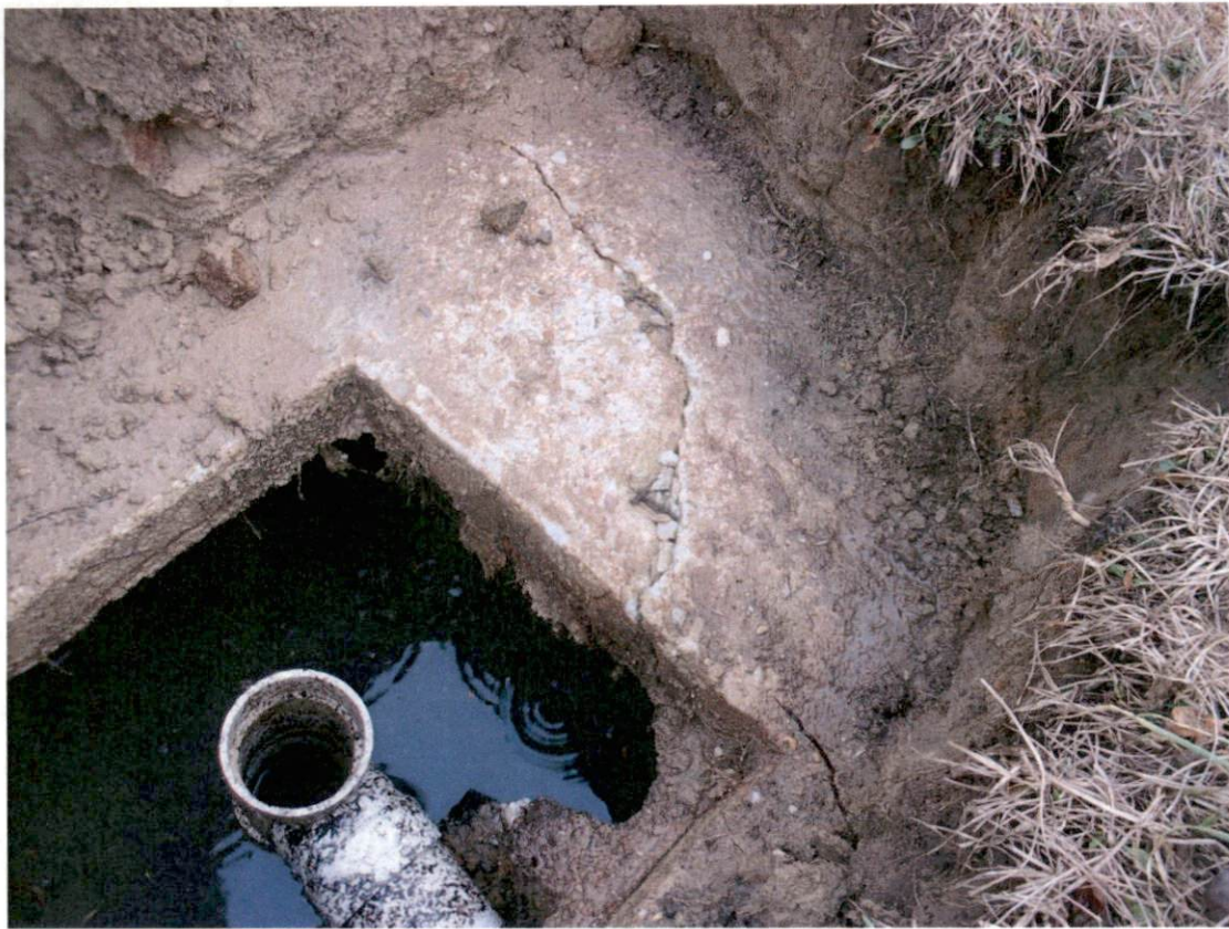
Large Crack on the Outlet Side of the Septic Tank
