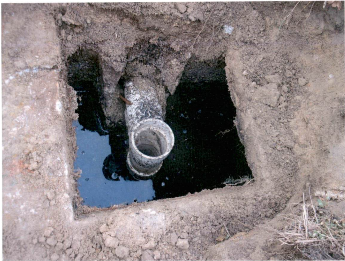
Outlet Access Point of the Septic Tank Showing Effluent Level Approximately 6" Low
