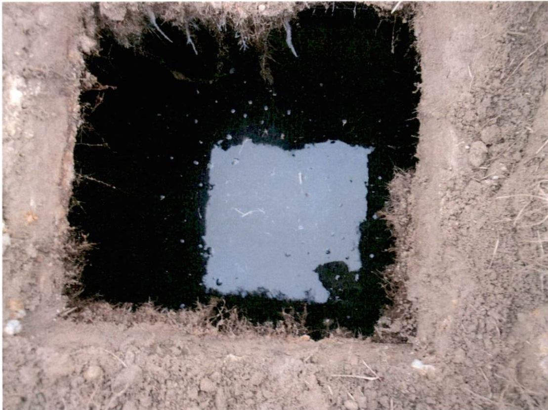
Inlet Access Point of the Septic Tank
