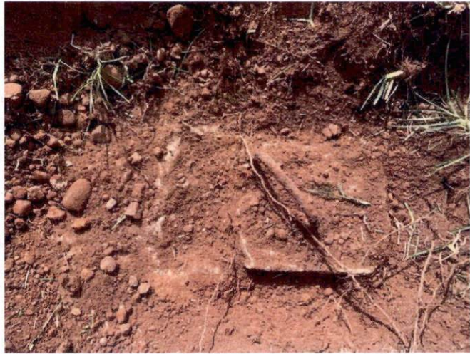
Outlet inspection port lid noted as damaged/broken
