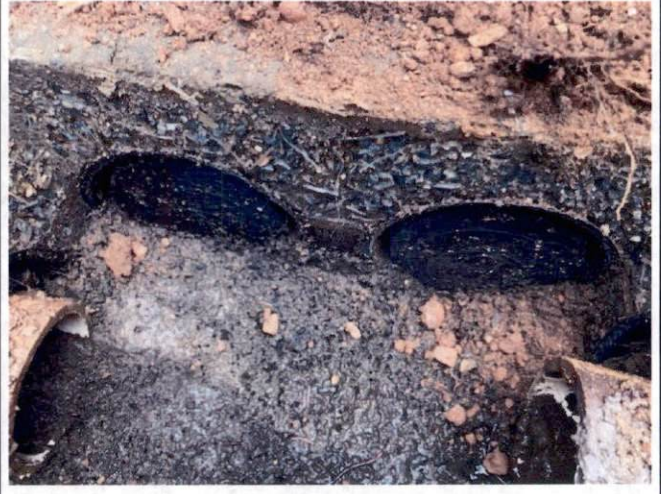
Distribution box shown with minor deterioration
