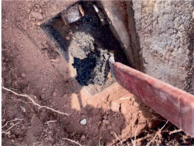
Solids shown collected inside of distribution box
