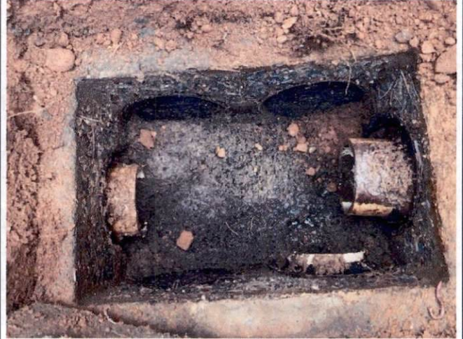
Distribution box shown open for inspection
