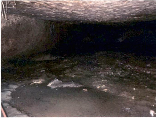
Inlet side of septic tank shown (inlet drain pipe noted as damaged)
