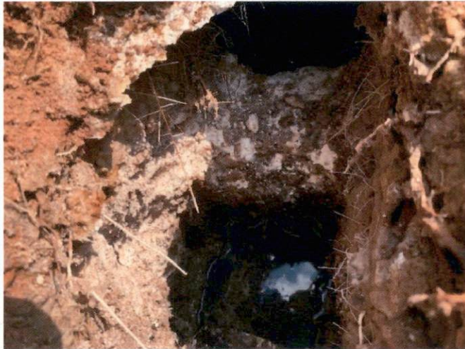
Minor deterioration shown on outlet baffle tee
