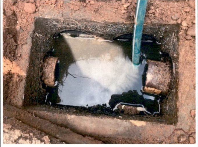
Drain lines noted as not taking water. Dbox flooded
