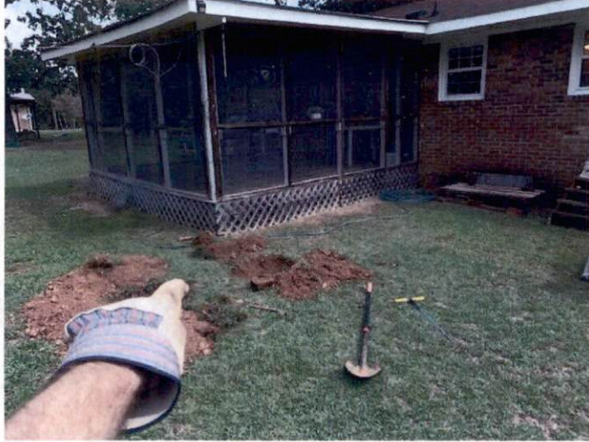
Location of distribution box shown
