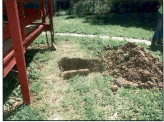
Exposed Access Openings
