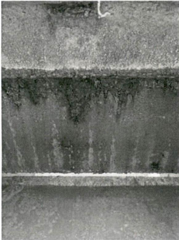
Outlet Side Baffle
