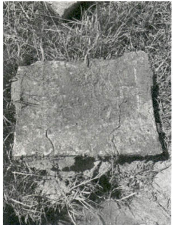
Distribution Box Lid
