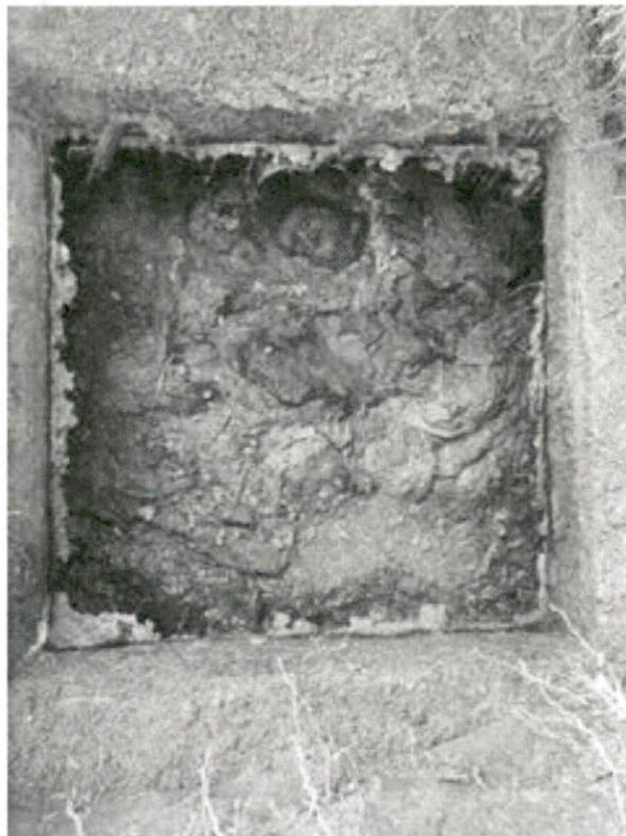
Inlet Side Before Pumping
