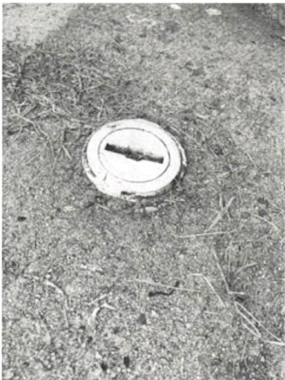
Inlet Sewer Line Cleanout
