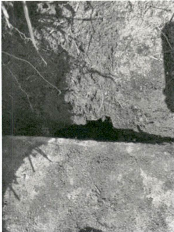
Hole In Tank Beside Outlet Lid
