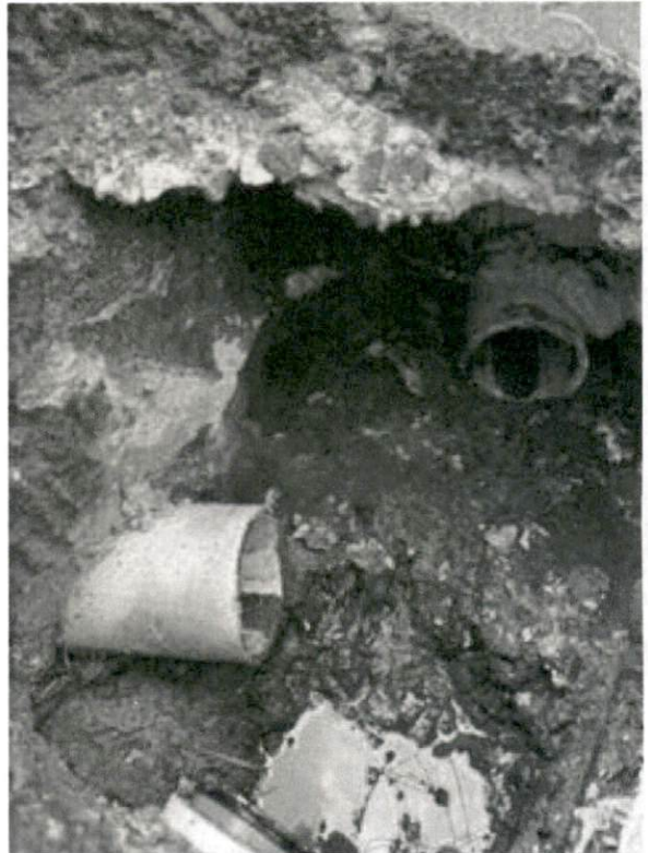
Inside Distribution Box
