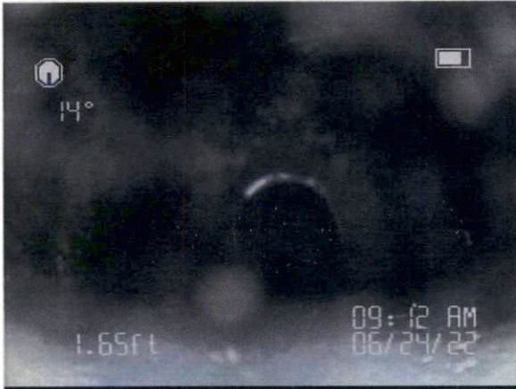
D-Box signs of Deterioration
