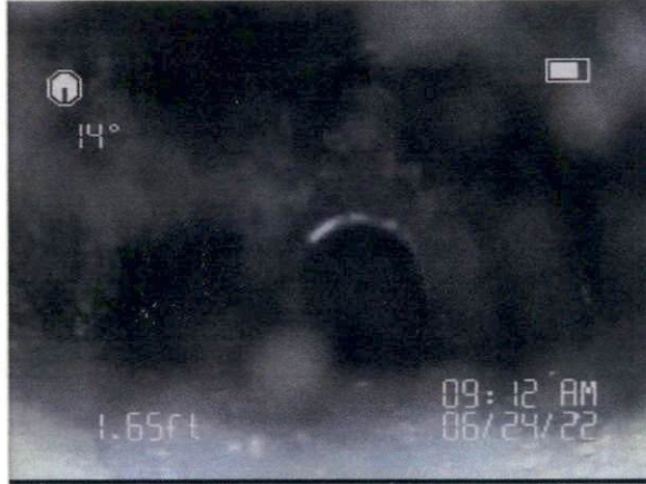
D-Box signs of Deterioration
