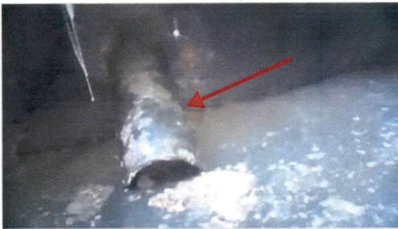
Inlet Pipe slopping downward
