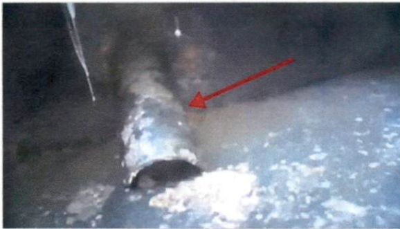
Inlet Pipe slopping downward
