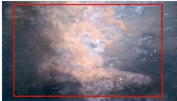
Evidence of early signs of tank deterioration
