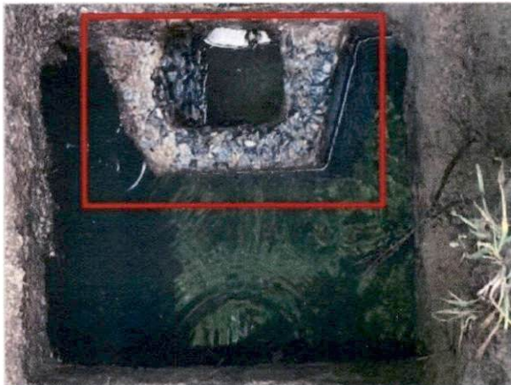
Outlet T heavy signs of deterioration
