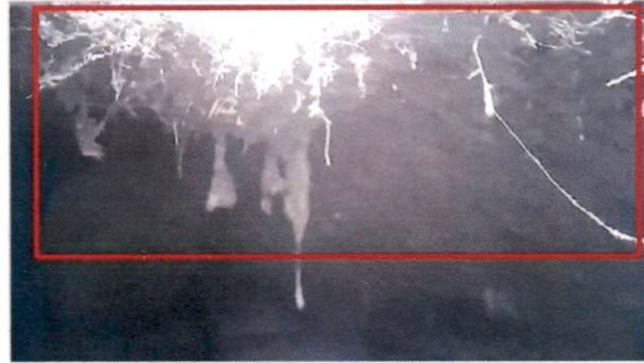
Roots in septic tank
