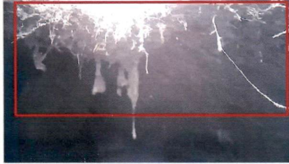
Roots in septic tank
