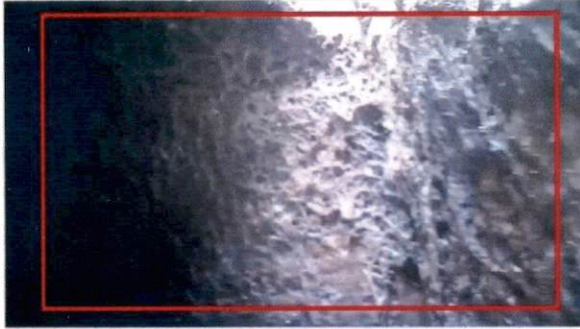
Roots in septic tank
