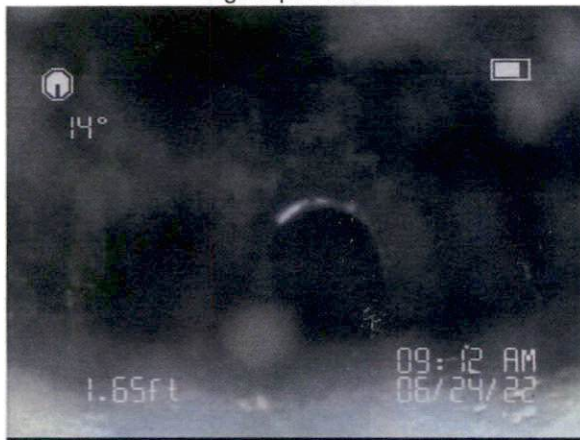
D-Box signs of Deterioration
