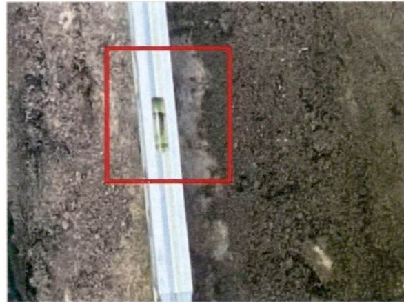
Level on the tank shows pitched back towards structure
