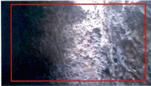
Roots in septic tank
