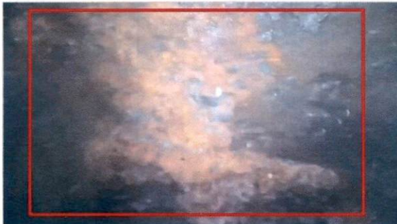
Evidence of early signs of tank deterioration
