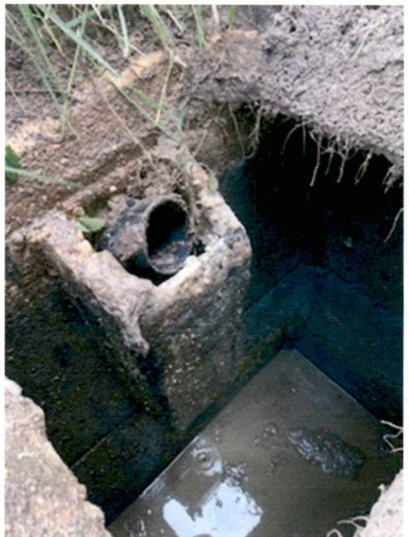
Outlet T and Drain Line
