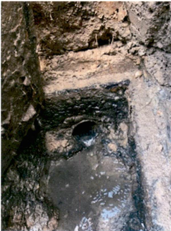
Distribution Box (Deteriorating)
