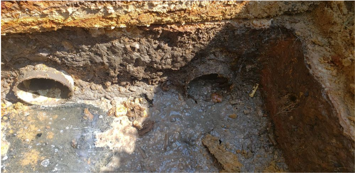
View of Inside of Distribution Box
