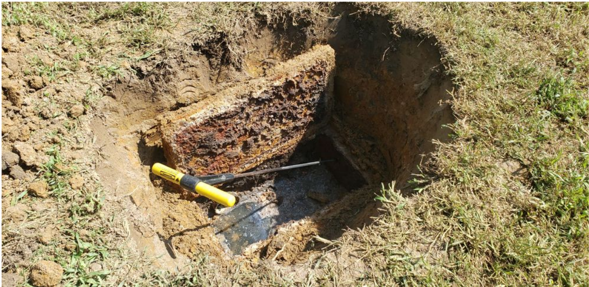
View of Inside of Distribution Box, Probed Through Sidewall
