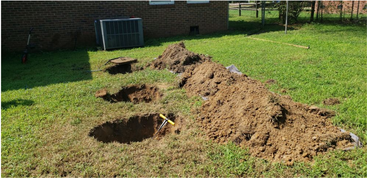
View of Location of Distribution Box
