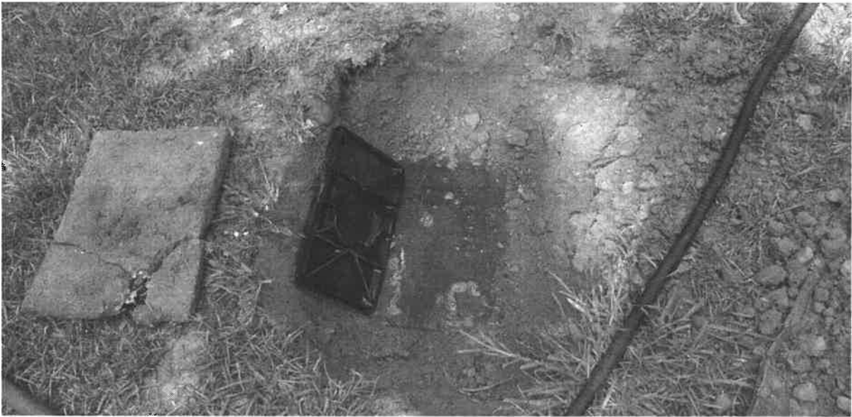
View of High Water Inside the Distribution Box
