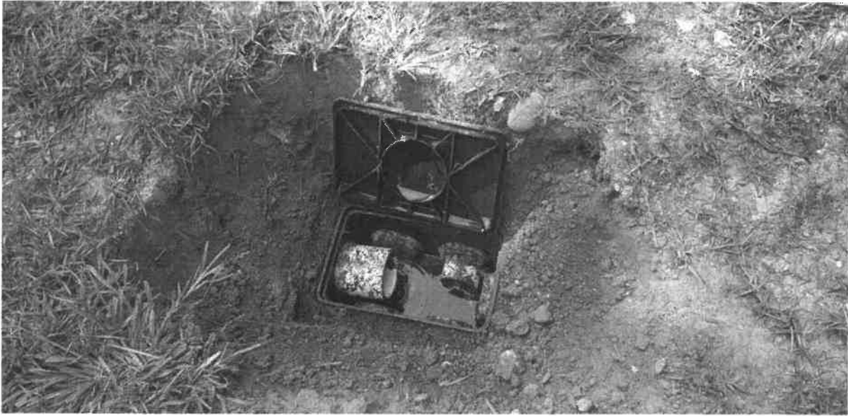
View of Distribution Box
