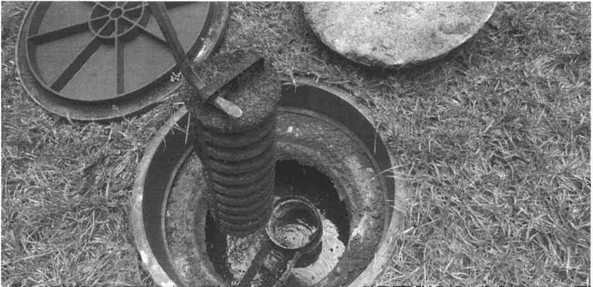
View of Dirty Outlet Tee Filter
