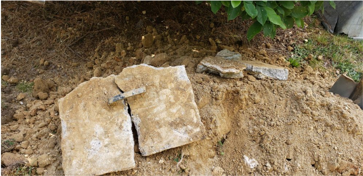
View of Broken Outlet Lid During Removal
