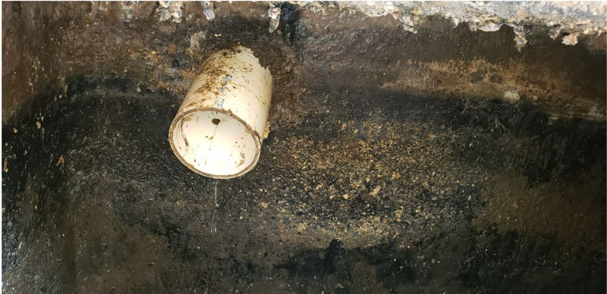
View of Inlet Pipe
