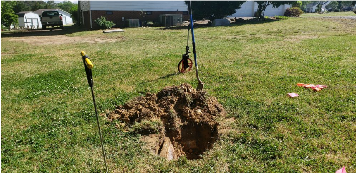
View of Location of Distribution Box
