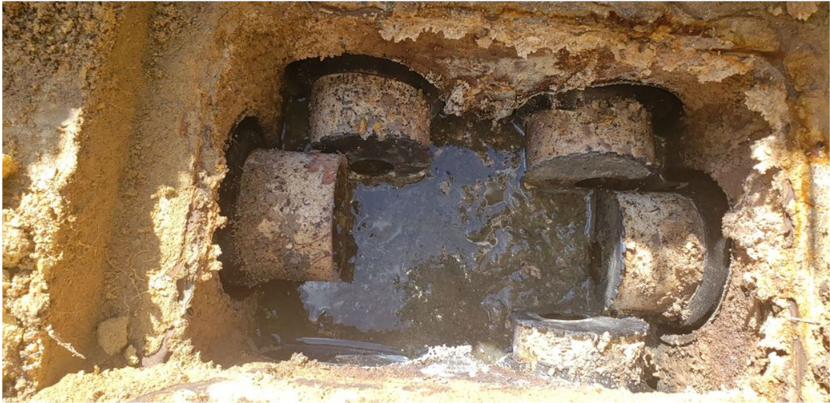
View of Inside of Distribution Box, Not Flowing Equally to All Outlets
