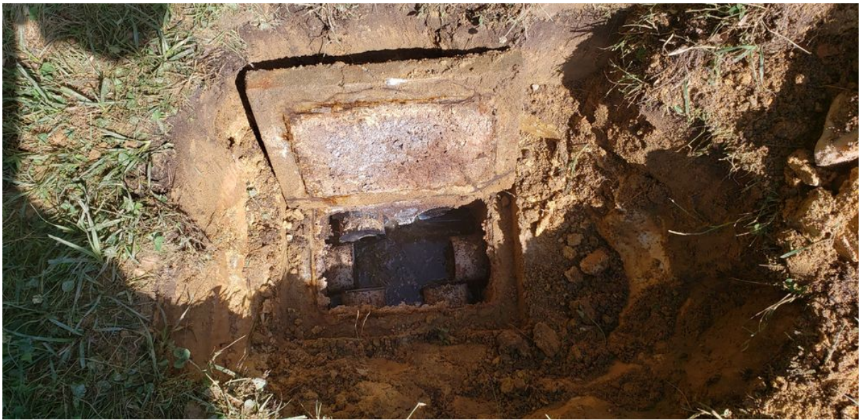
View of Inside of Distribution Box
