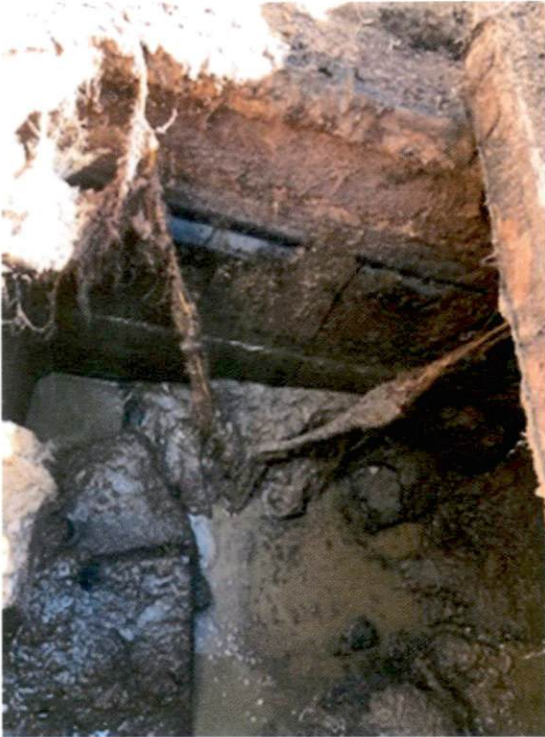
Roots in Septic Tank Along with Part of the Original Top/Lid
