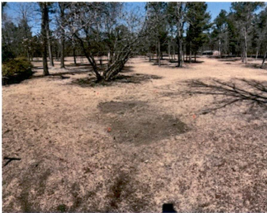
Overall View of Septic System Once Covered and Vegetation Over the Drain Field.
