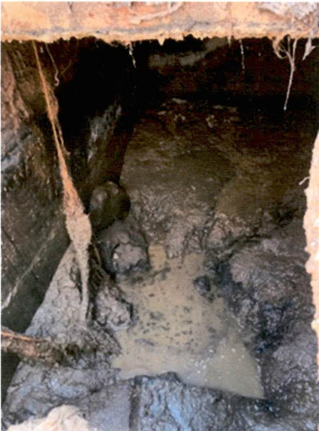
Inside of Septic Tank. (Tank Has No Baffle Wall and Sand Has Partially Filled the Tank)
