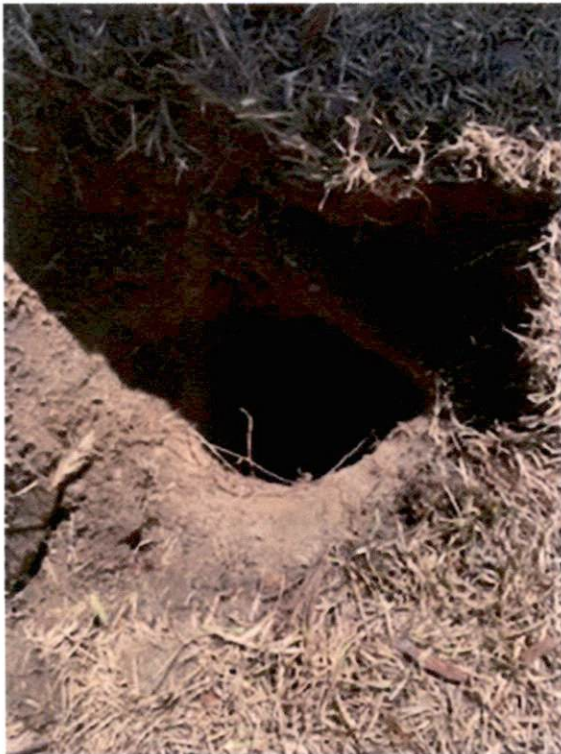
Distribution Box Deterioration. (The roots in the ground were holding the dirt from falling in)
