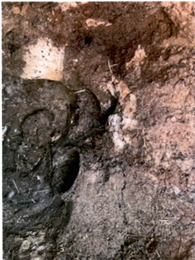
View of the Hole in the Side of the Distribution Box
