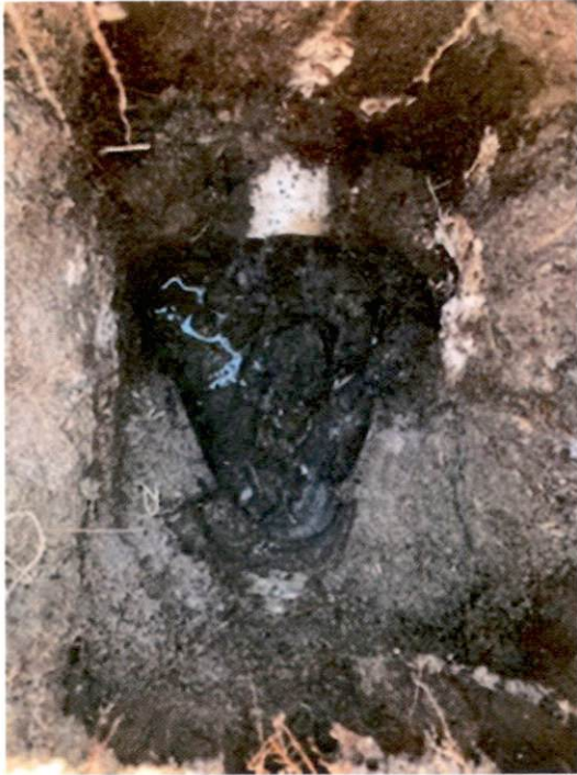
Distribution Box Uncovered. (Roots and some soil in the box. Side of the distribution box also has a hole in it from deterioration)
