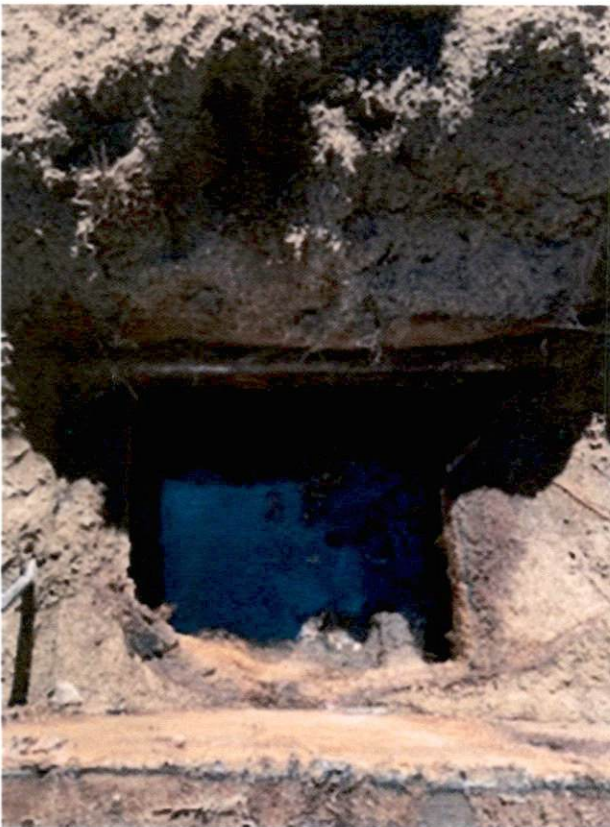
Drain Side of Septic Tank. (Original Top/Lid Has Fallen in the Tank)
