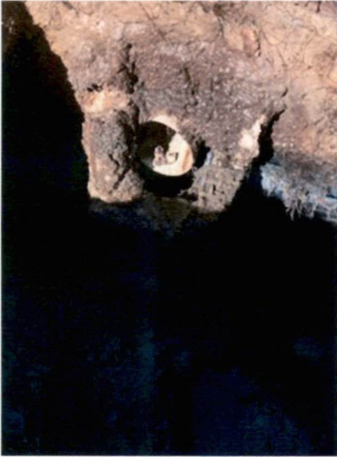
Outlet T Deterioration
