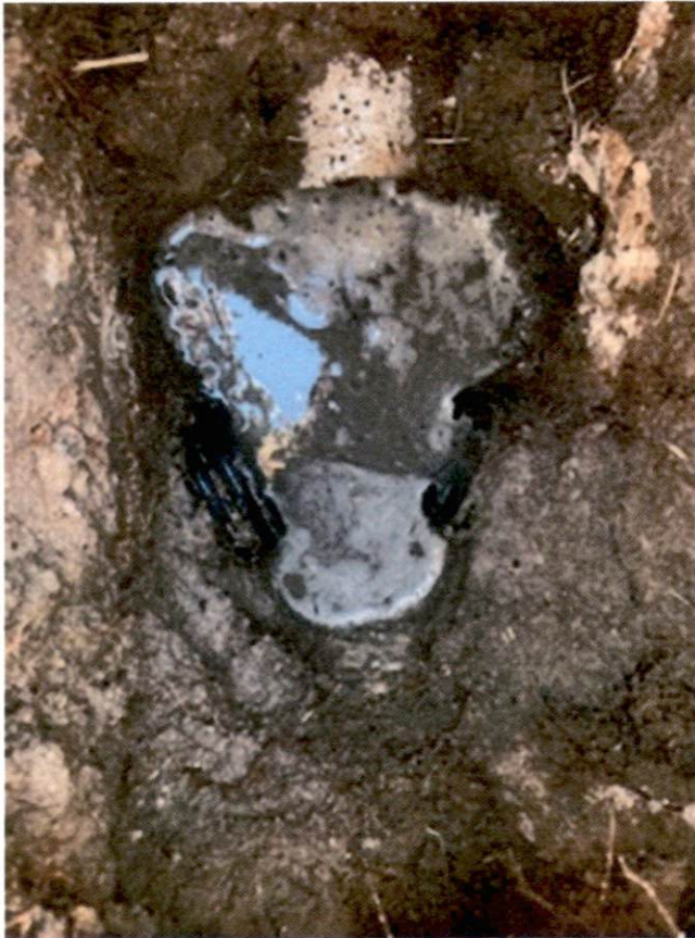
Water Added to Distribution Box. (Drain Lines Not Accepting the Water)
