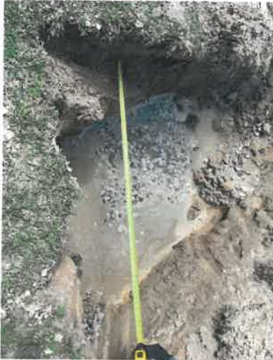
LINES TOO CLOSE
