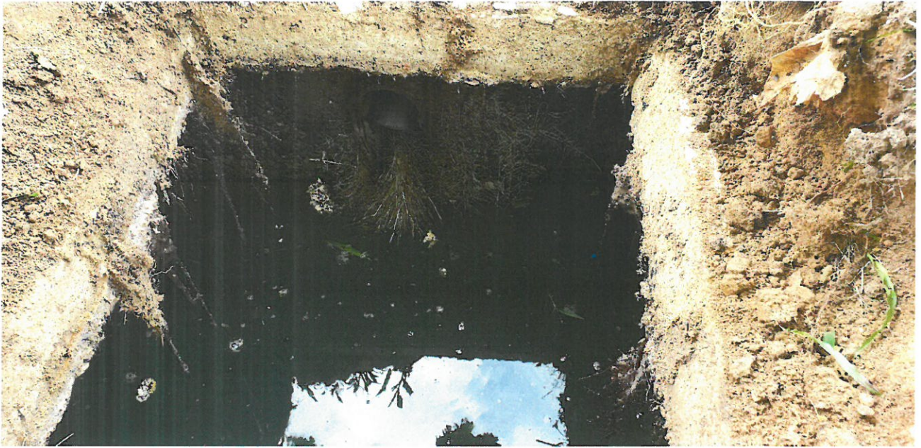
View of Root Intrusion at Inlet Pipe
