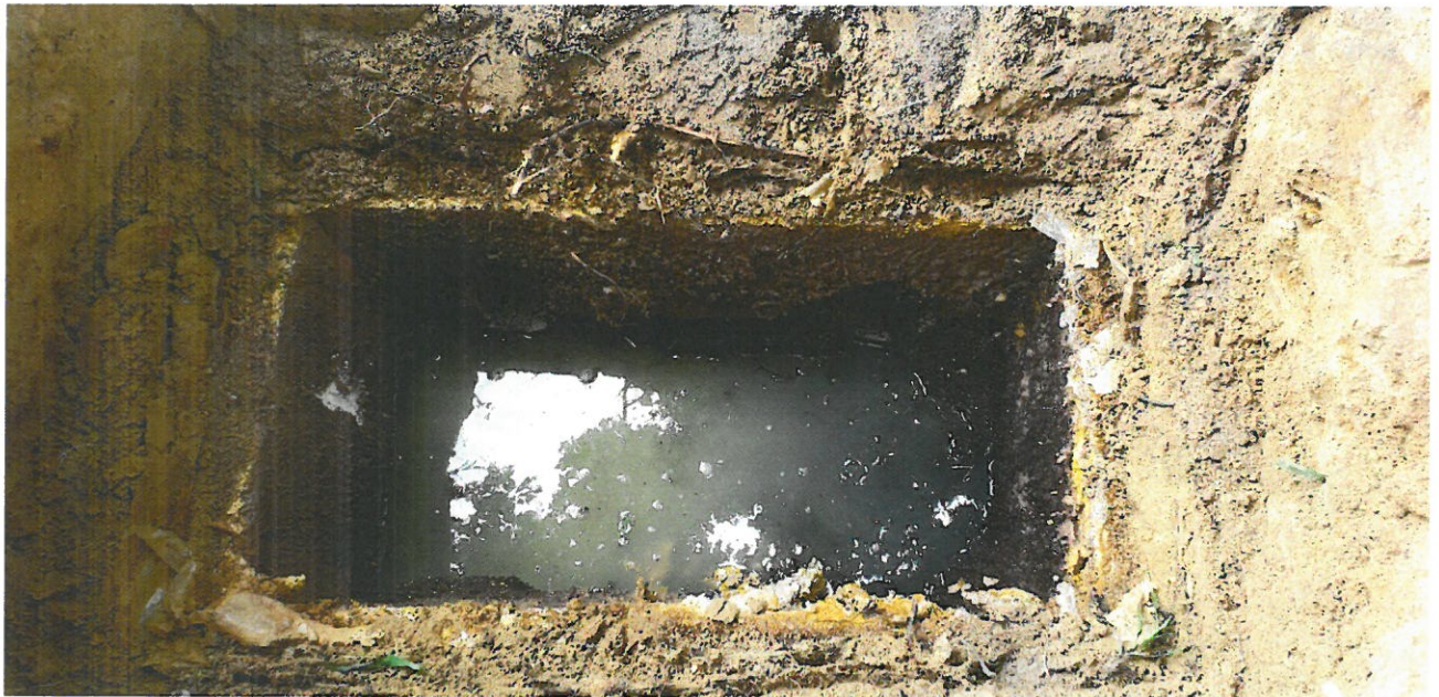
View of Root Intrusion in Distribution Box
