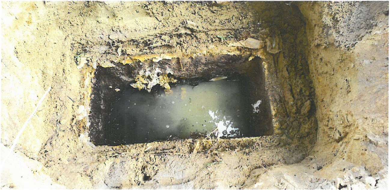
View of Inside of Distribution Box, Deterioration Along Sidewalls
