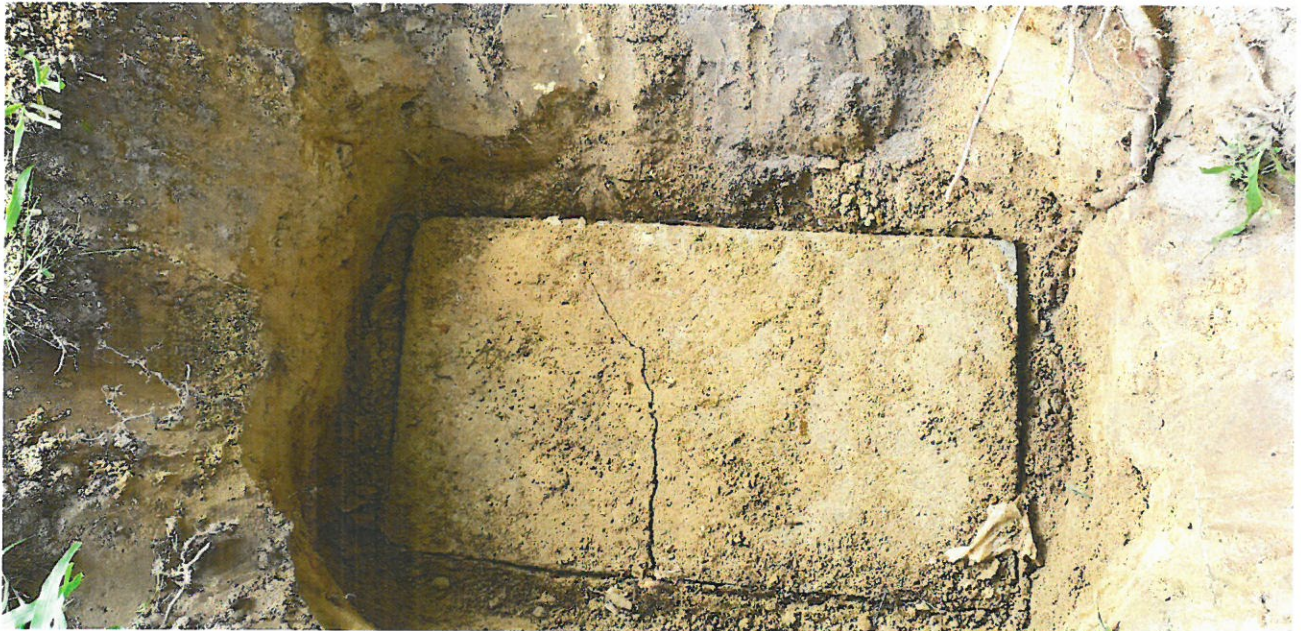
View of Cracked Distribution Box Lid
