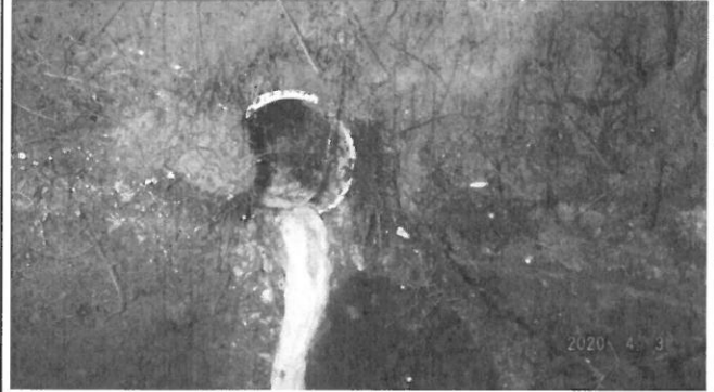
Inlet drainpipe shown not fully extending into the septic tank and roots shown at inlet pipe penetration
