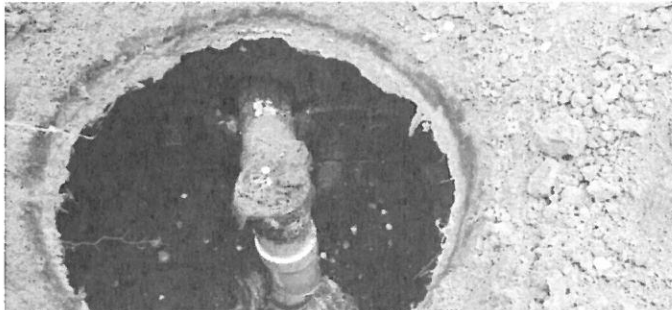
LOW WATER LEVEL IN TANK AND VOIDS AROUND PIPE
